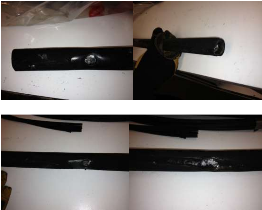
Figure 12: Recent failures on DMA13 & MTN12 feeders
