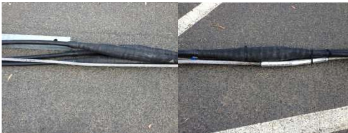
Figure 13: Old Cable joints in replaced section of cable
