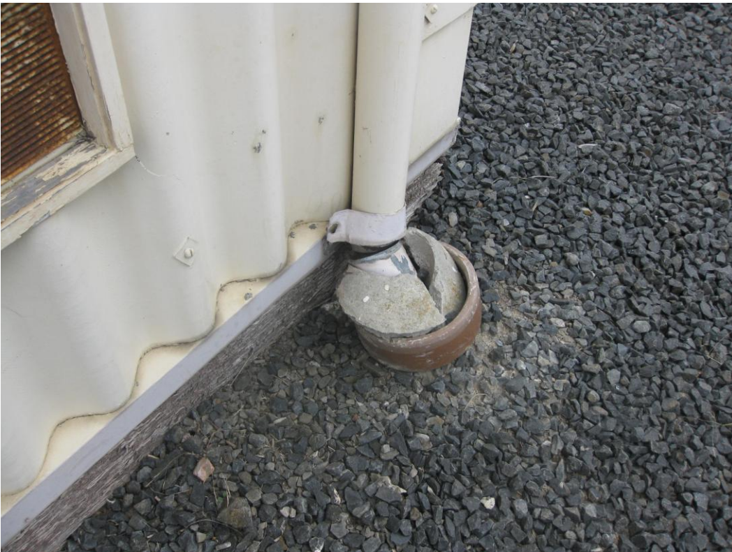
Photo No.4 – Control Room Building – Broken downpipe outlet.
