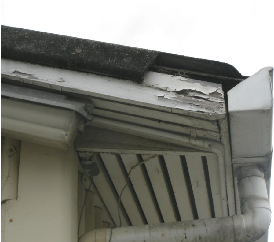
Photo No.2 - Control Room – Asbestos roof gable flashing broken.
