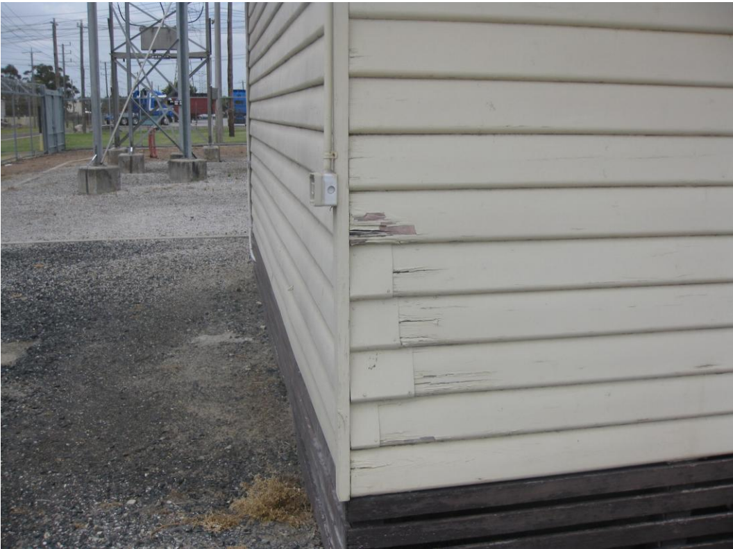
Photo No.5- Control Room – N-E corner weatherboards rotting.
