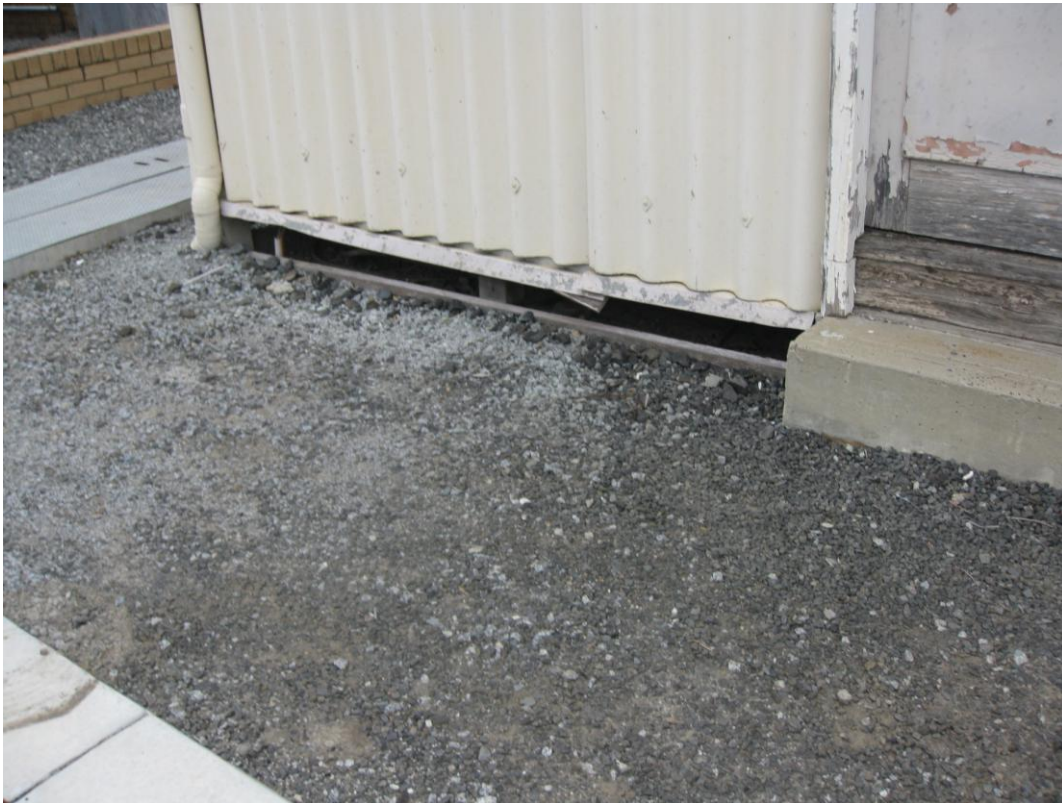
Photo No.8 – Control Room Building – Missing Base Board at N-E corner.
