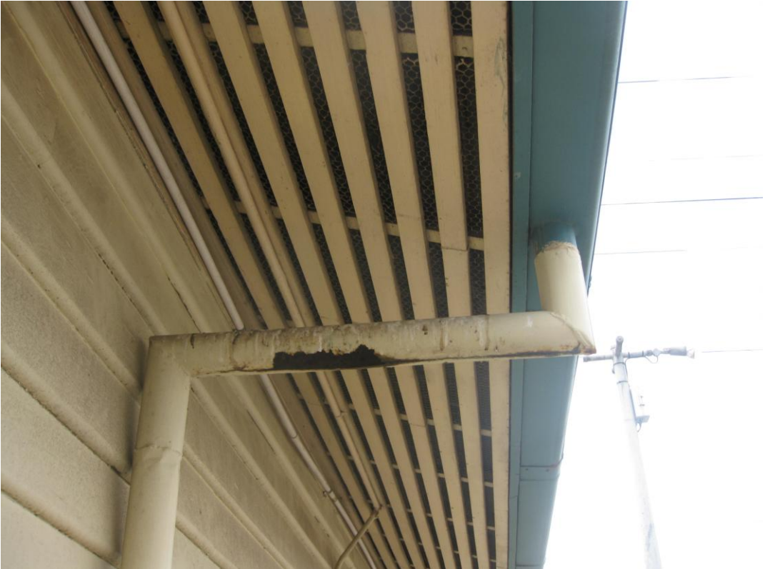
Photo No.2 – Control Room – Corroded downpipe.
