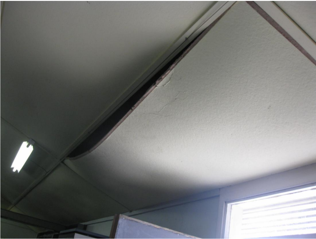
Photo No.3 – Control Room - ‘Canite’ ceiling panel sagged and distorted.
