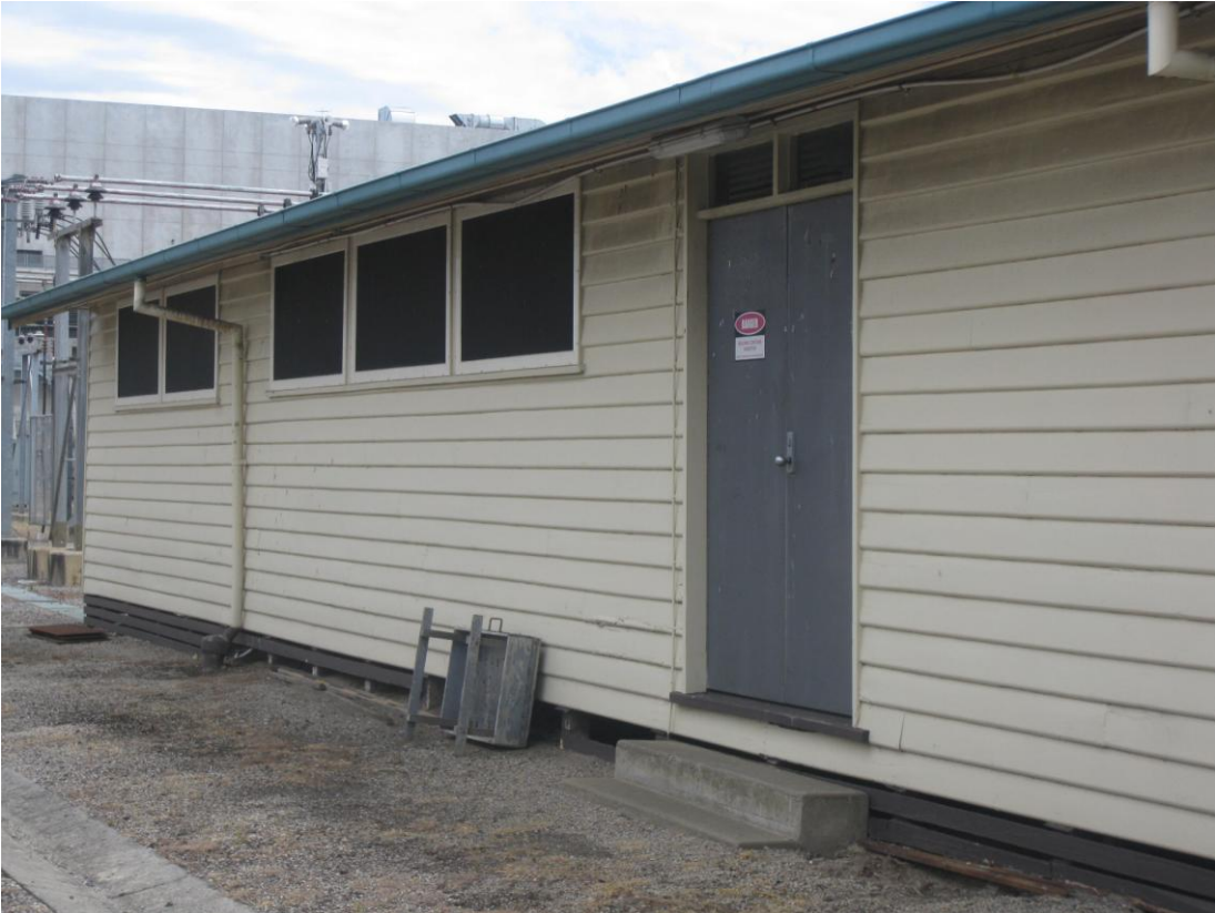
Photo No.6 – Missing base boards.
