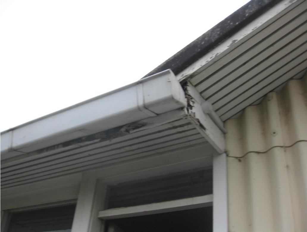
Photo No.3 – Control Room Building – Rotting timber fascia..
