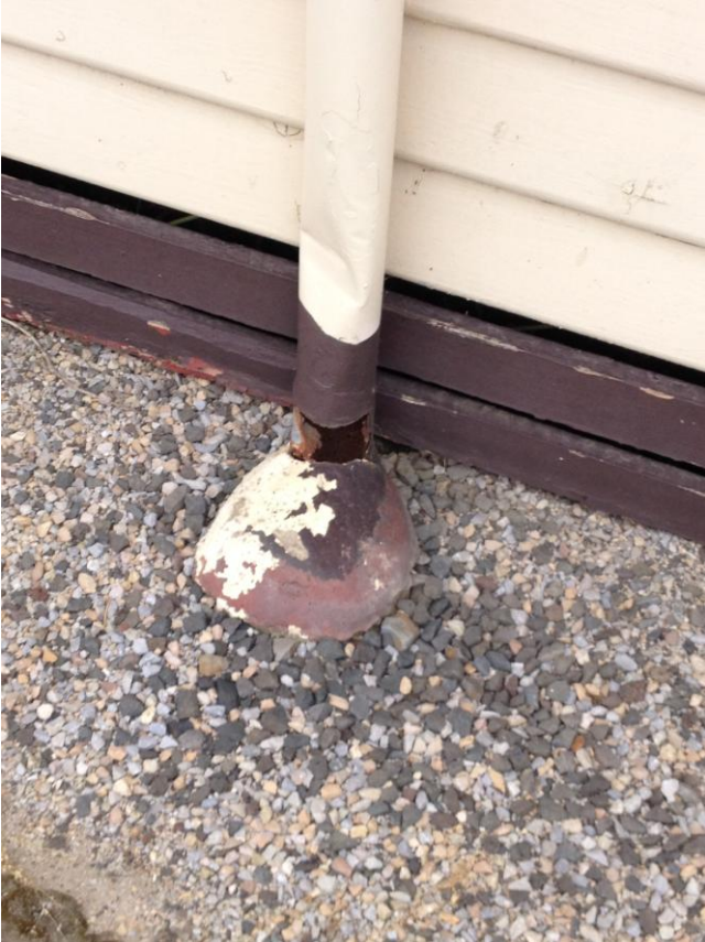
Photo No.8 – Control Room – Corroded Down Pipe causing wash away of yard surfacing fines.
