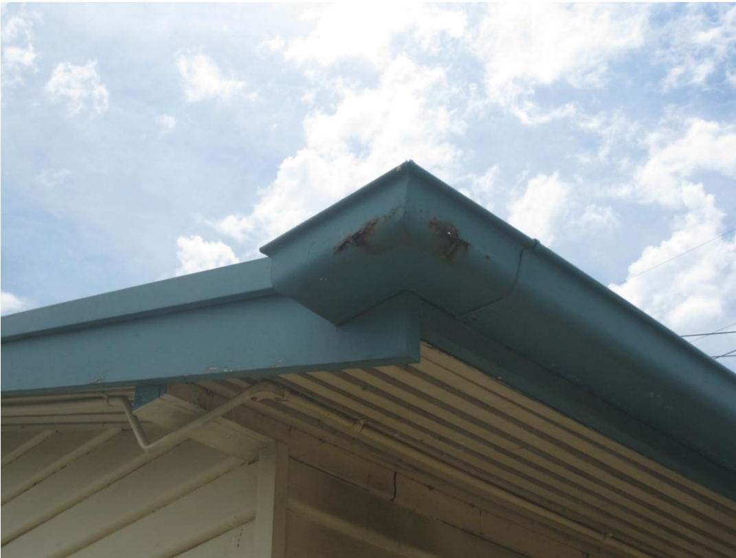
Photo No.1 - Control Room - Corrosion of roof gutter.
