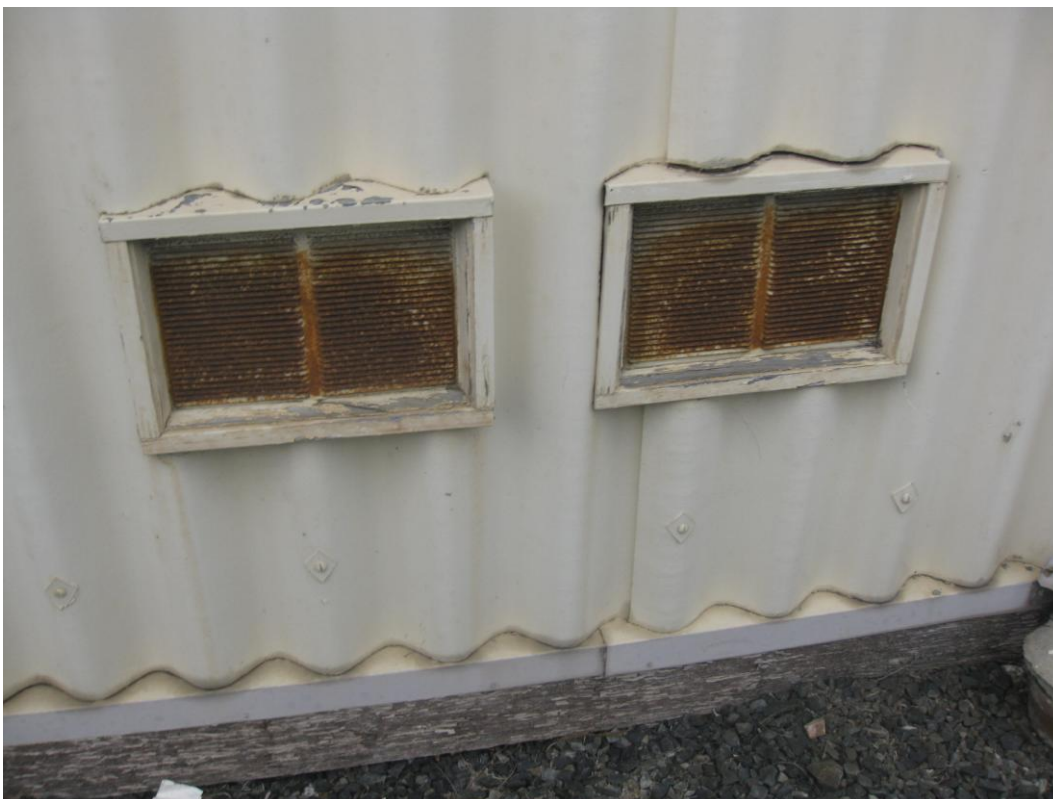
Photo No.6 - Battery Room Vents – Corrosion on external face of metal vents.
