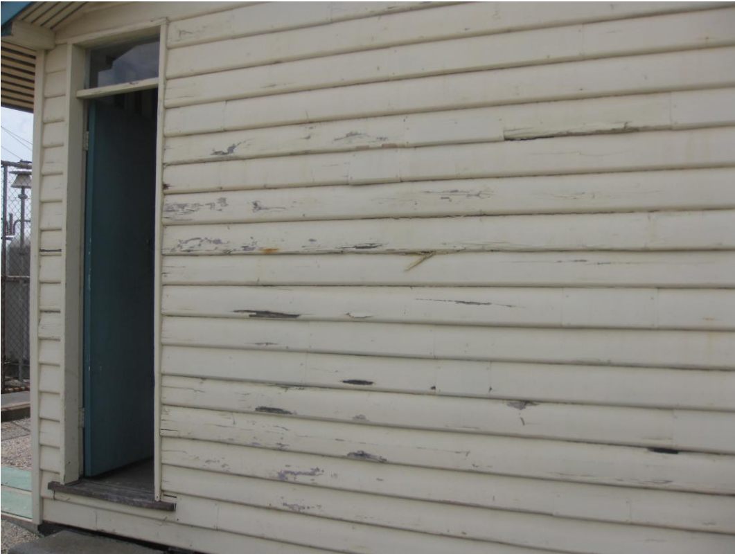
Photo No.4 - Control Room – West wall peeling paint and rot in weatherboards.
