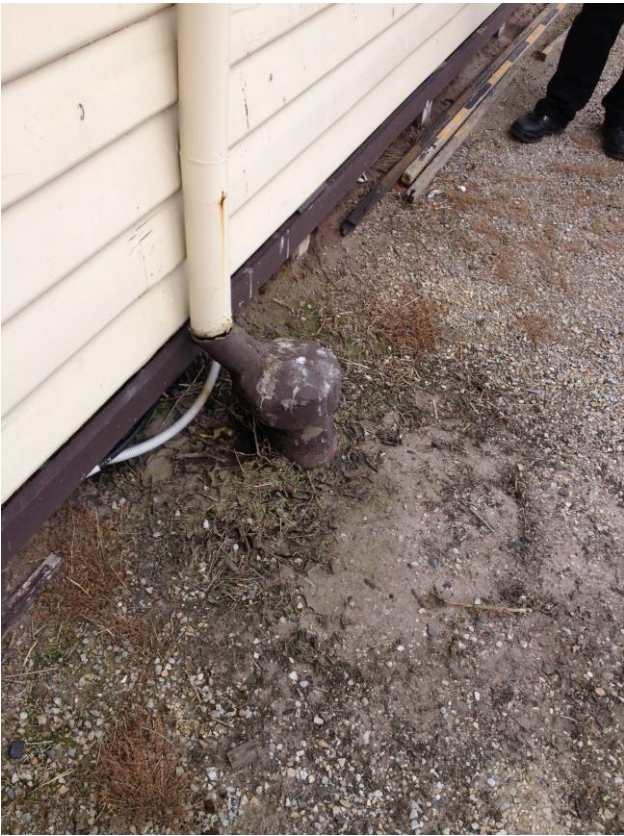
Photo No.7 – Control Room – Leaking Down Pipe causing yard surface wash away.
