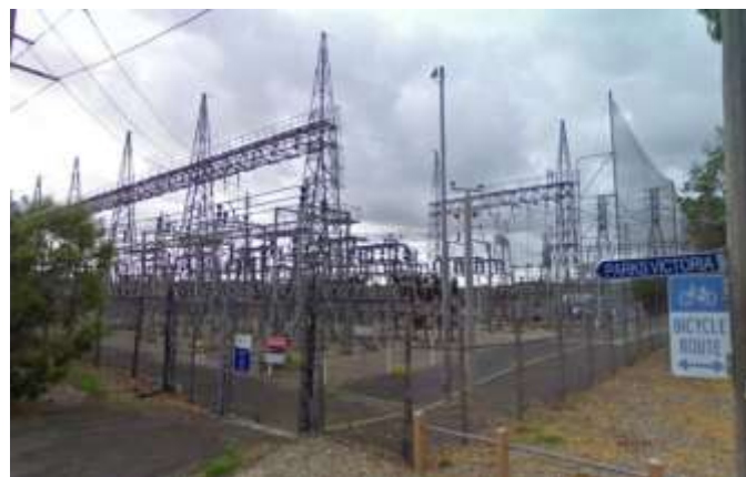
Figure 1: Existing RTS 66kV Switchyard
