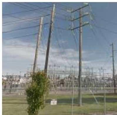
Figure 1: Existing HTS 66kV Switchyard
