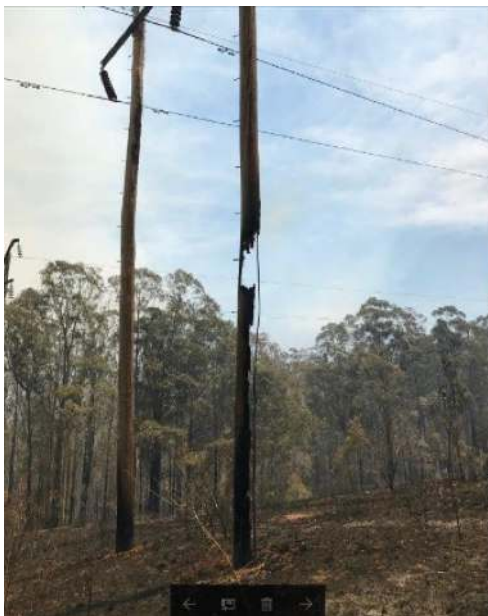
Figure 1: Line 963 Structure 446 Fire Damage
