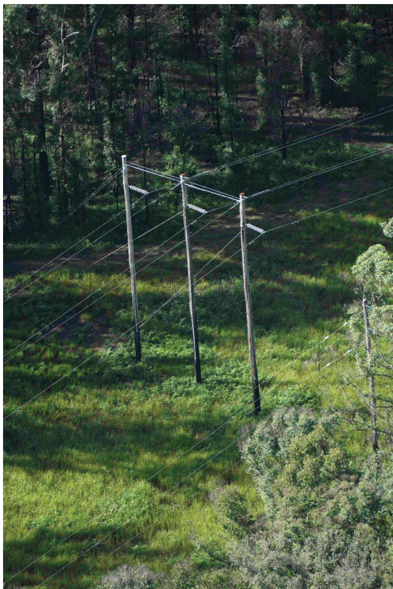
Figure 2: Structure 451 with Fire Damage
