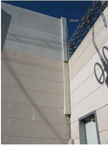
Sydney South No. 6 transformer - entrance to the compound
