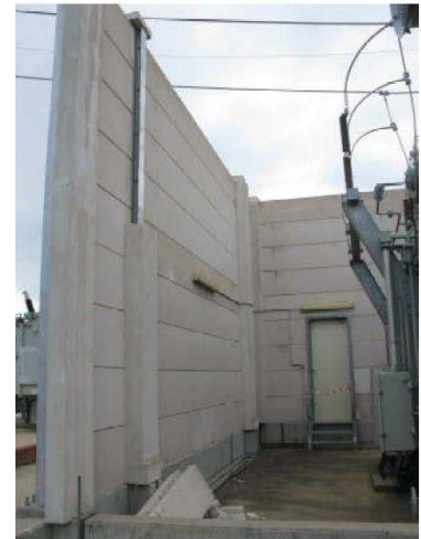
Orange No.1 transformer – fallen brickwork
