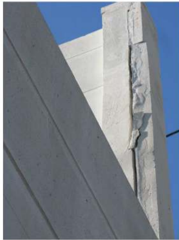
Sydney South No.6 transformer - wall joint cracking
