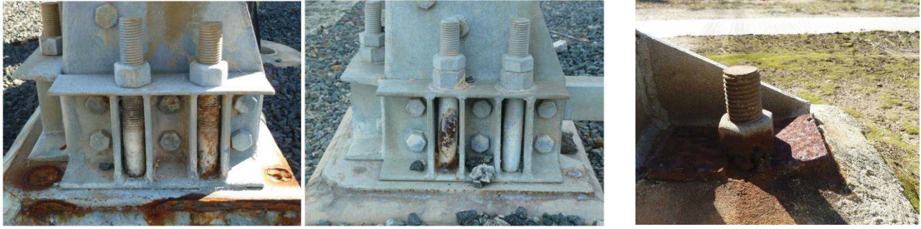
Figure 3: Typical corrosion to holding down bolts and baseplates
