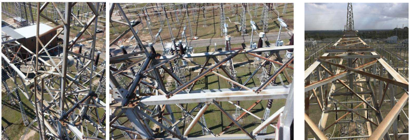
Figure 2: Typical gantry steel members showing corrosion
