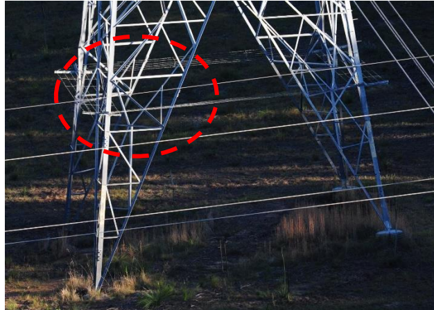
Figure 2 Anti-Climbers without Diagonal Wires and/or Grid Infill
