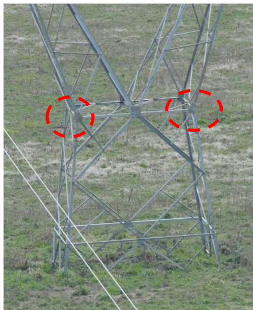
Figure 1 Tower with Spike Type Anti-Climbers
