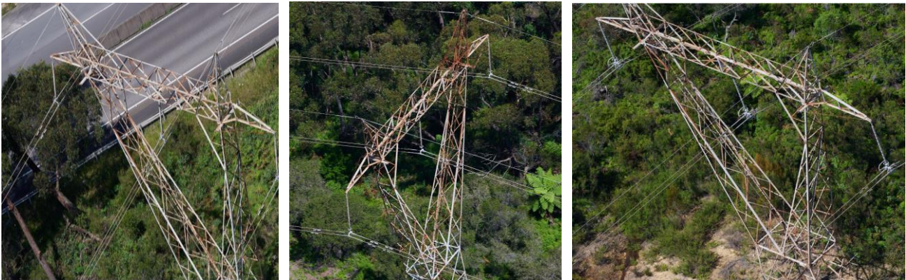
Figure 2 – Photos of Deterioration of structures
