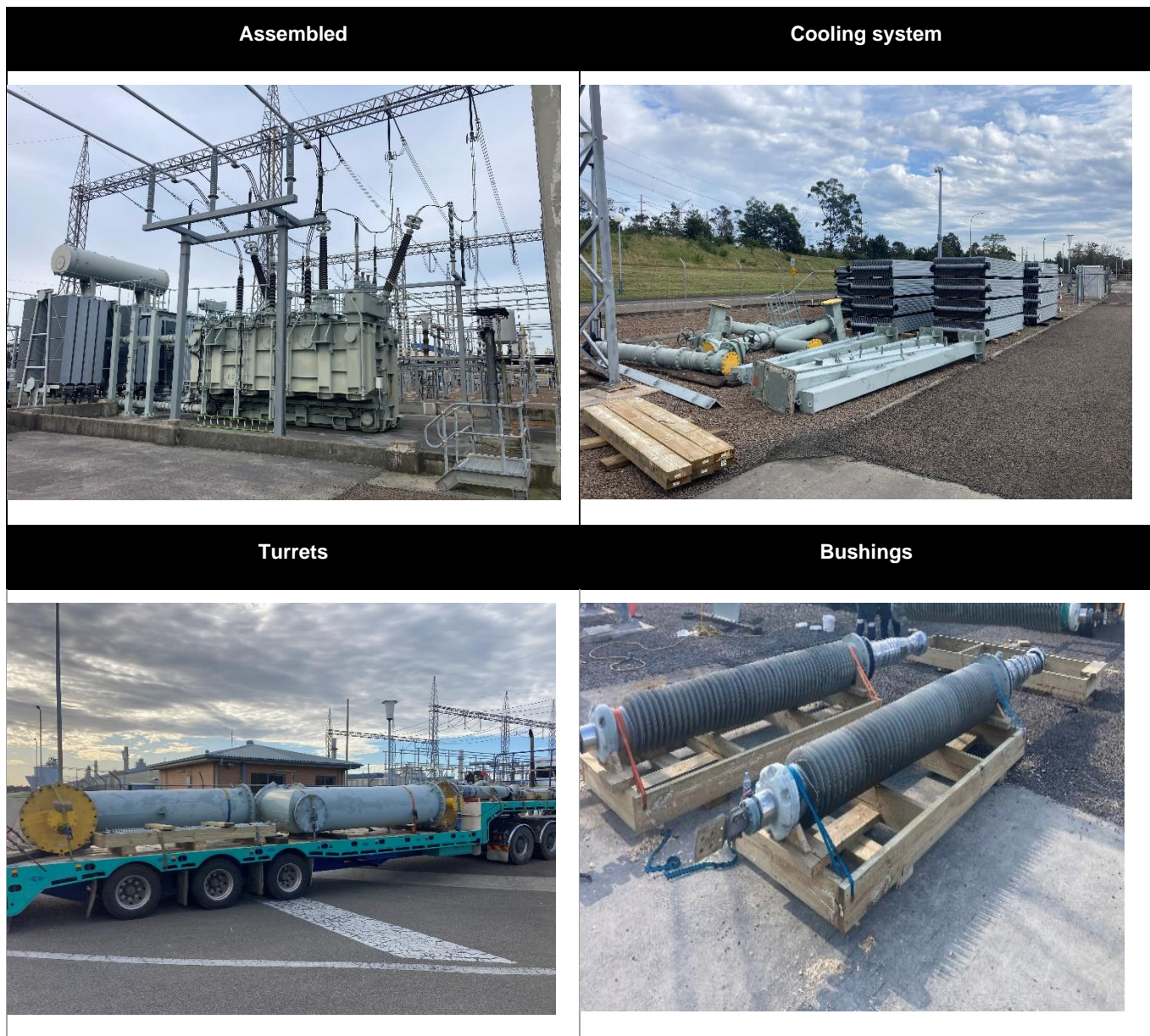
Figure 4 Assembled and disassembled transformers
