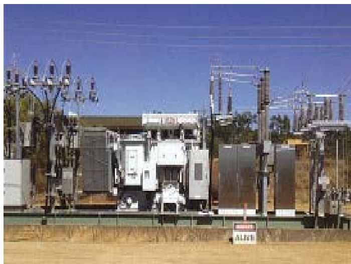
A typical mobile substation installation
