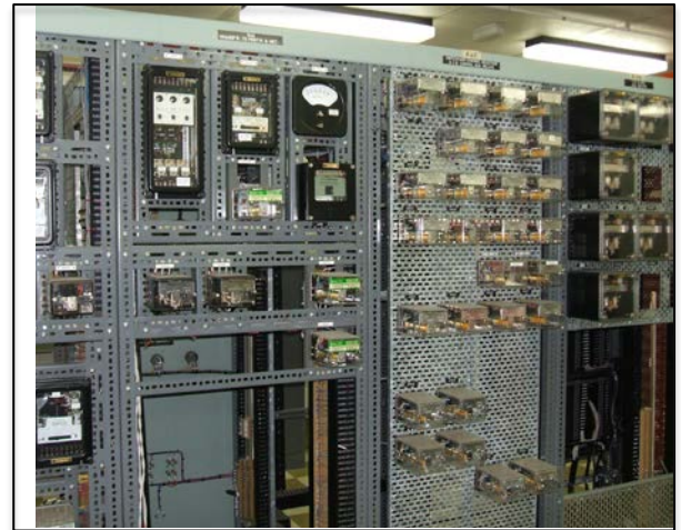
Gordon Substation 220 kV / 22 kV transformer protection
