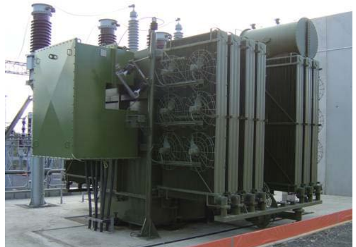
Existing Lindisfarne transformers
