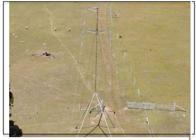
Example of a K-pole structure currently in service
