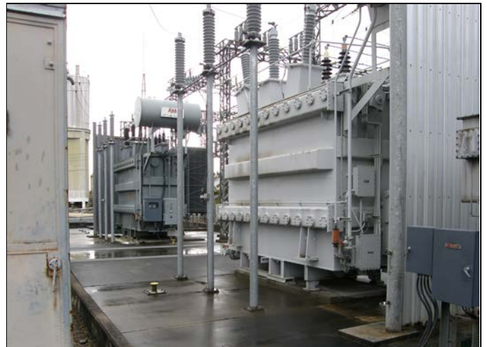
Existing transformers at Rosebery Substation
