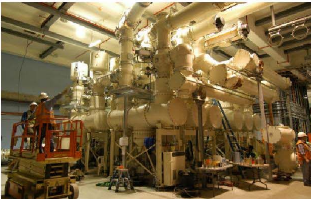
330kV gas insulated switchgear in Haymarket substation, Sydney CBD
