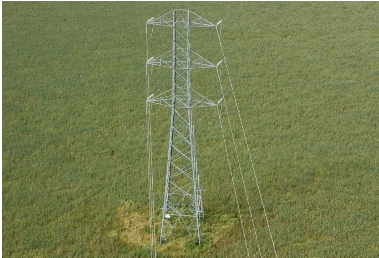
Figure 1: Steel lattice tower (galvanised)
