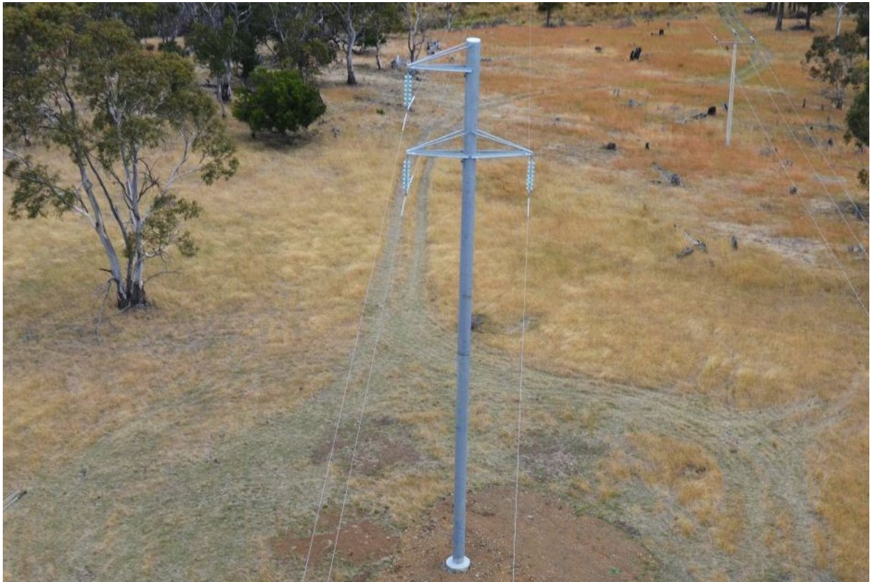
Figure 7: Steel pole structure
