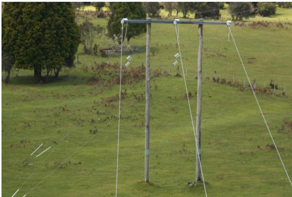
Figure 5: Wood pole structures
