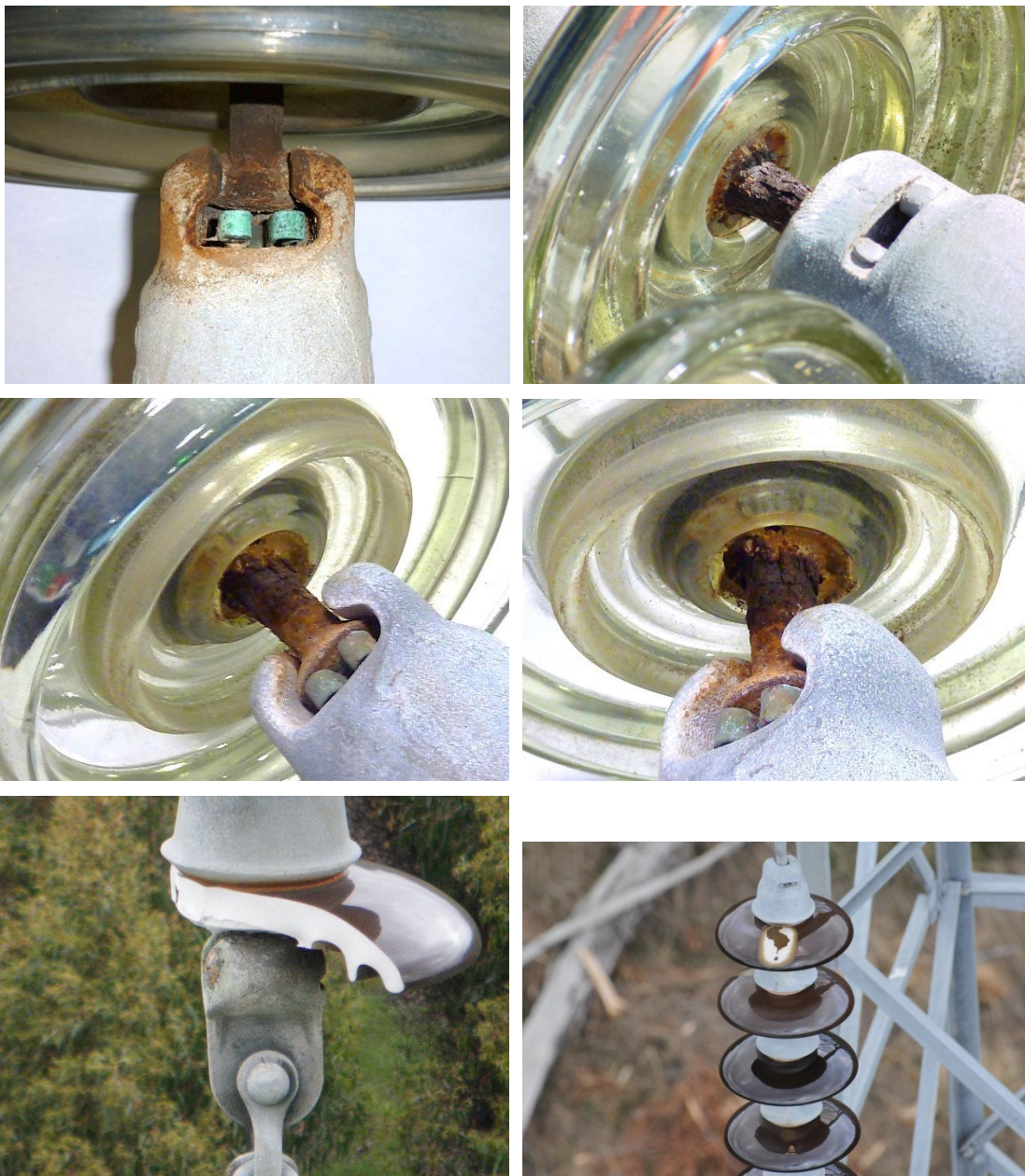
Figure 6 Typical insulator defects
