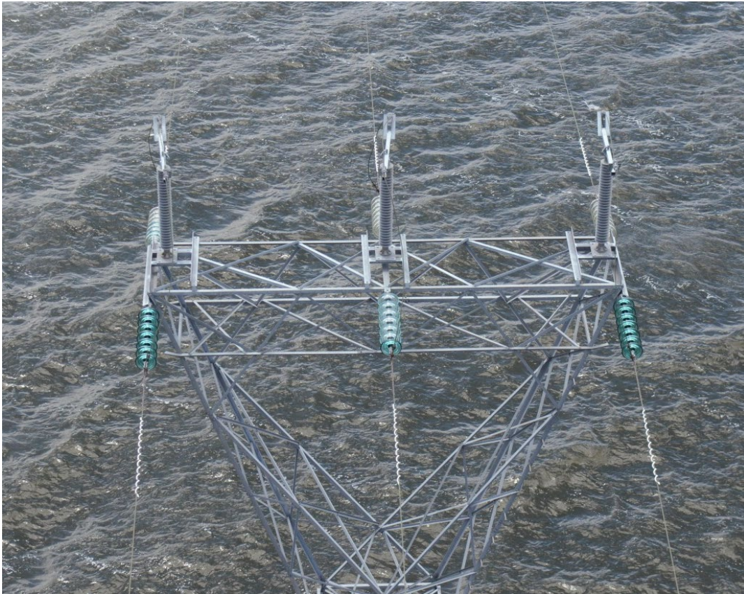
Figure 5 Porcelain post insulators
