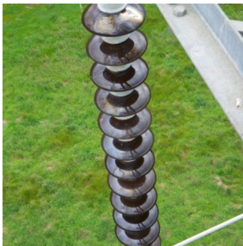
Figure 2 220 kV porcelain disc insulator assembly
