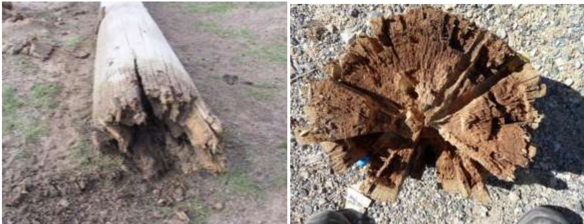
Figure 5 Wood poles that has failed in service from rot
