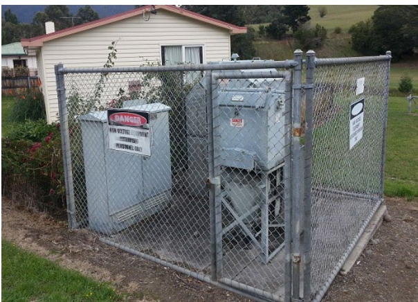
Figure 3 Fence type substation (1967)
