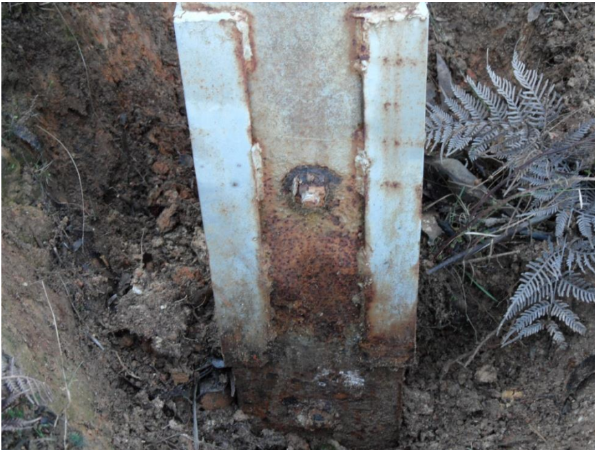
Figure 10: Poor condition steel and concrete (Stobie) pole
