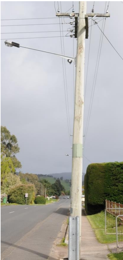
Figure 18: Staked wood pole
