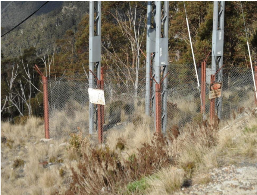
Figure 24: Anti-climbing Barrier with Faded Signage
