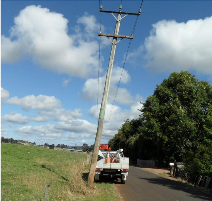
Figure 8: Pole leaning more than 6° (or more than 4 pole tops)
