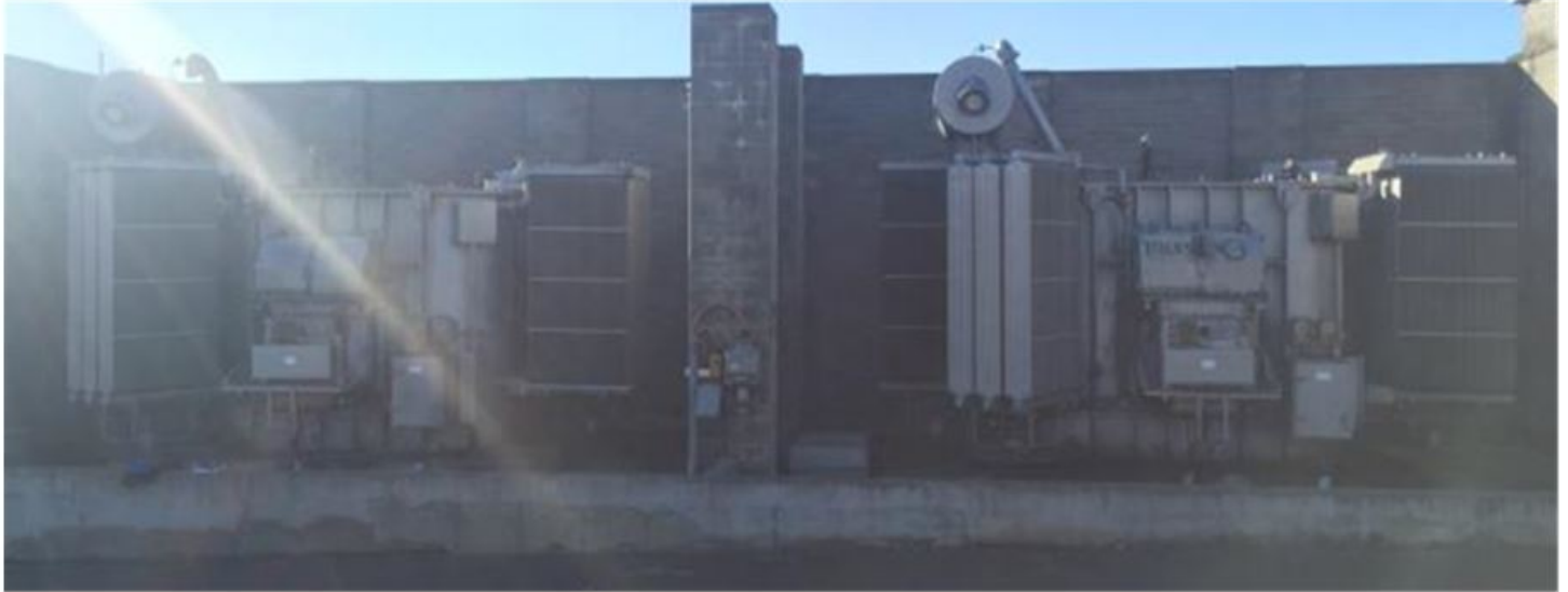
Photo 1 – Claremont Zone transformers
