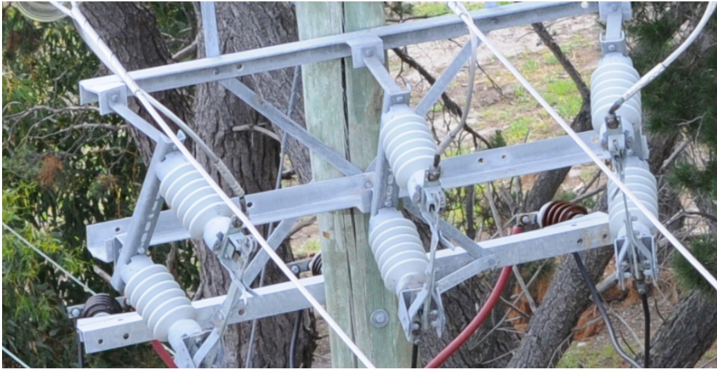
Figure 1 Pole mounted HV Links
