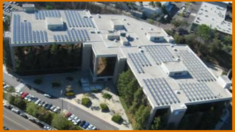
SunEdison's AT&T Installation, USA
