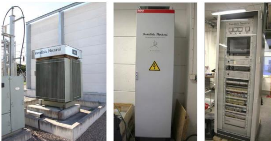
Arc Suppression Coil
