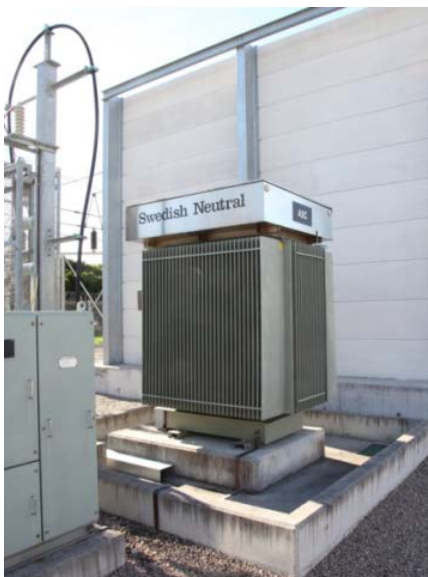
Arc Suppression Coil
