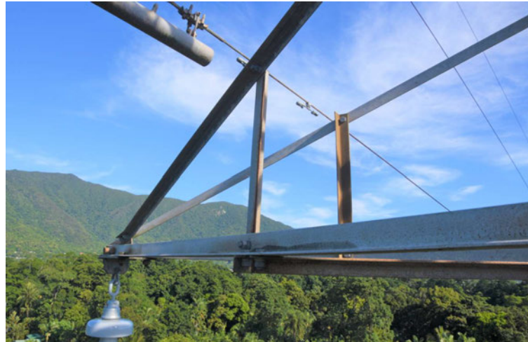
Figure 16: Replaced and original components in the crossarm of suspension tower STR - 1540 (2017)
