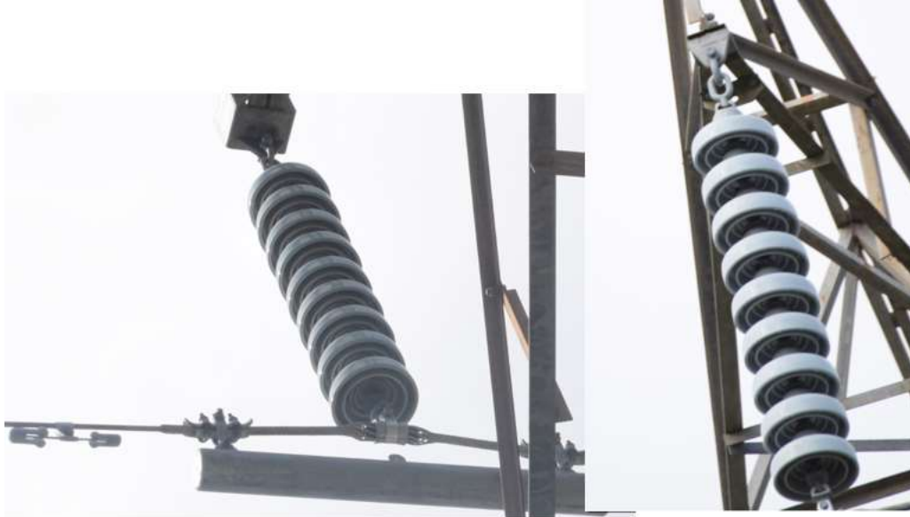
Figure 22: Suspension Insulators in good condition - examples (2019)
