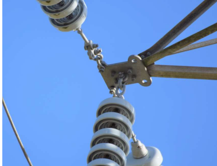
Figure 26: STR-1554 Tension and Bridging Insulator Hardware (2019)
