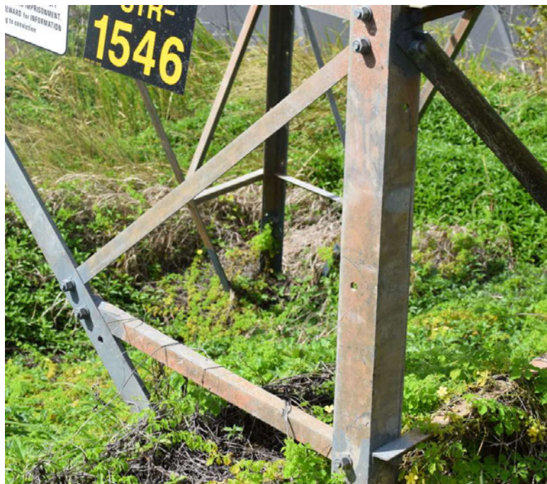
Figure 8: Typical example of corrosion with bolts in better condition than members- example STR - 1546 (2019)
