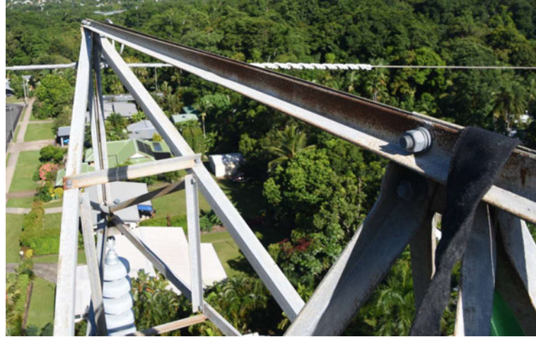
Figure 18: Typical example of corrosion on earthwire peak; STR - 1540 (2017)
