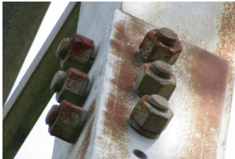
Figure 10: Rare instances of G3 bolt corrosion are more pronounced on tower STR - 1565 (2019)
