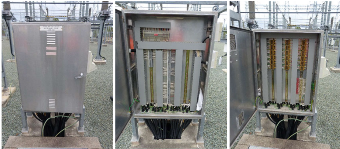
(c) =C05-A30 Bay Marshalling Kiosk
