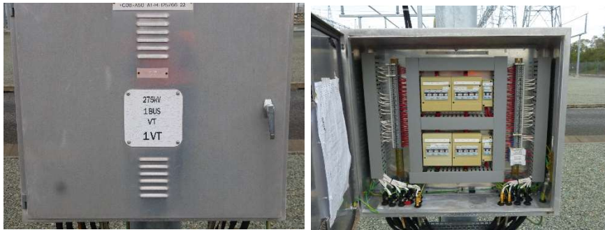
(f) =C08-A50 - 1 Bus VT Marshalling Kiosk
