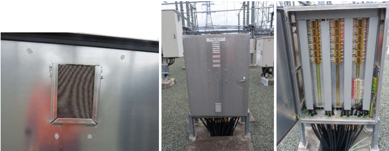
(a) =C04-A10 Bay Marshalling Kiosk
