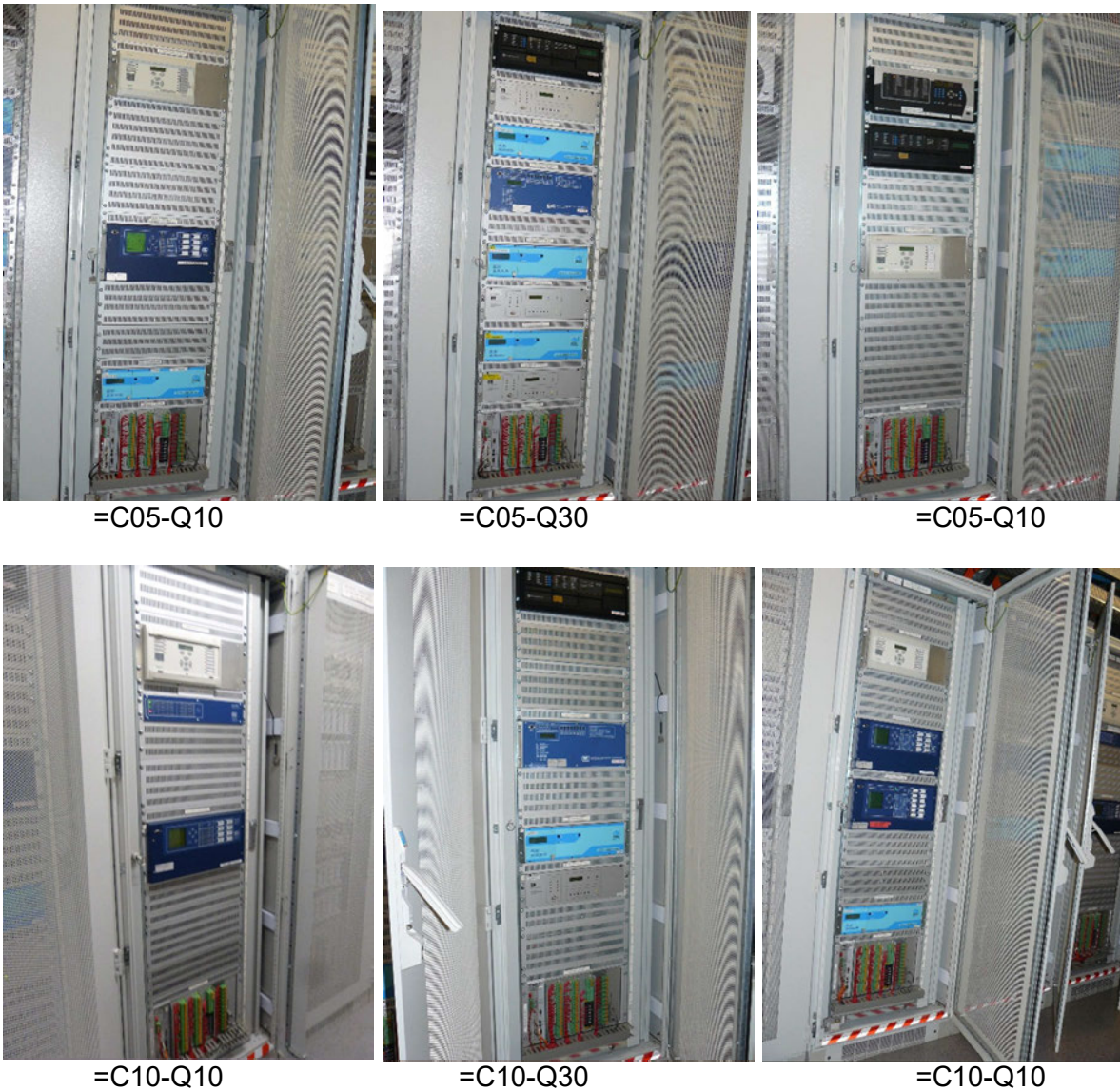
Figure 6 – Typical Indoor Secondary Systems Panels at Greenbank Substation
