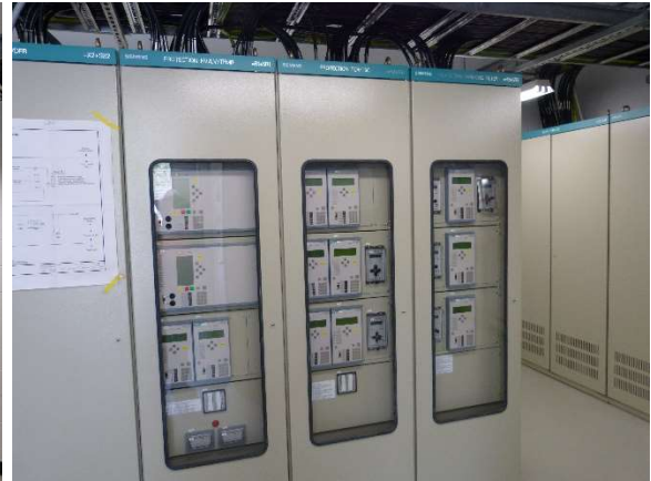
(b) SVC AC Protection Panels
