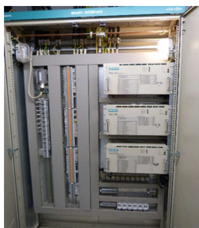
(g) Yard Interface panel
