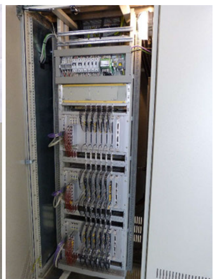
(e) TCR and TSC Valve Base Electronics
