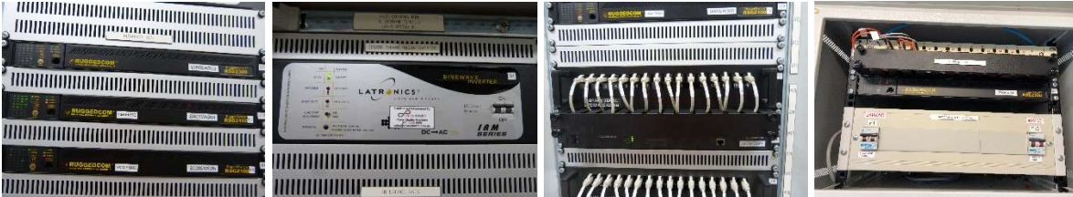
Figure 12 – Greenbank Substation and SVC OpsWAN Equipment
