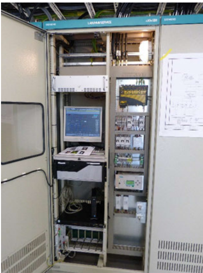
(c) HMI and SCADA Panel
