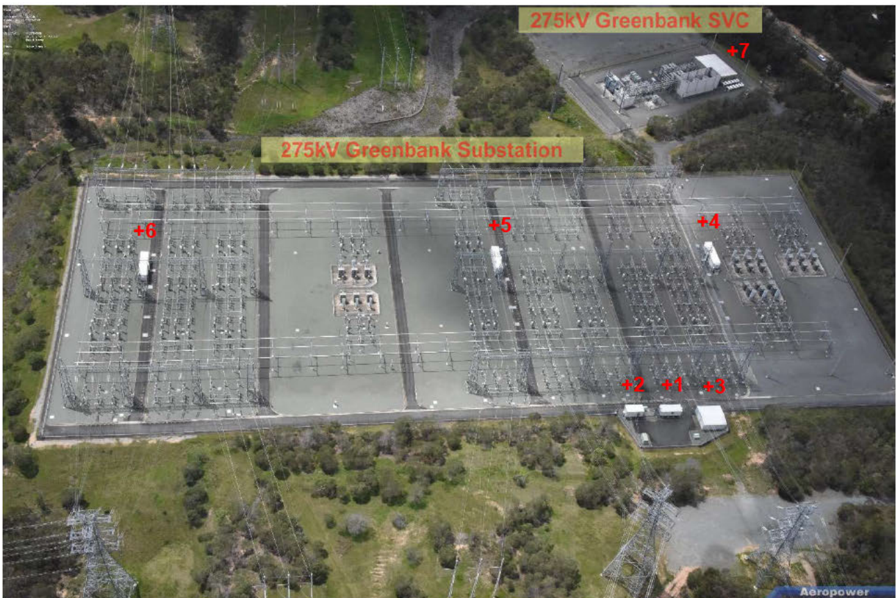
Figure 1 – 275kV Greenbank Substation and SVC and 275kV Substation Aerial View
