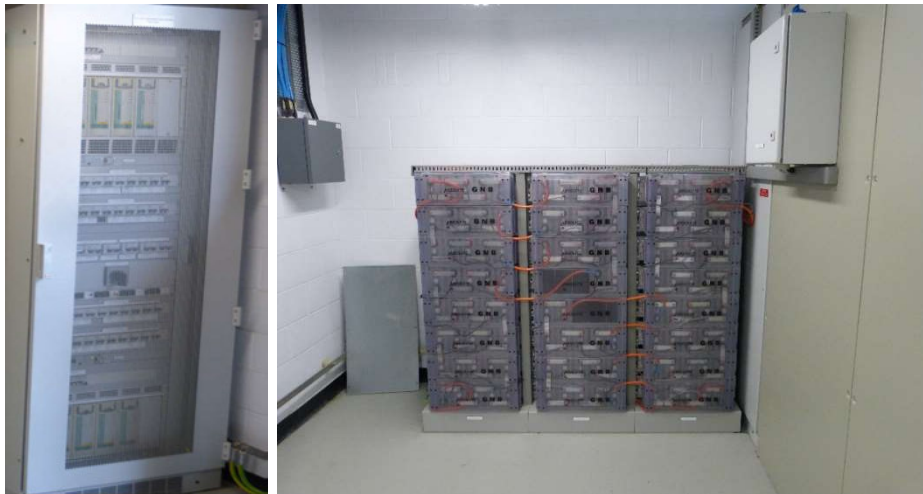
(Buildings +7 - SVC 125V X and Y DC Batteries and Chargers - 2008)
