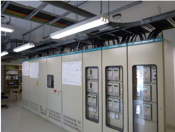
(a) SVC Control and Protection Panels
