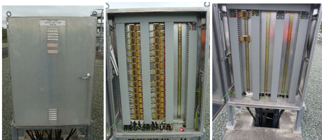
(e) =C08-A2 - 2 Bus CT Marshalling Kiosk
