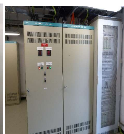
(h) AC Changeover and Battery Charger
