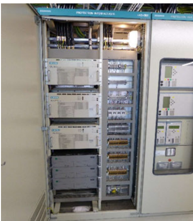
(f) Digital Fault Recorder
