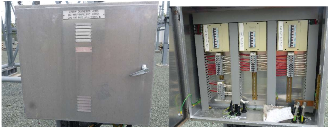
(i) =C06-A92 Diameter =C06 DC Marshalling Kiosk
