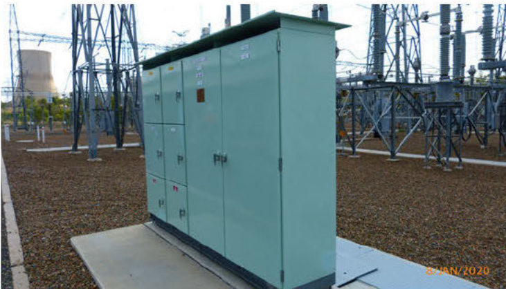
Figure 26: AC changeover board
