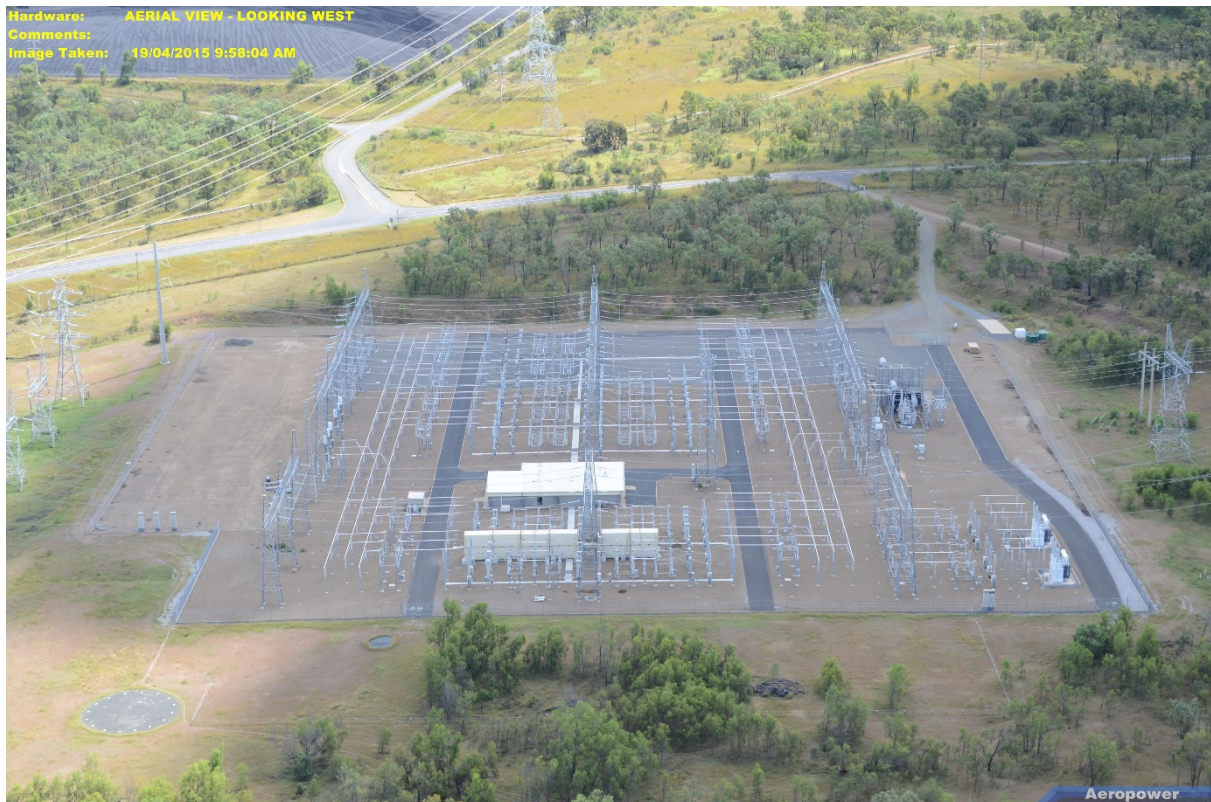
Figure 1 – Aerial Photo of H024 Calvale Substation – 2015
