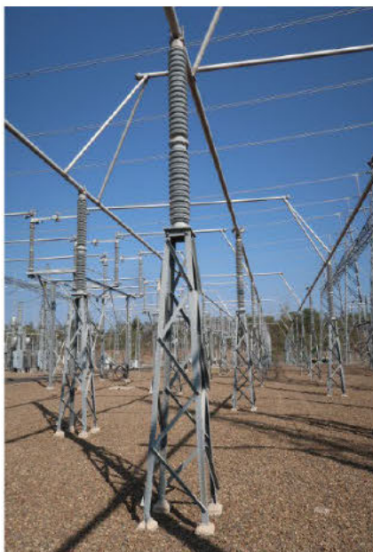
Figure 15: 275kV Lattice Bus Support Structure
