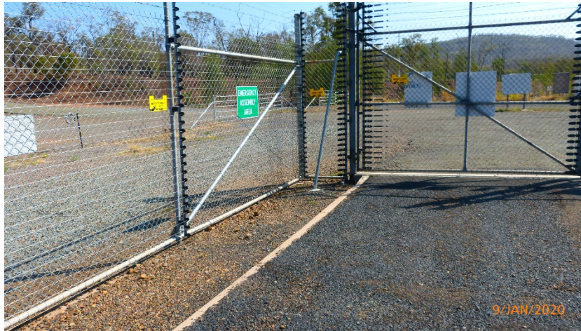
Figure 29: Broken road surface
