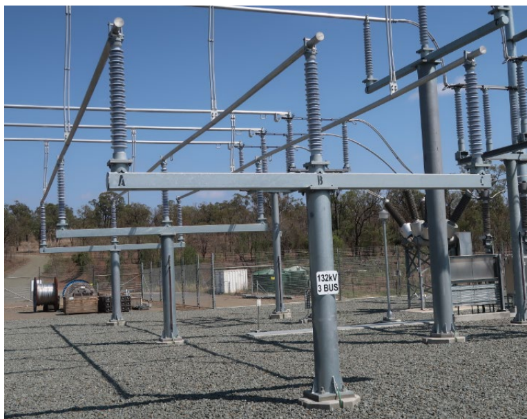
Figure 17: 132kV Bus Support Structure
