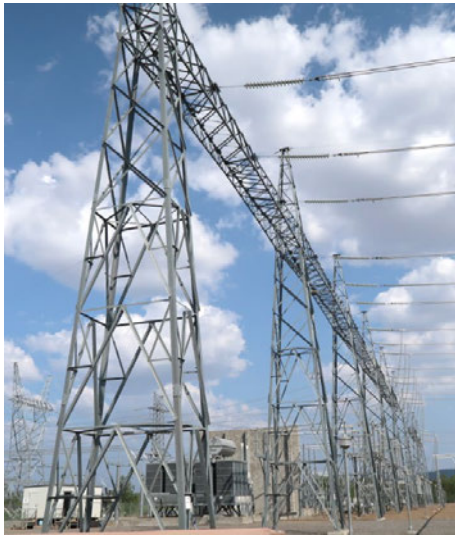
Figure 21: 275kV Strain Structure
