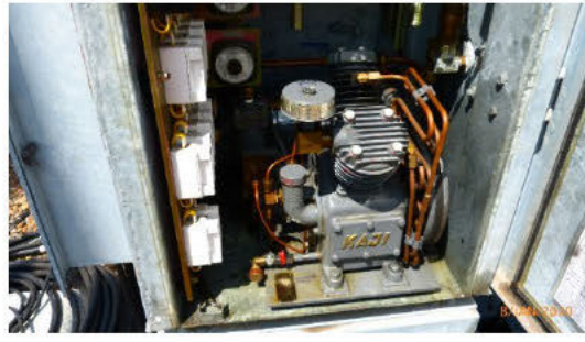
Figure 14: CB Mech box oil leak
