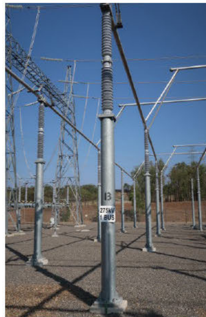
Figure 16: 275kV Tubular Bus Support Structure
