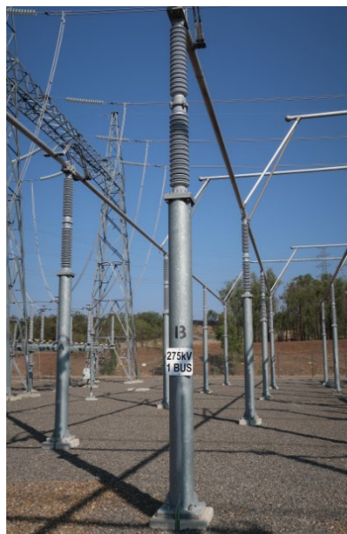
Figure 18: 275kV Tubular Bus Support Structure
