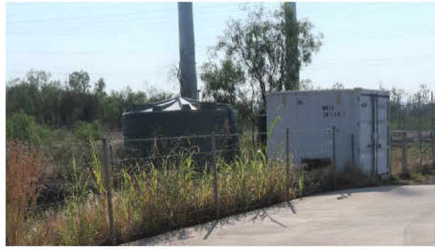
Figure 7: Water Tanks at wash-down station
