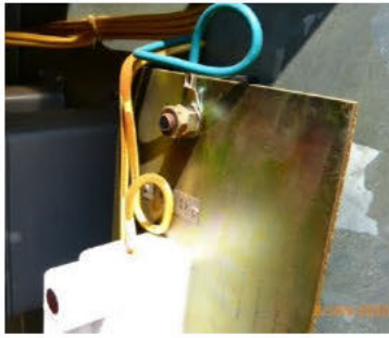
Figure 13: Wiring UV damages
