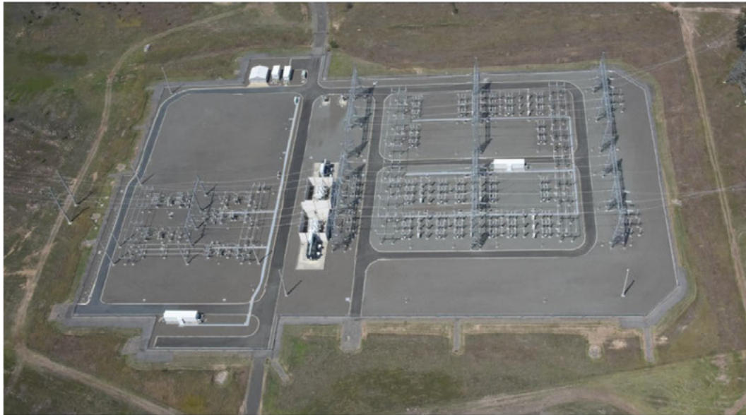
Figure 1-1: Teebar Creek Substation Aerial View
