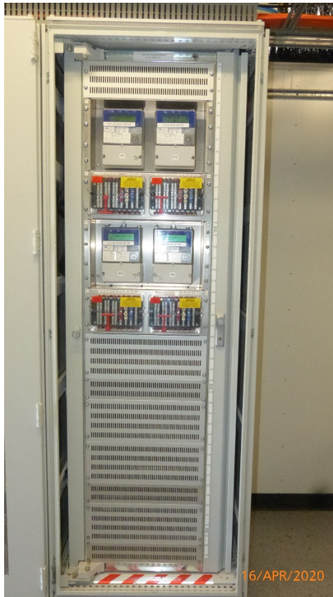
Figure 9 – Teebar Creek substation typical revenue metering panels
