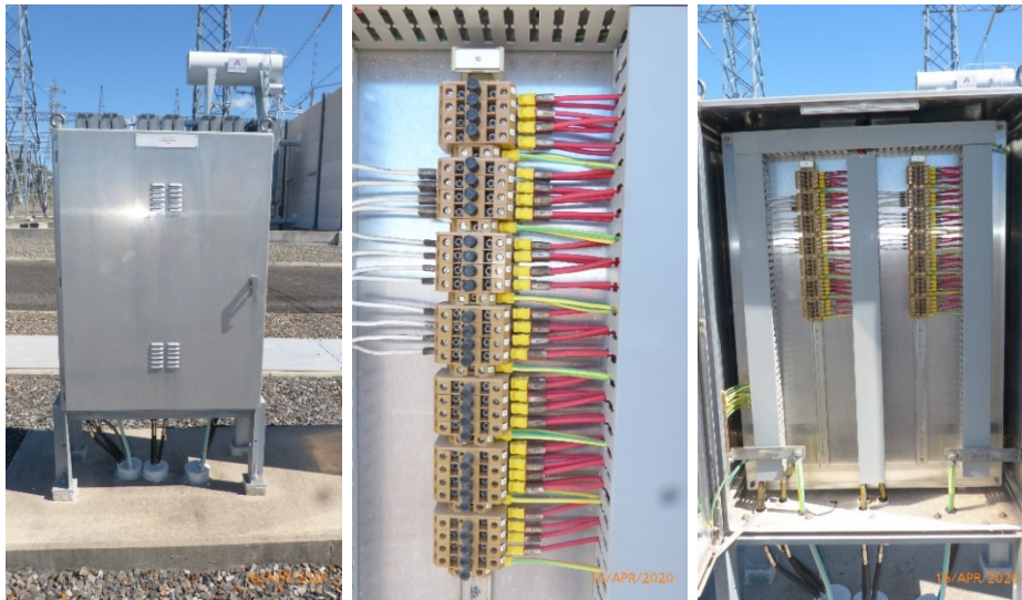
(a) 132kV - 2 Bus Marshalling Kiosk (+KD2-A1)
