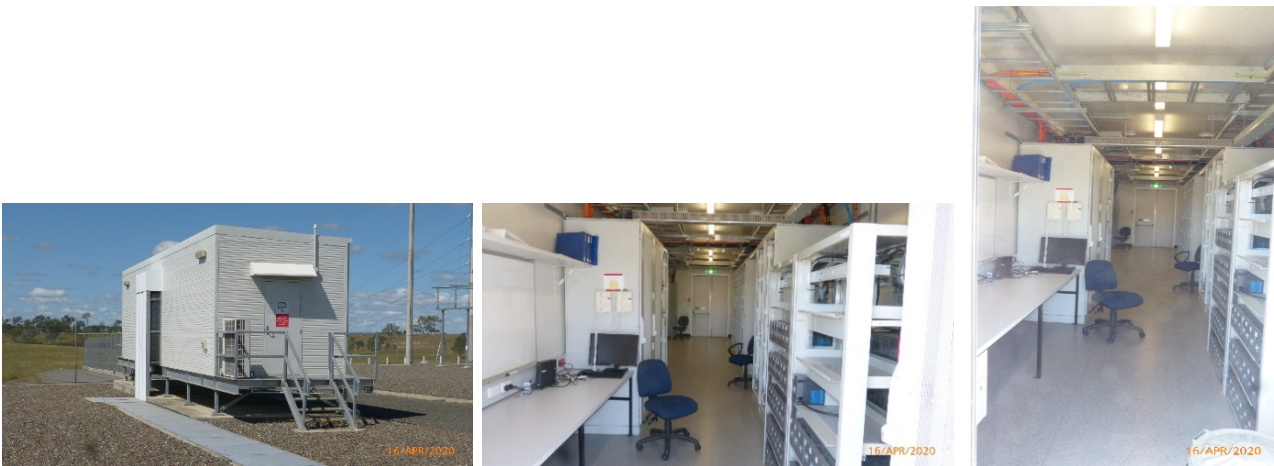
(c) 132kV Demountable Control Building +3
