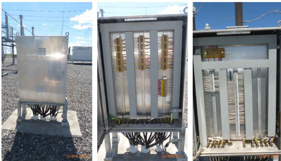
(f) 275kV Bay =C05-Q10 Feeder 8850 Marshalling Kiosk (+C05-A10)
