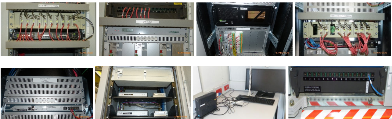
Figure 12 – Teebar Creek Substation Typical OpsWAN Equipment
