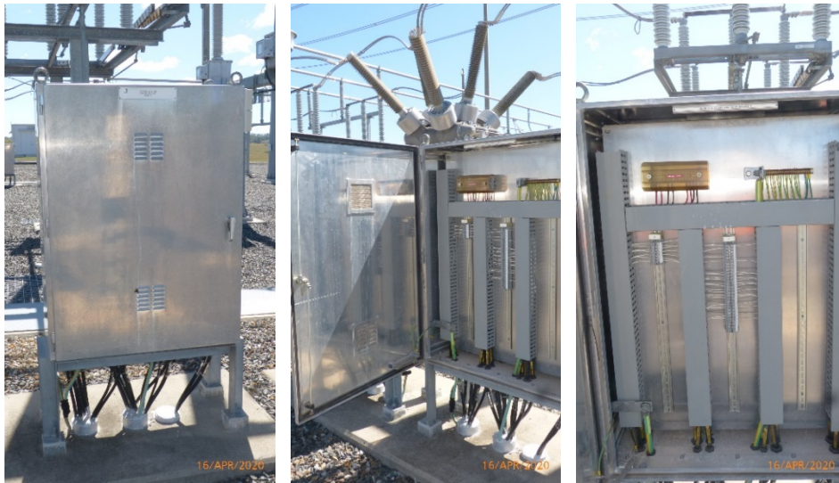
(c) 132kV Bay =D09 Marshalling Kiosk (+D09-A10)
