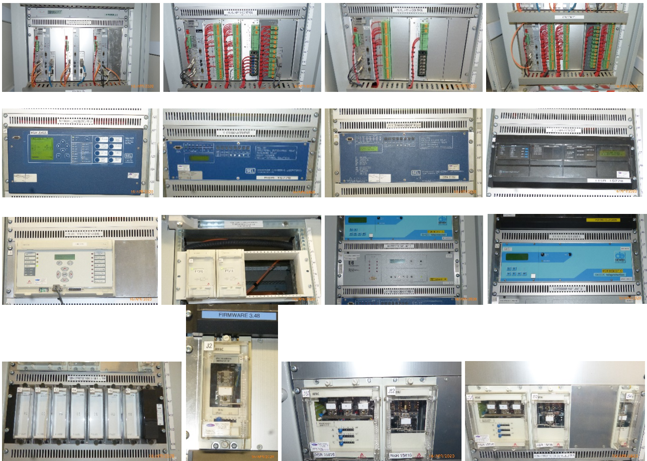
Figure 8 – Teebar Creek Substation Typical Indoor Secondary System Equipment (2007)
