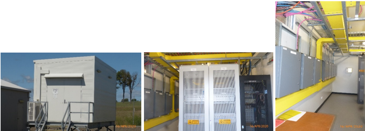
(b) Telecommunication Building and OpSWAN Server +2
