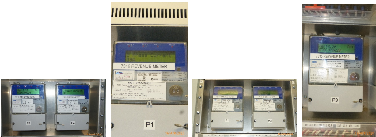
Figure 10 – Teebar Creek substation typical revenue meters
