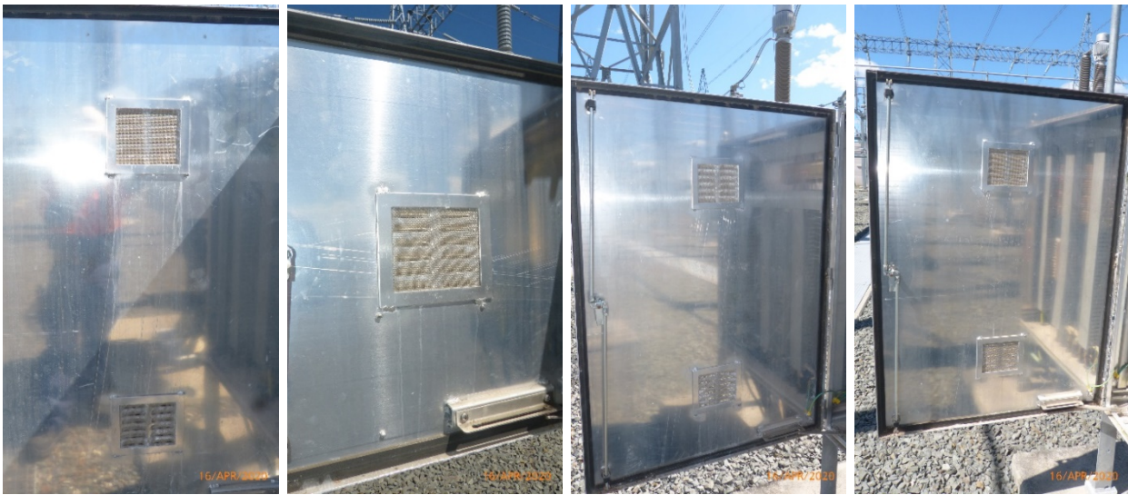
(a) Outdoor Marshalling Cubicle Doors with Unsuitable Mesh Filters and Door Seal
