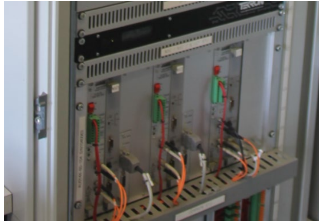
SCADA NSC1/NSC2 RTU and LCF RTU
