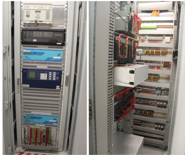
Feeder 8842 protection and control panel
