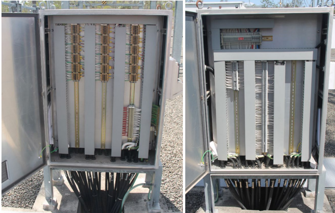
275kV Coupler 507 bay marshalling kiosk
