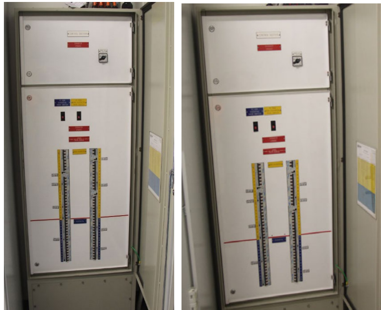
AC distribution board in Building +3 and +4
