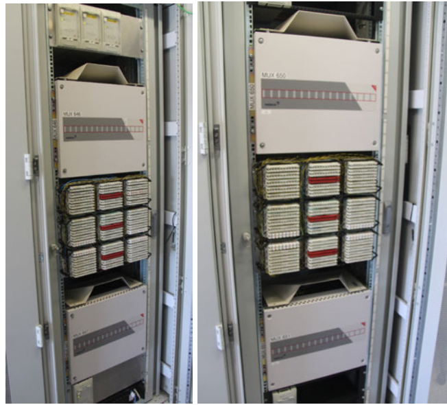
PDH at Building +3 and +4
