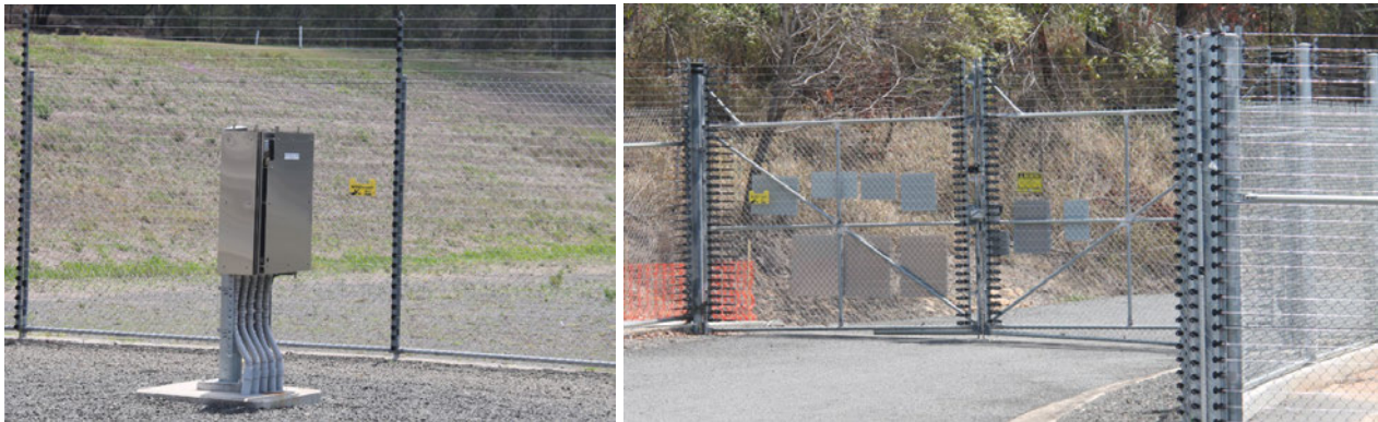
Electric fence and associated control cubicle
