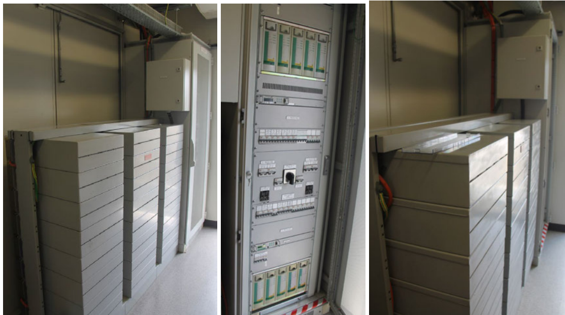
125VDC Batteries and charger in Building +3 and +4
