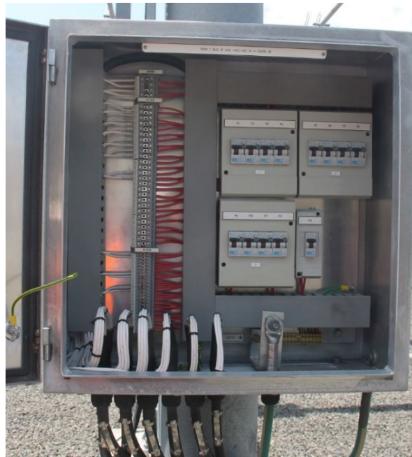
110kV 2 Bus VT box
