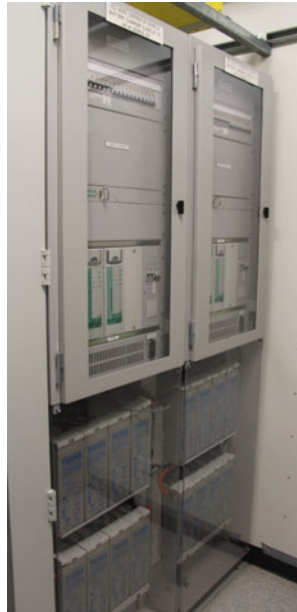
48VDC Batteries and charger in telecommunication building +2
