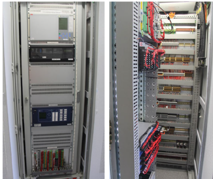
Feeder 8819 protection and control panel
