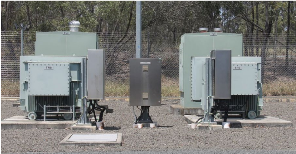
Energex Station transformer TR8 and TR9
