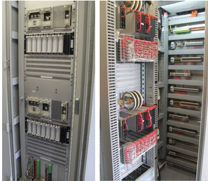
110kV 1 Bus zone protection and control panel
