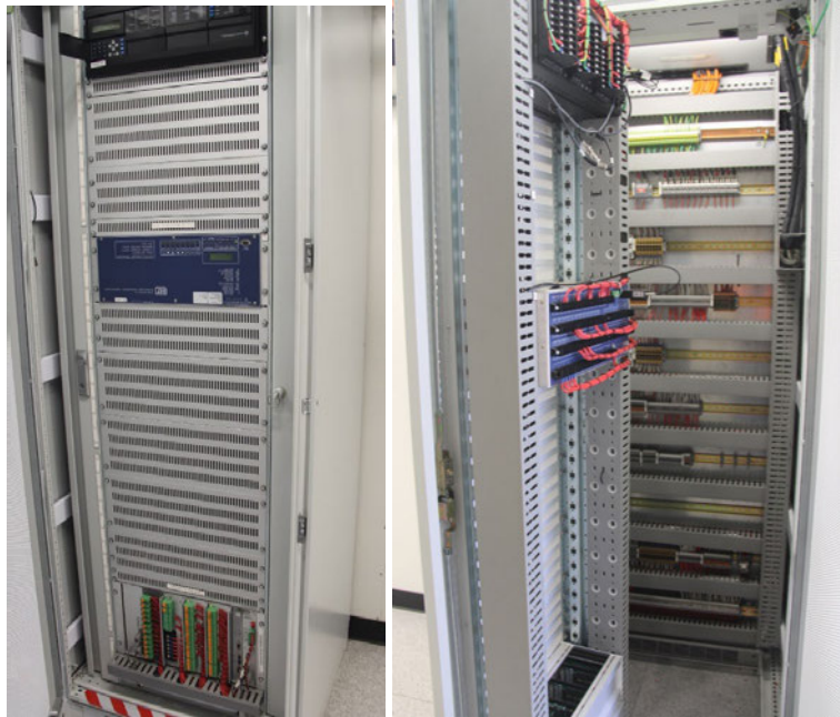
Coupler 504 protection and control panel
