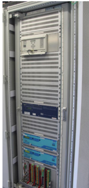
Feeder 791 protection and control panel
