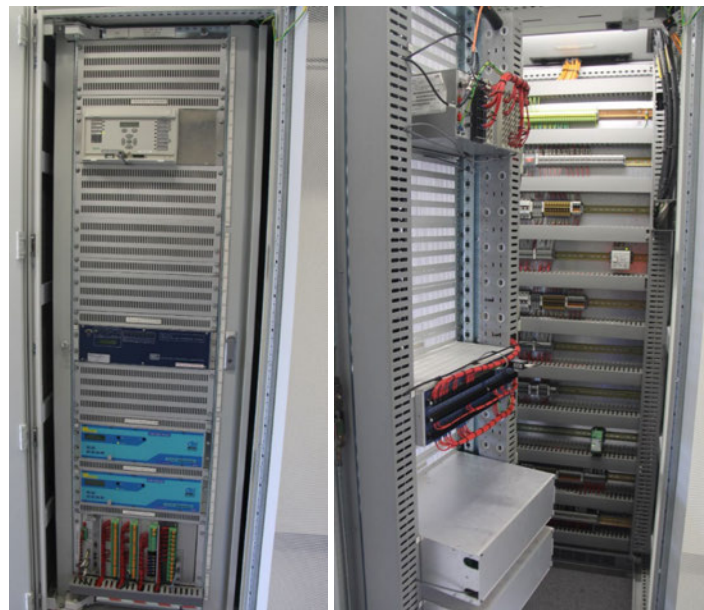
Feeder 7295 protection and control panel
