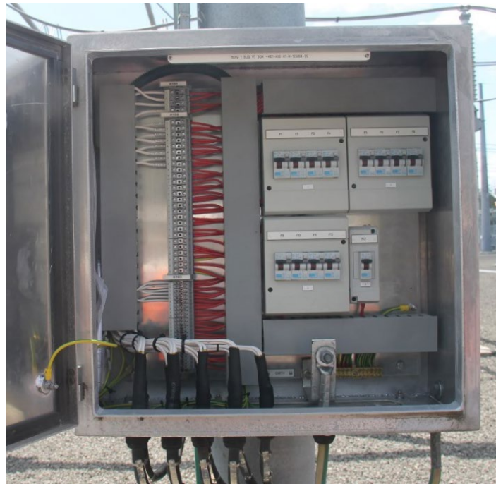
110kV 1 bus VT box
