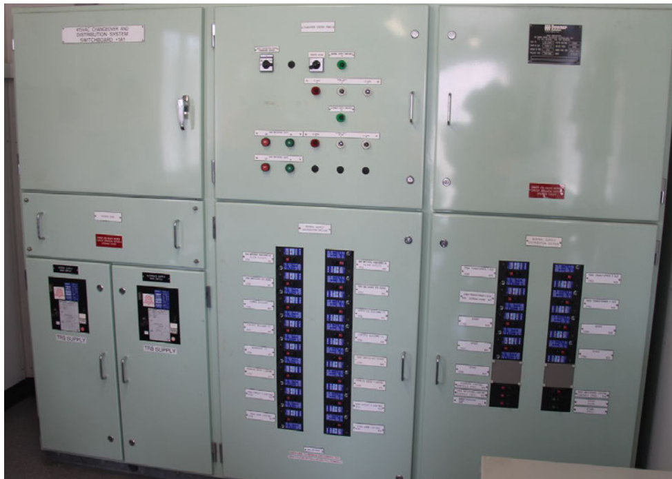
AC changeover board in Amenities building
