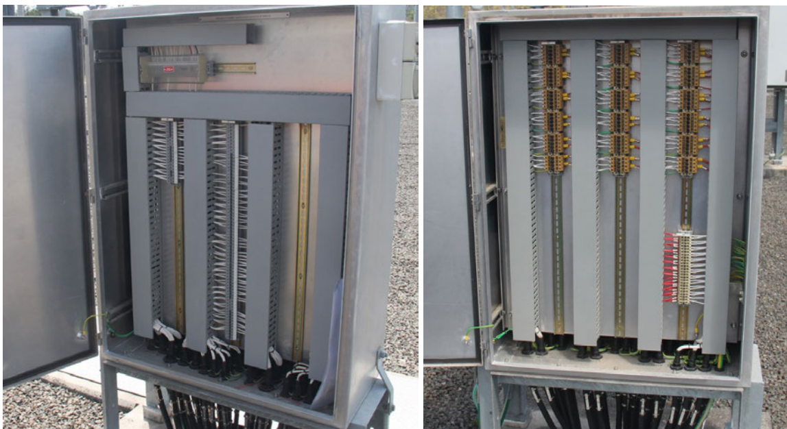
275kV Feeder 8819 bay marshalling kiosk
