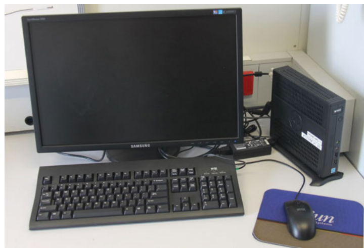
HMI Wyse Terminal in Building +4
