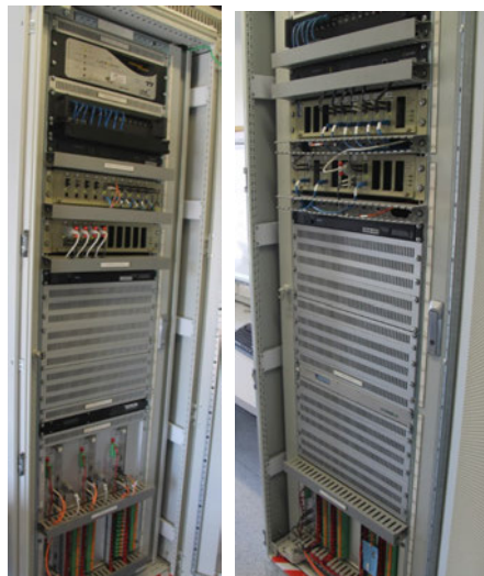
Station OpsWAN panel in Building +3 and +4
