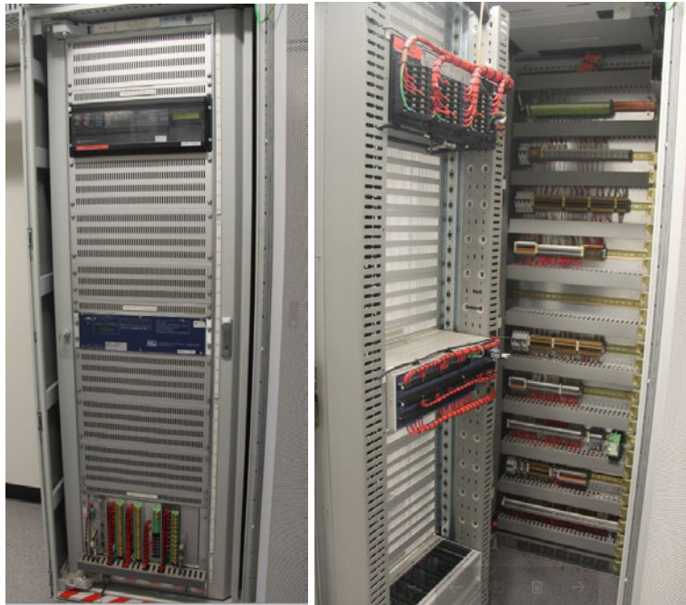
110kV 4T protection and control panel
