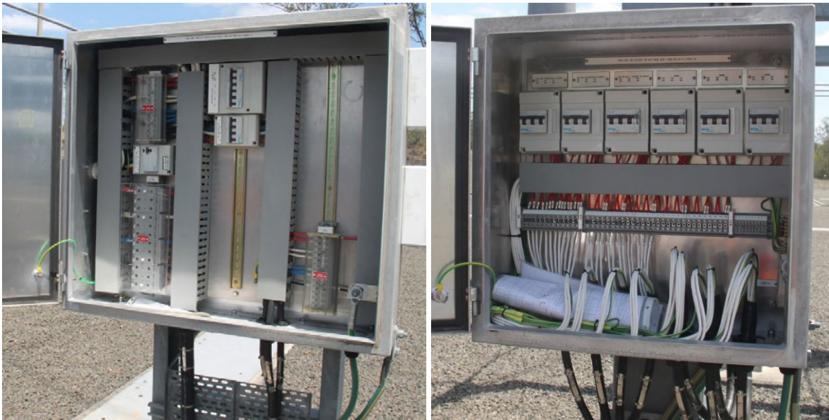
110kV Bay =D06 Feeder 718 bay AC supply and VT box
