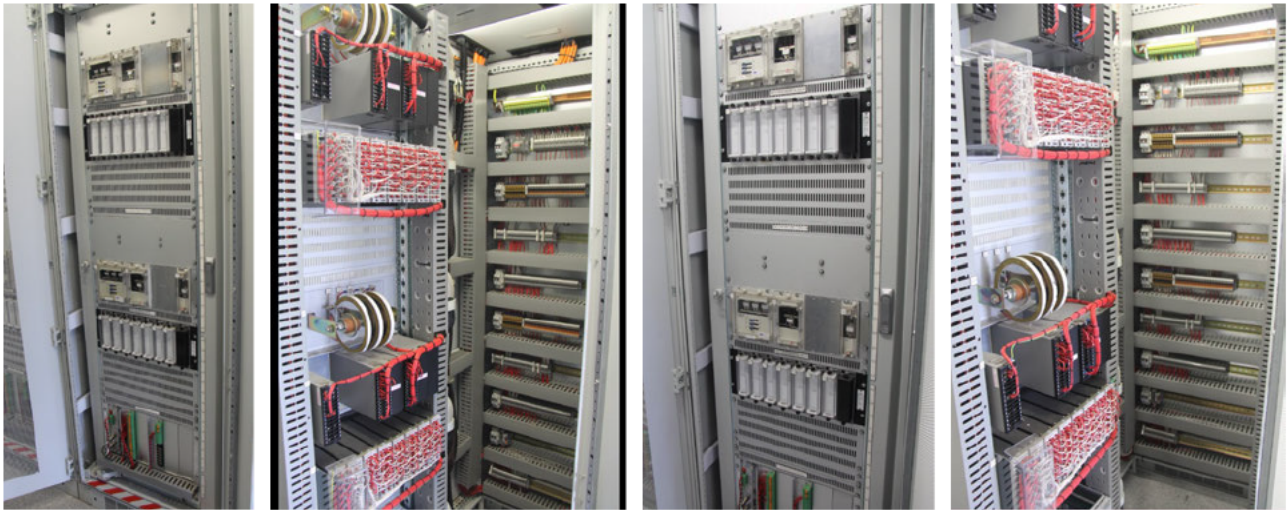
275kV 1 & 2 Bus protection and CB fail bus trip panel
