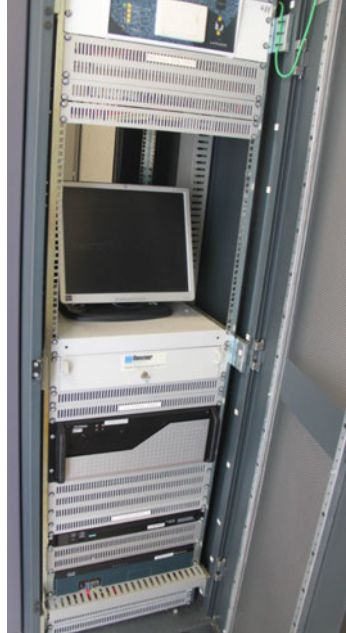
Master OpsWAN panel in Building +2
