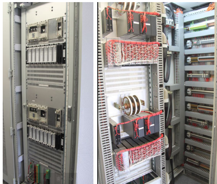
110kV 2 Bus zone protection and control panel
