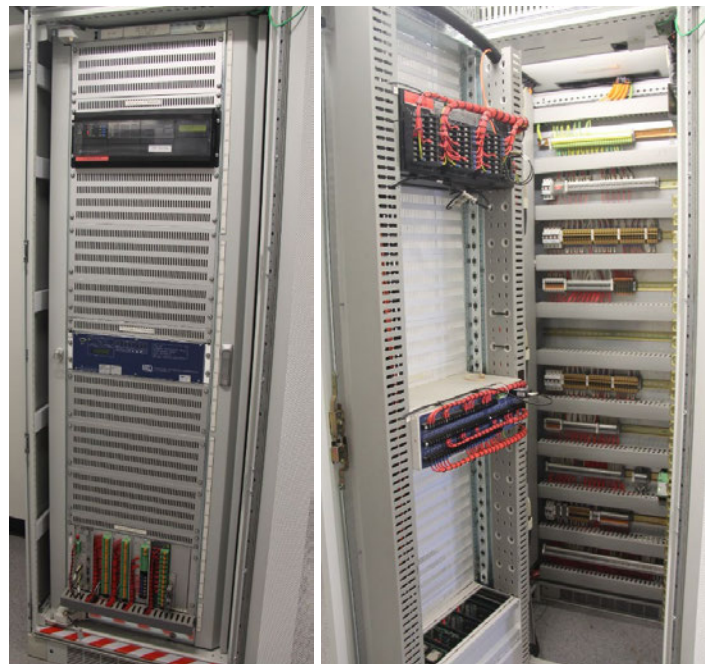
110kV 5T protection and control panel
