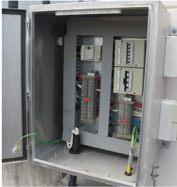
T4 oil filter/maintenance outlet kiosk
