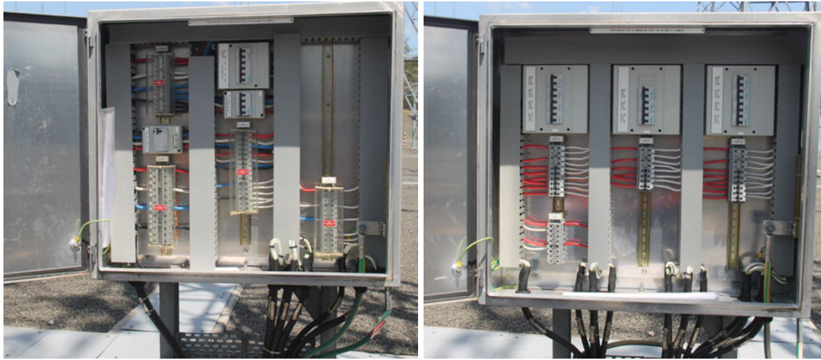
275kV =C07 AC and DC marshalling kiosk
