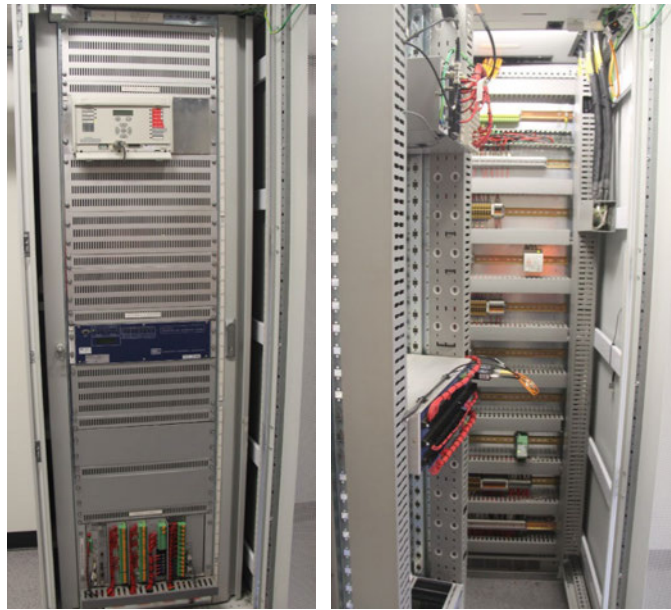
Feeder 718 protection and control panel
