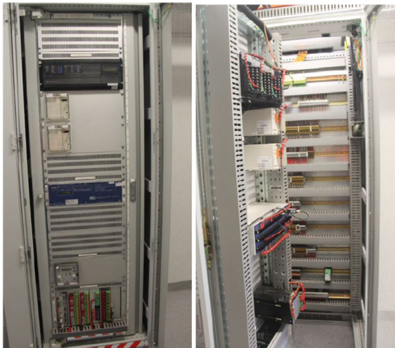
3 CAP protection and control panel
