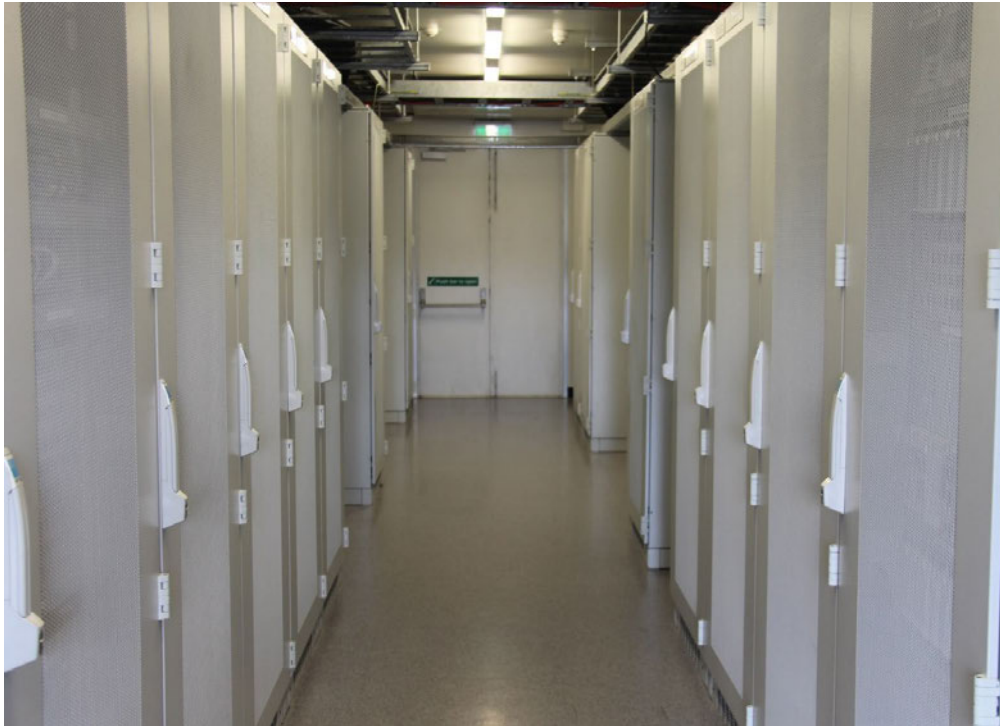
Control building +3 inside
