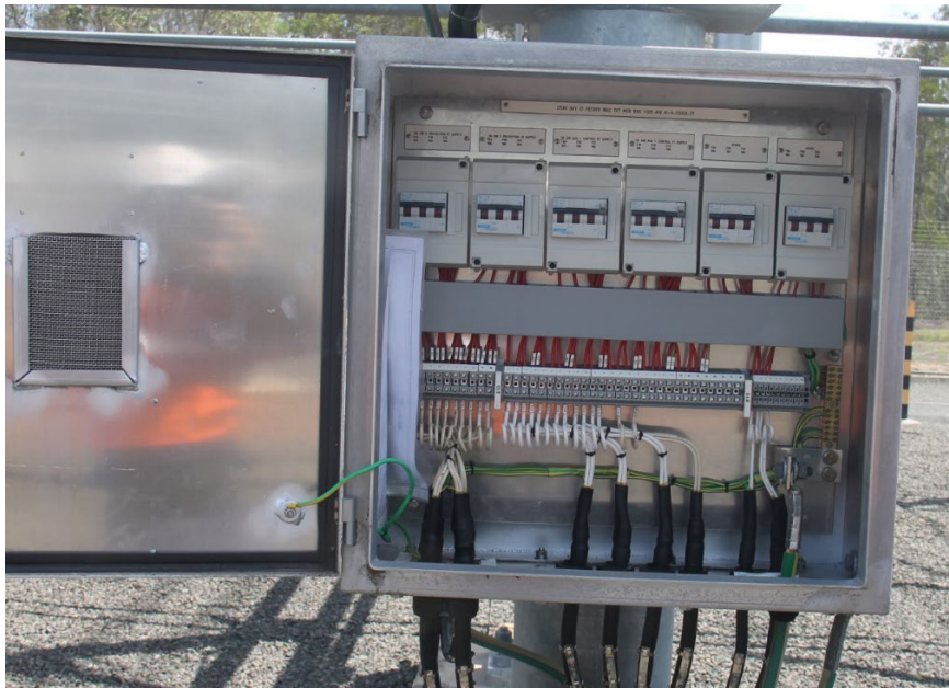
275kV Feeder 8842 VT box
