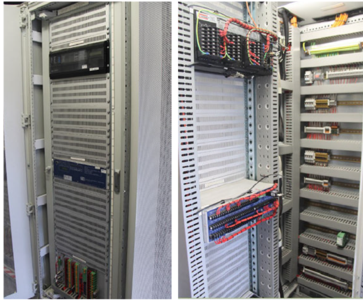
110kV Bus coupler protection and control panel
