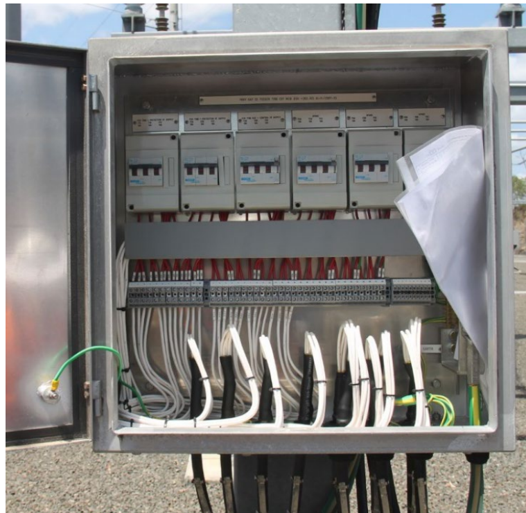
110kV Bay =D03 Feeder 7296 bay VT box
