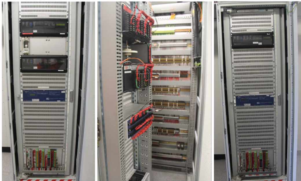
1 Transformer 275/110kV protection and control panel
