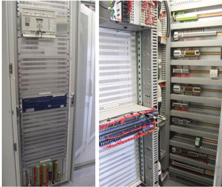
Feeder 7296 protection and control panel
