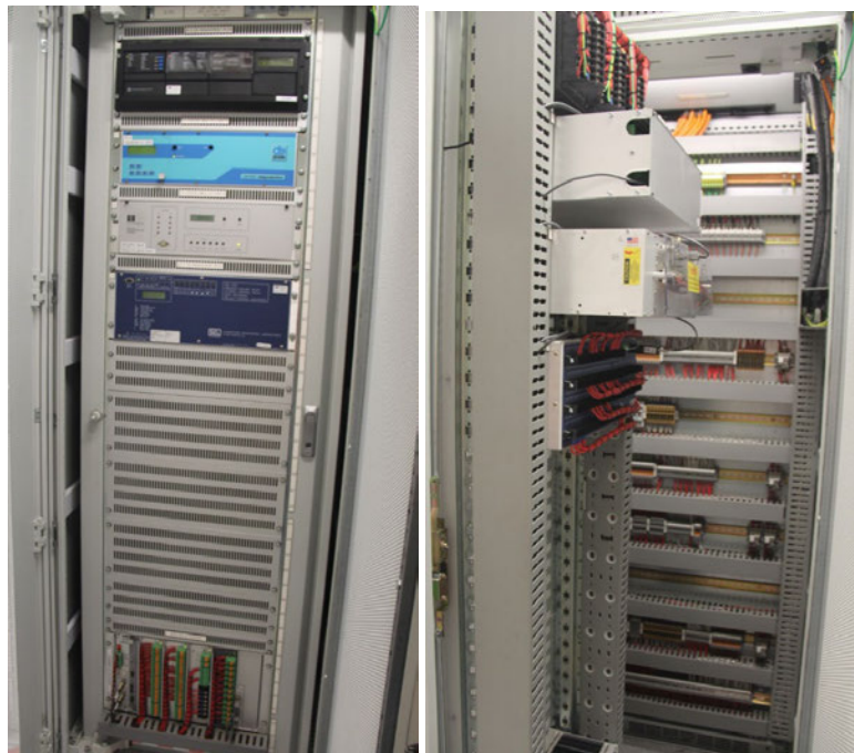
Coupler 507 protection and control panel
