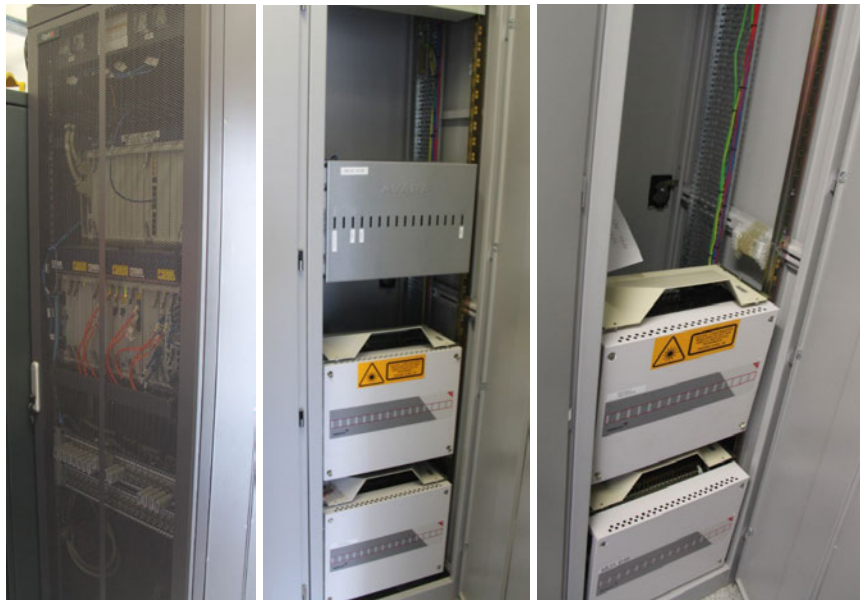
SDH and PDH at Building +2
