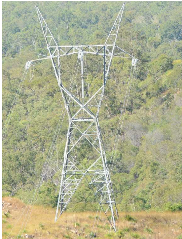
Figure 3: 1122-STR-4863 - Tension Tower
