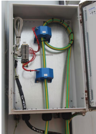
GIC transformer neutral monitoring system
