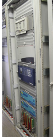
Feeder 8848 protection and control panel
