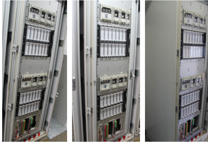
110kV Bus zone protection and control panels
