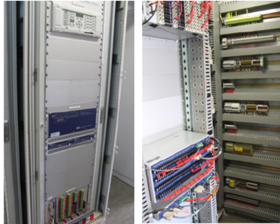
=D1.3 Feeder 730 protection and control panel
