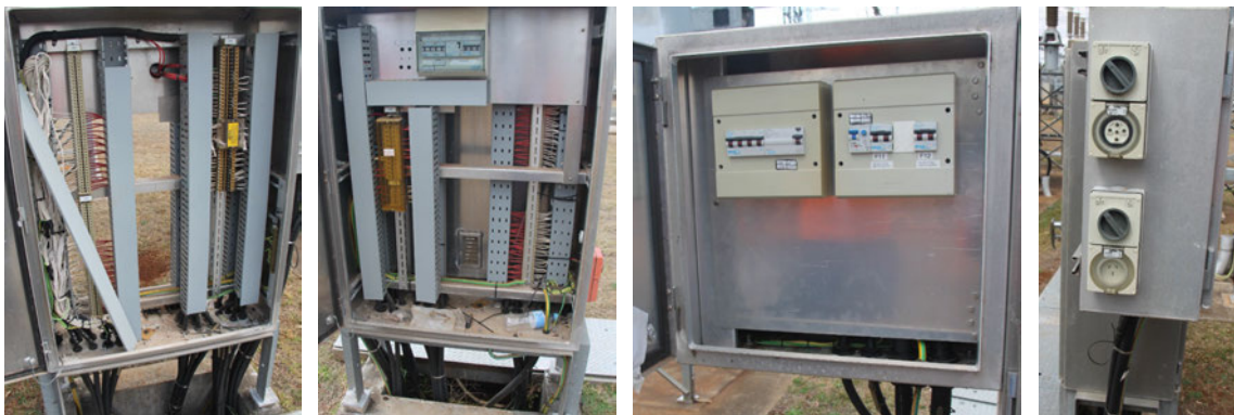
=D1.2 Feeder 728 marshalling kiosk
