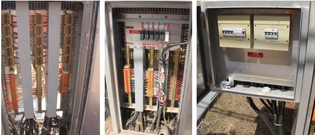
=D8 110kV Transformer 3 marshalling kiosk
