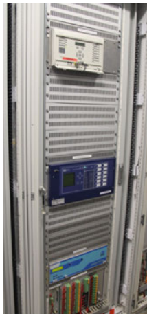
Feeder 8849 protection and control panel
