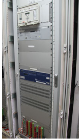
=D5.2 Feeder 732 protection and control panel
