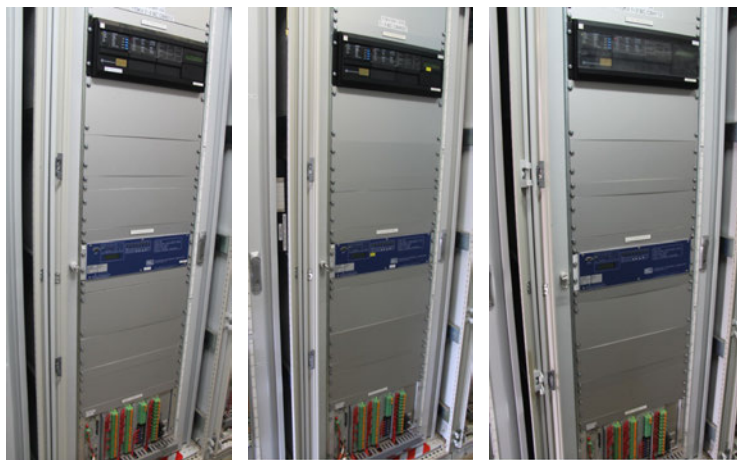
110kV bus coupler 401, 402 and 411 protection and control panel
