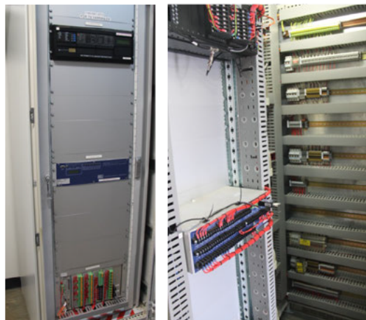
=D7.3 Feeder 734 protection and control panel
