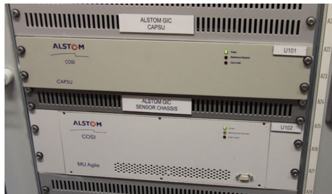
Transformer HV GIC monitoring system
