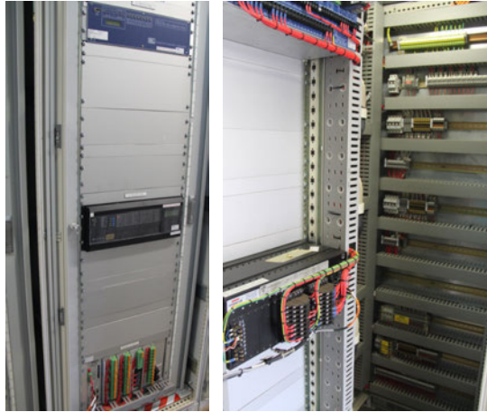
=D2.3 Feeder 7233 protection and control panel
