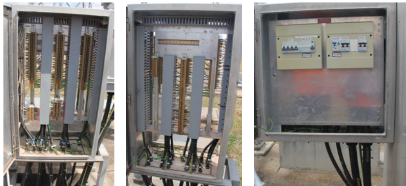
=D6 Feeder 731 marshalling kiosk
