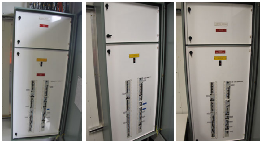
AC distribution board within building +6, +7 and +8
