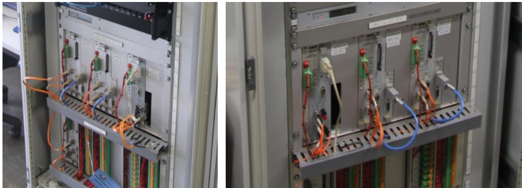
LCF and SCADA RTUs (330/275kV and 110kV)
