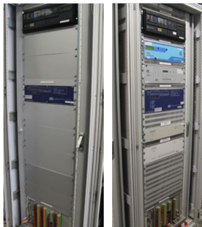
275kV bus coupler 501 and 504 protection and control panel
