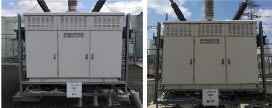
1 and 2 CAP protection and control panel
