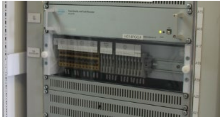
Power Quality Monitoring Panel
