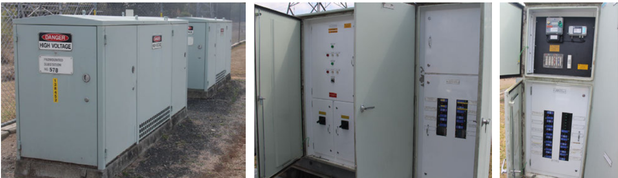
415VAC station transformer and AC changeover board
