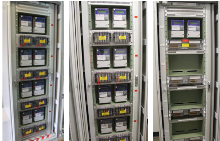
Metering panel (+6A9, +7A8 and 7A9)
