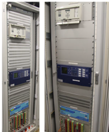
330kV =B02 Feeder 9907 and =B01 Feeder 9908 protection and control panel
