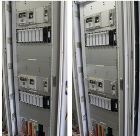
275kV 1 & 2 Bus zone and CB fail panels
