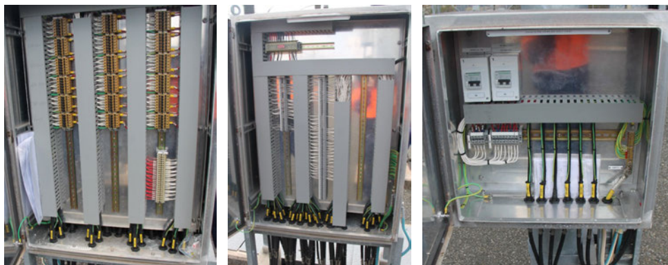
=C4 275kV 5 transformer CB marshalling kiosk and VT box
