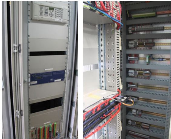
=D12.3 Feeder 7348 protection and control panel
