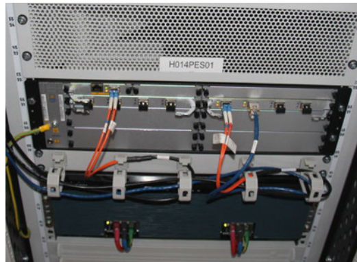
Site Infrastructure & MPLS panel
