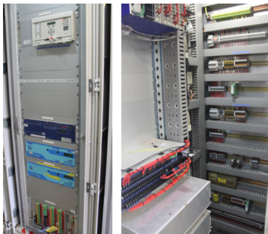
=D14.3 Feeder 735 protection and control panel
