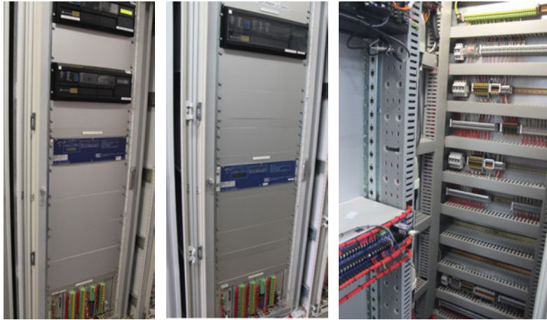
2T protection and control panel
