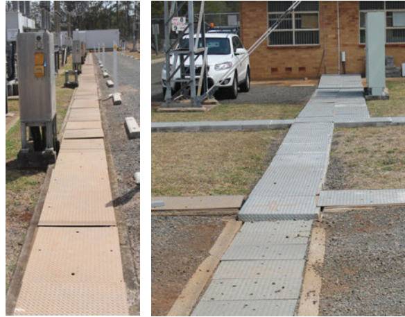
Typical substation trenches
