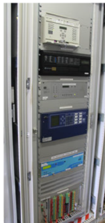
Feeder 831 protection and control panel
