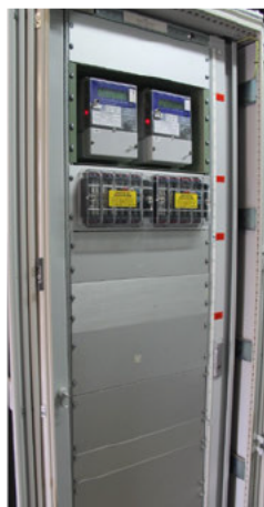
Feeder 727 metering panel (+6A8)
