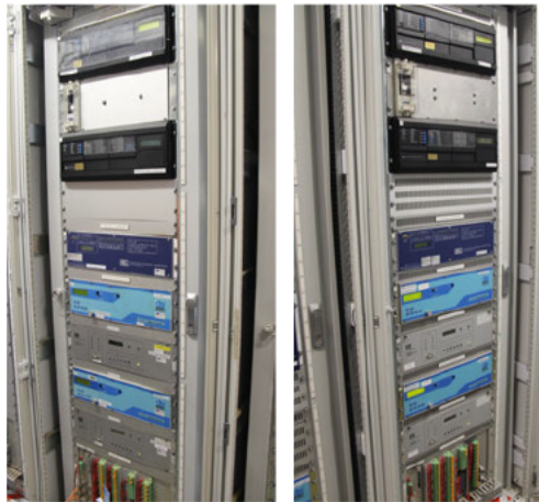
4 and 5 Transformer 275kV protection and control panel
