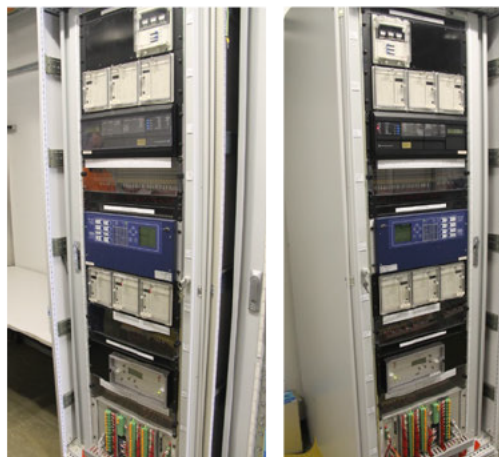
330kV 3 & 4 CAP protection and control panel
