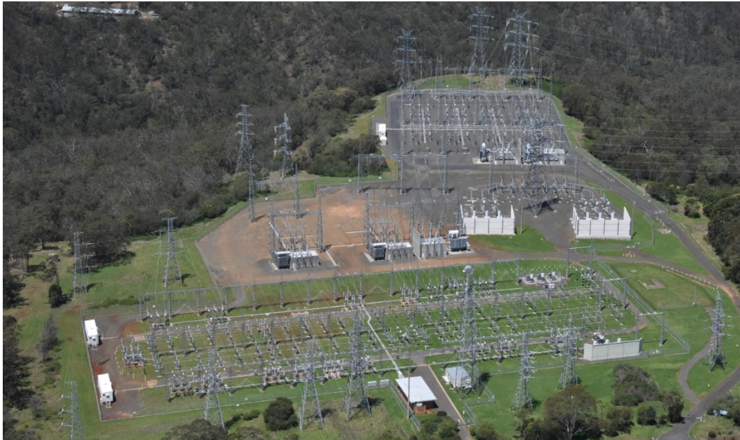
Figure 3-2 - Middle Ridge Substation yard bird view
