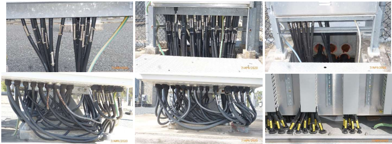
Figure 6 – Physical appearance of typical outdoor secondary system cables
