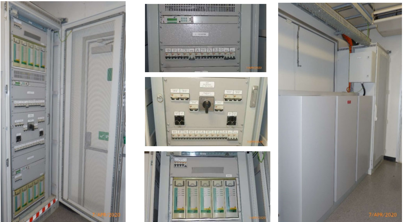
(Buildings +7 – Chargers, Monitors, DC Distribution 2006, Batteries 2006)
