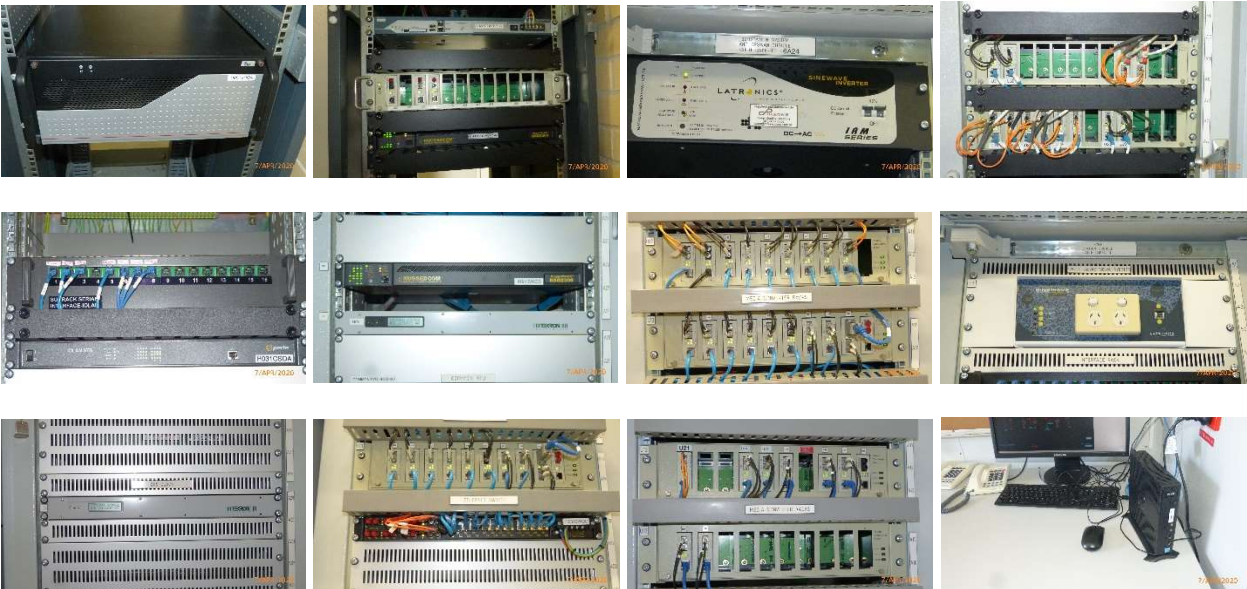
Figure 12 – Molendinar Substation Typical OpsWAN Equipment
