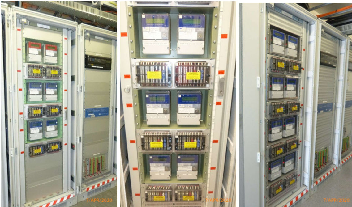
Figure 9 – Molendinar substation typical revenue metering panels
