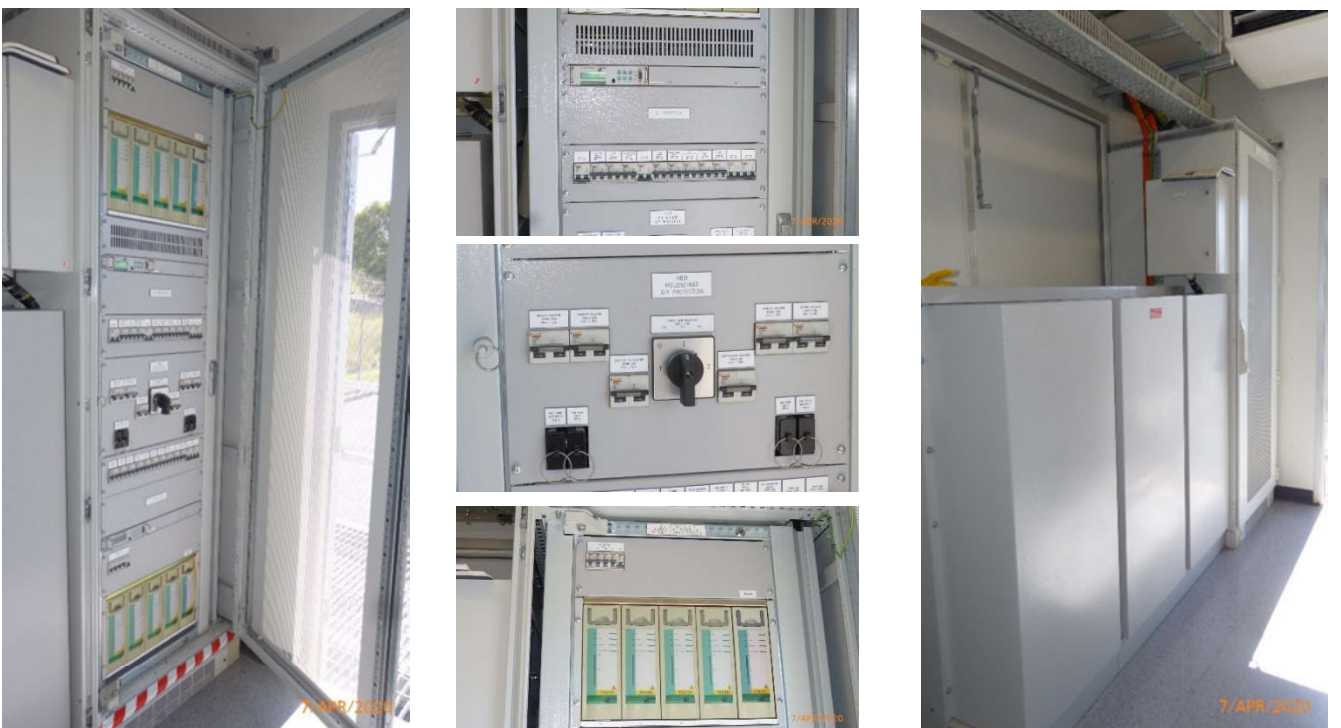
(Buildings +8 – Chargers, Monitors, DC Distribution 2006, Batteries 2006)
