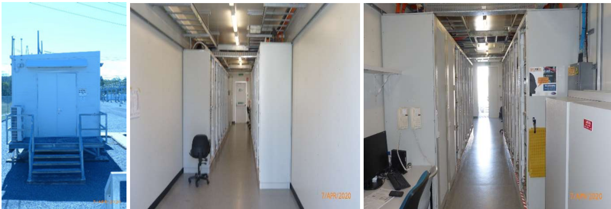
(c) Demountable Control Building +7
