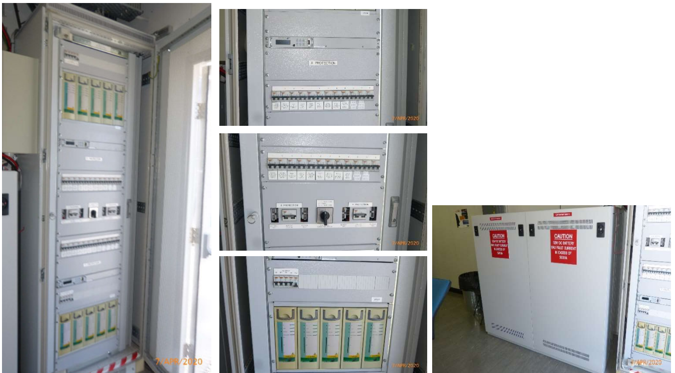
(Buildings +6 – Chargers, Monitors, DC Distribution 2009, Batteries 2017)
