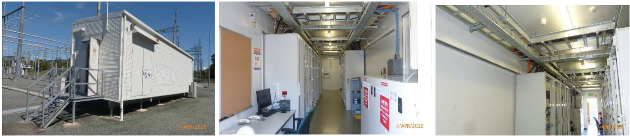
(b) Demountable Control Building +6
