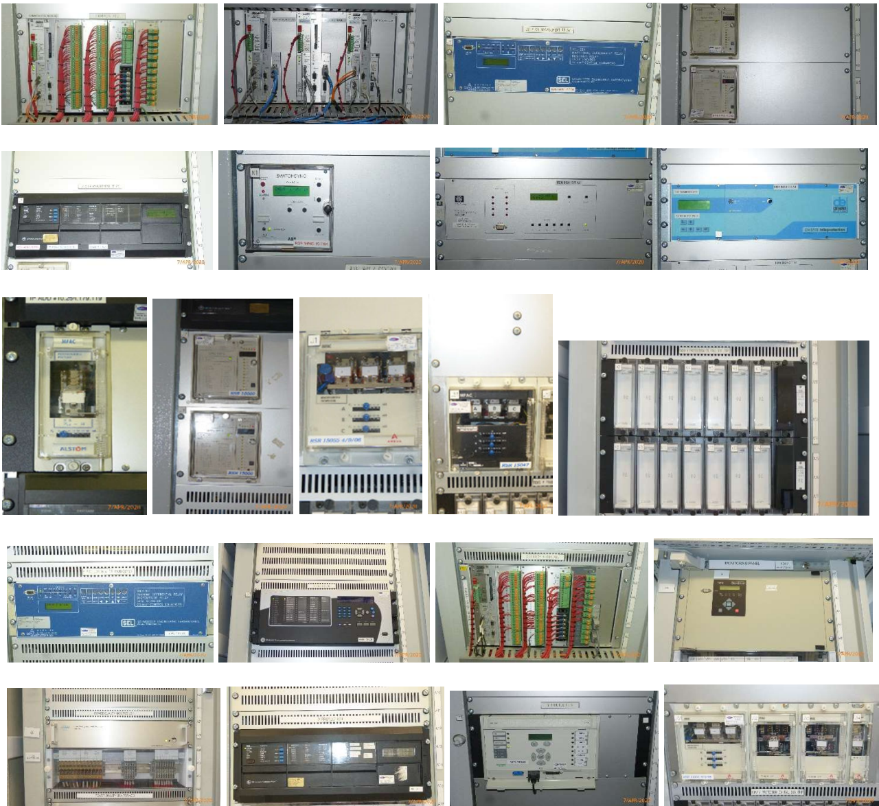
Figure 8 – Molendinar Substation Typical Indoor Secondary System Equipment (2003 - 2007)
