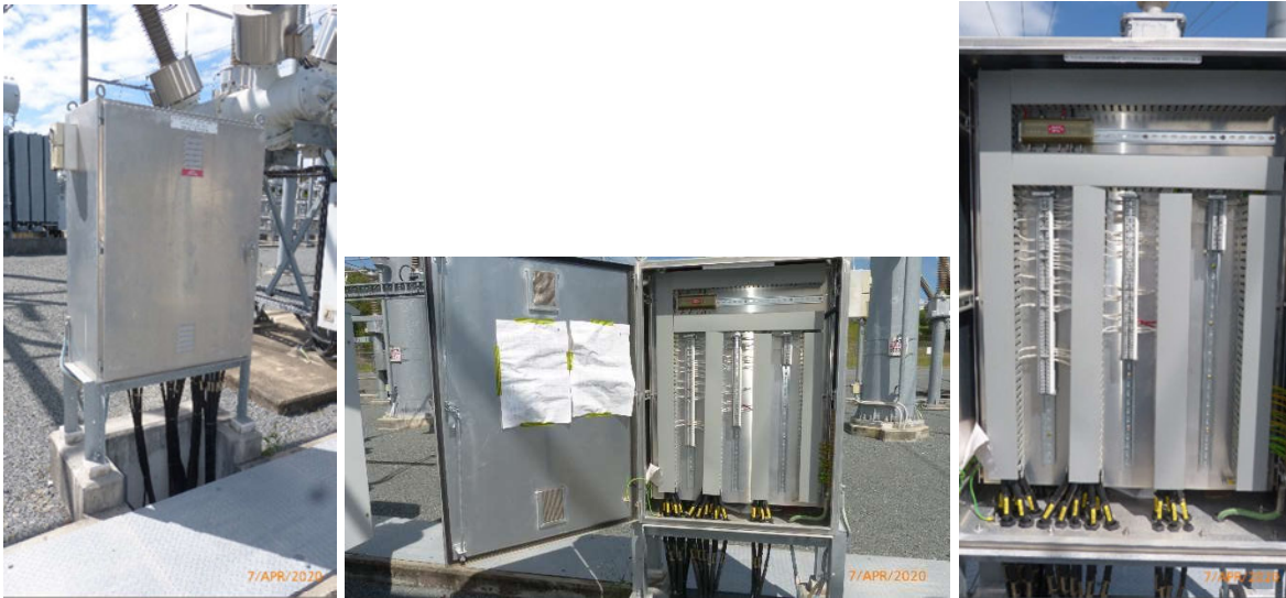
(a) 12 TFMR Deadtank CB Marshalling Kiosk (+D26-A10)
