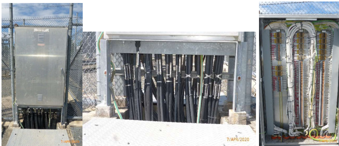
(c) Interface Marshalling Kiosk to Energex Switchyard (+U20-A10)
