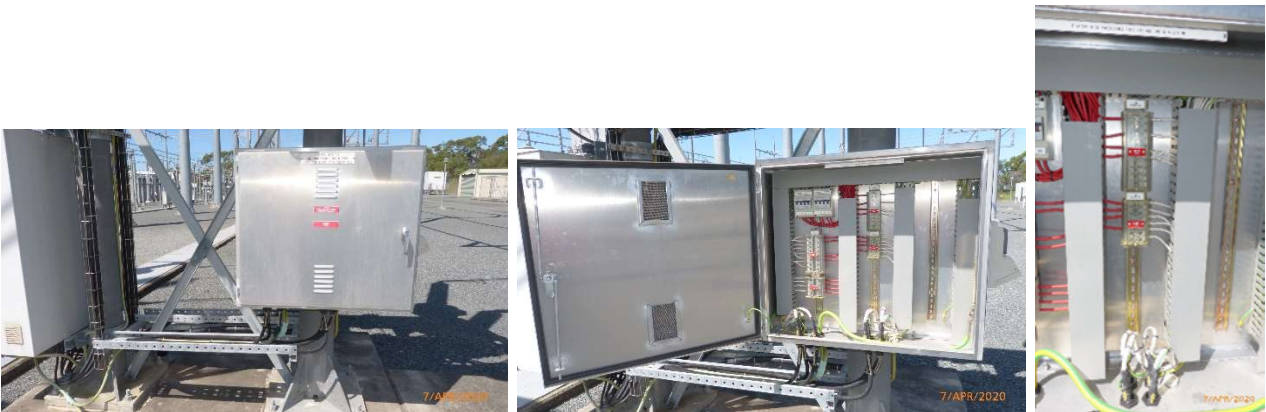
(e) CB79172 (F917 Southport) AC (+D13 A91) and DC (+D13 A92) Marshalling Kiosks
