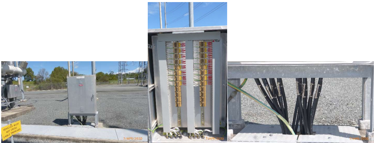
(b) 2 Bus CT Summation Marshalling Kiosk (+RD2-A10)
