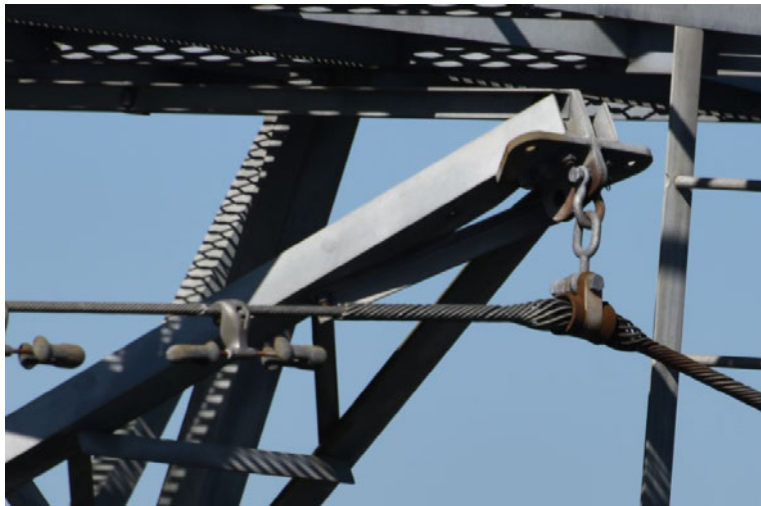
Figure 26: STR-0115 with corroded OPGW hardware and dampers (2018)
