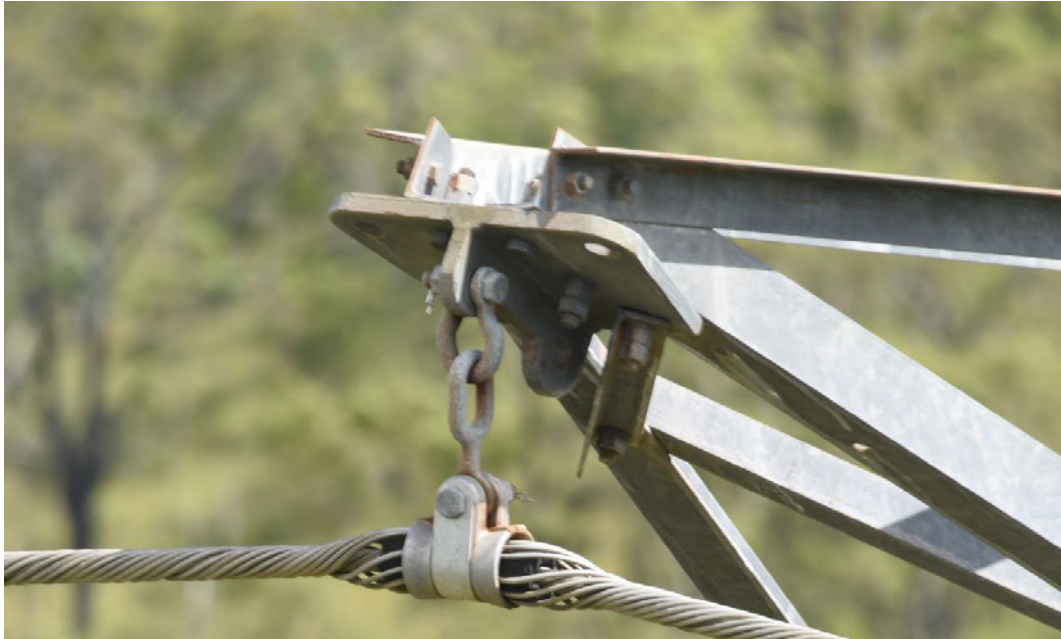
Figure 19: STR-0030 Earth Peak corrosion (2018)
