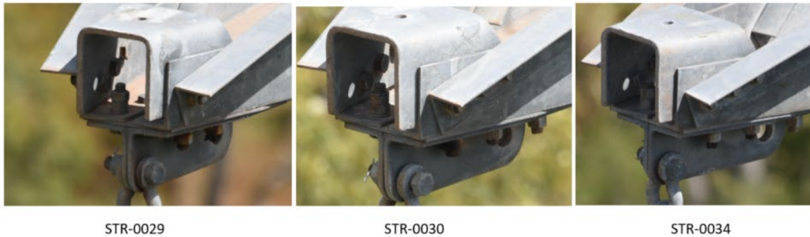
Figure 15: Examples of G4L corrosion in Attachment Zone fasteners (2018)
