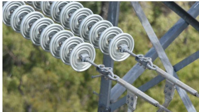
Figure 29: STR-0038 Tension Insulators (2018)
