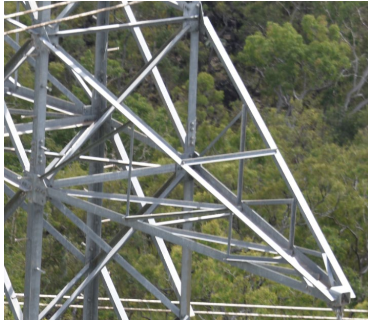
Figure 17: STR-0030 cross arm corrosion (2018)
