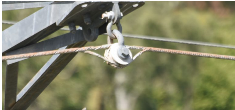
Figure 25: STR-0029 with corroded OHEW hardware (2018)
