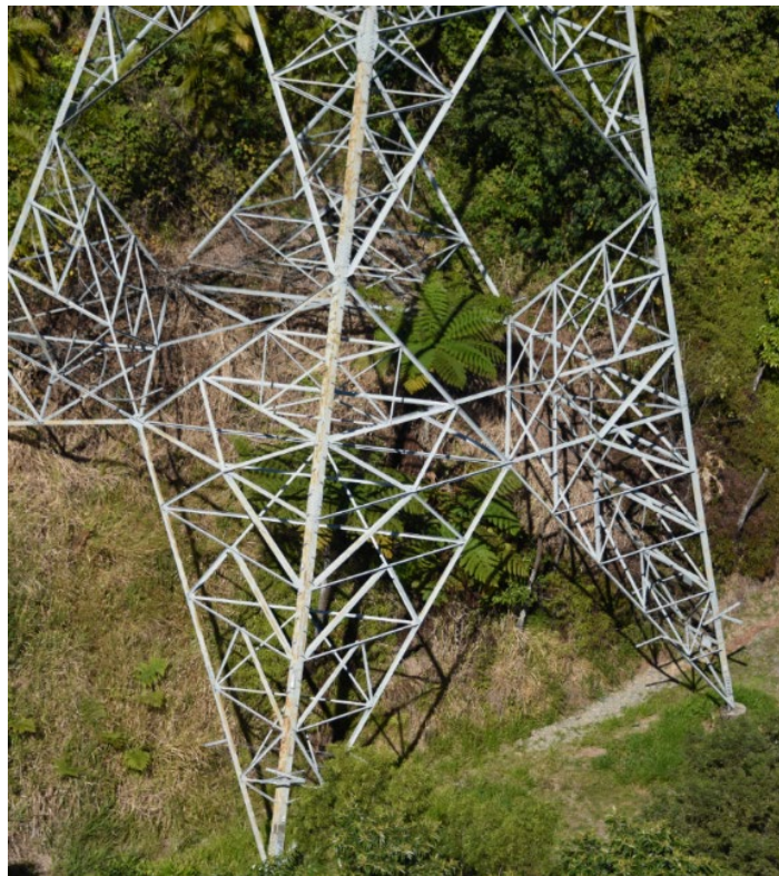
Figure 10: STR-01017; Sample of corrosion on tower base members
