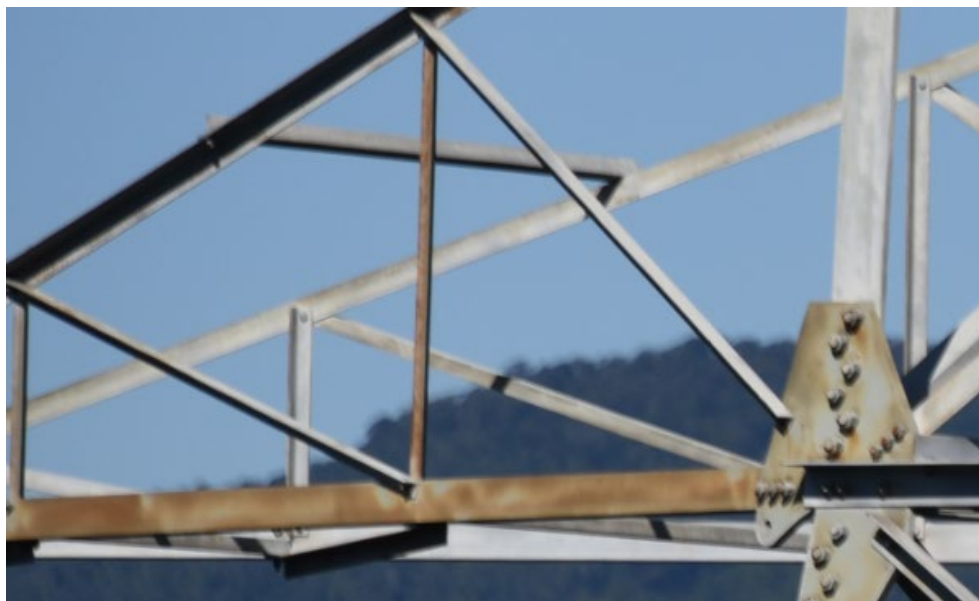
Figure 18: STR-0115 cross arm corrosion (2018)
