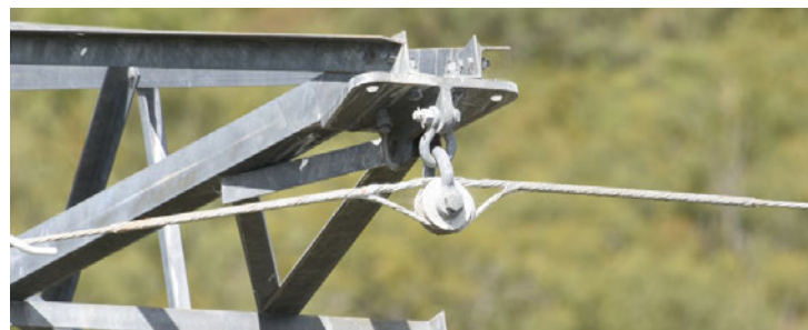
Figure 24: STR-0057 Example of earthwire and twingrip from the line (2018)
