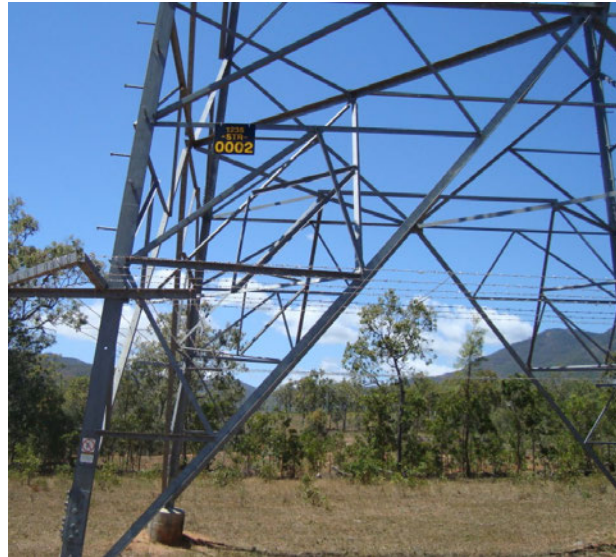
Figure 9: STR-0002; Sample of corrosion on tower base bolts (2015)
