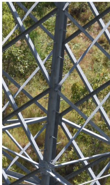
Figure 6: Grade 1 corrosion shown on step bolts 1235-STR-0034 (2018)
