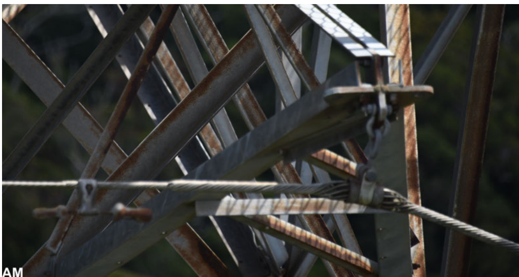
Figure 20: STR-0101 Corrosion on Earth Peak (2018)
