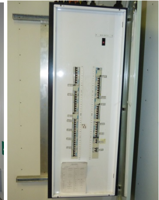
110kV building +C
