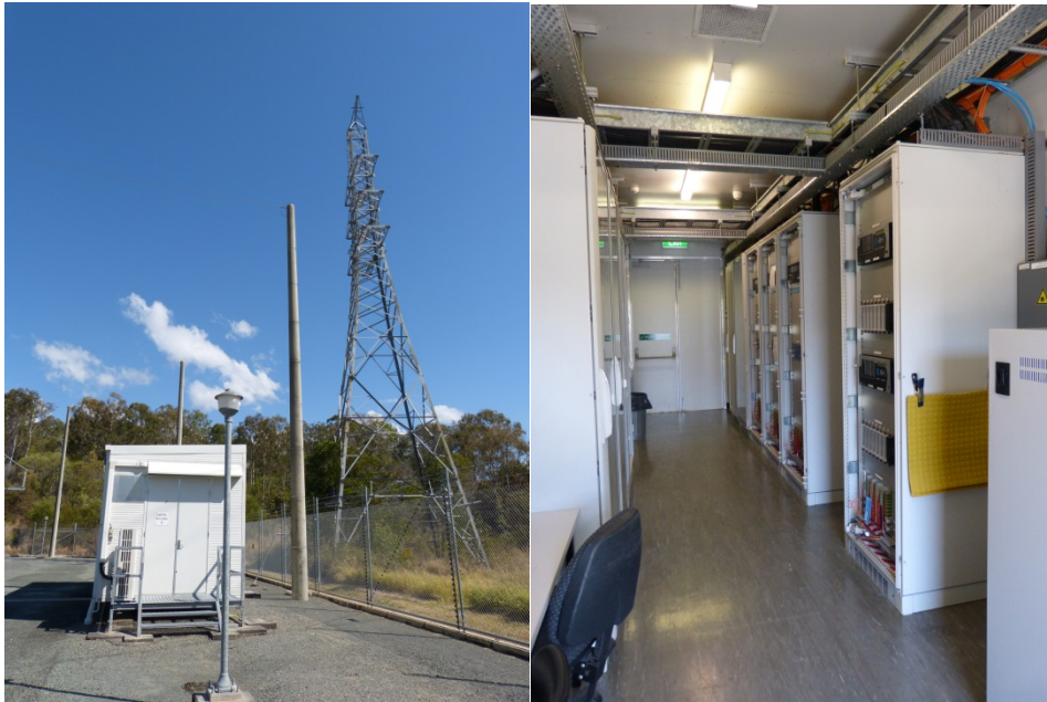
Figure 5 - H021 Murarrie 110kV Demountable Building "+B"
