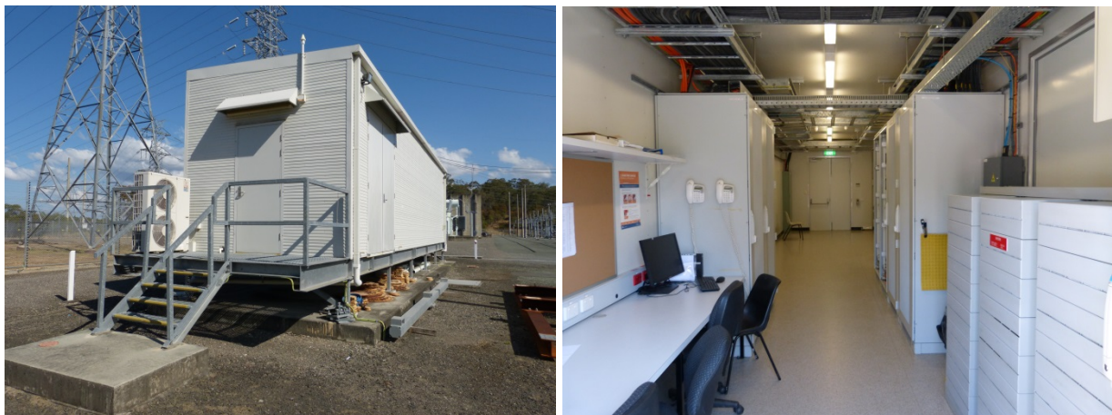
Figure 3 - H021 Murarrie 275kV Demountable Building “+5”
