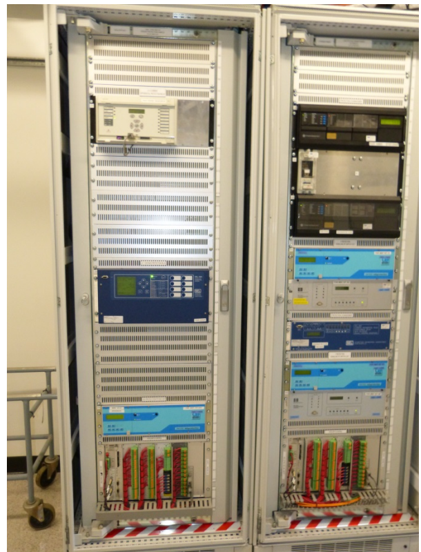
+5A4 - 275kV Bay =C02 - Fdr 8837 2008
