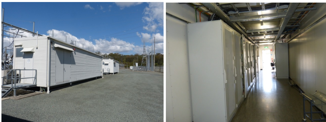
Figure 4 - H021 Murarrie 110kV Demountable Building “+A”
