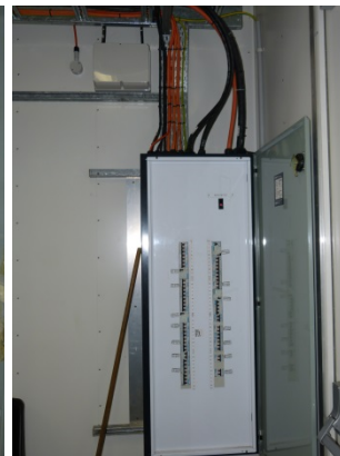
110kV building +B
