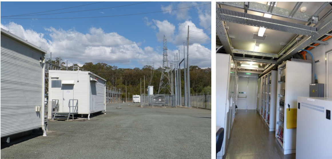
Figure 6 - H021 Murarrie 110kV Demountable Building "+C"
