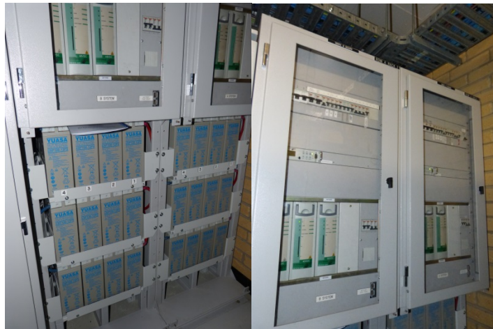
Building +T - 50VDC Batteries and Chargers
