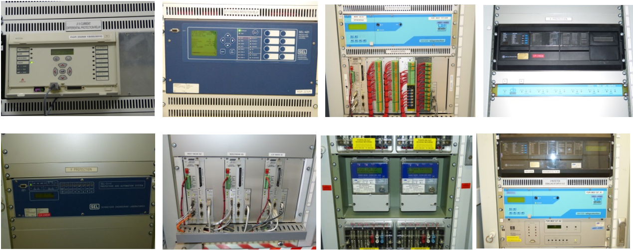
Figure 11 - Murarrie 275kV and 110kV – Typical Substation Secondary Systems Equipment
