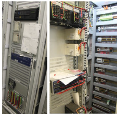
1 CAP protection and control panel
