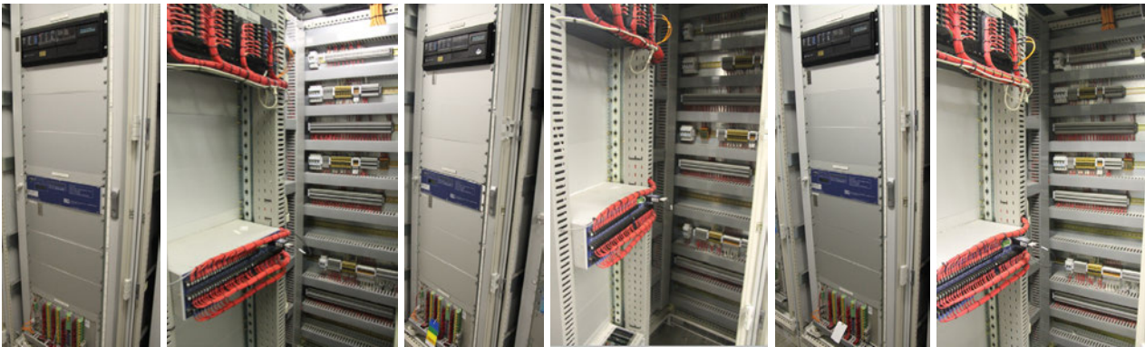
1-2, 2-3 and 3-4 bus coupler CB management and control panel
