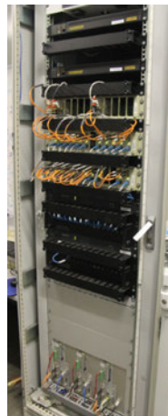
Substation master & OpsWAN cubicle
