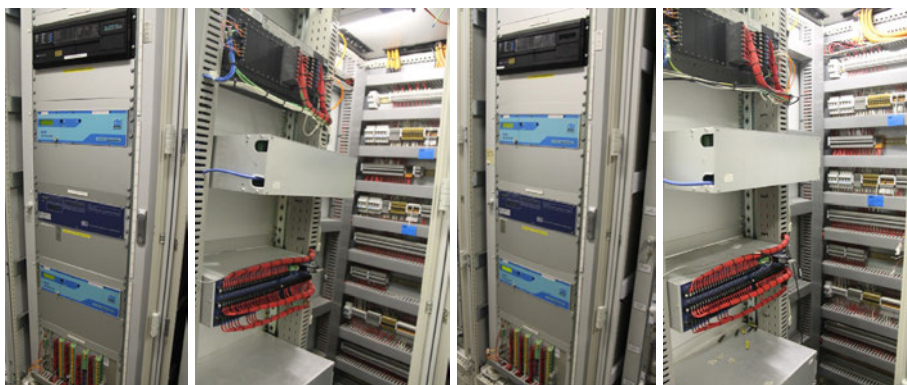
Feeder 7103 and 7147 protection and control panels
