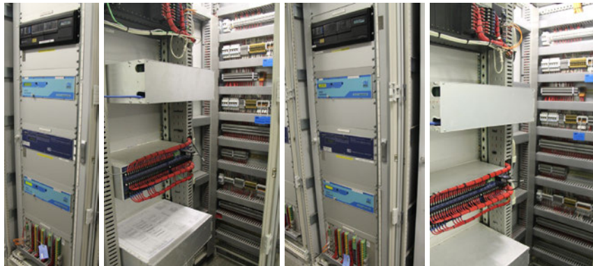
Feeder 7101 and 7102 protection and control panels
