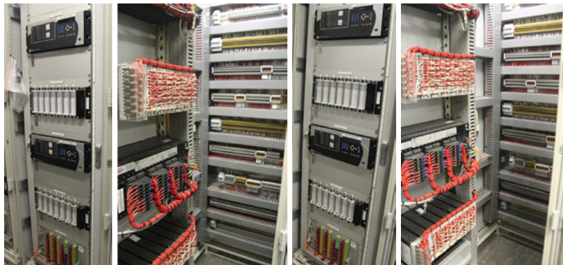
3 and 4 Bus zone protection and control panels
