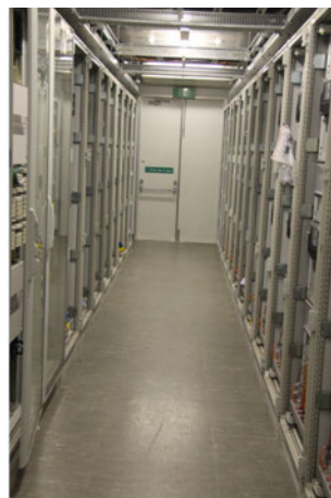
Inside of 132kV protection and control building
