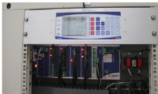
Transformer cooling control unit
