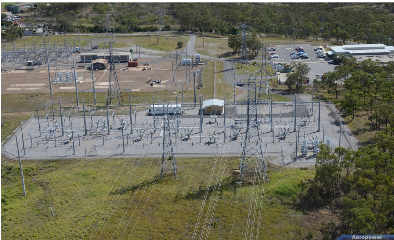
T152 and T019 Gladstone South Substations
