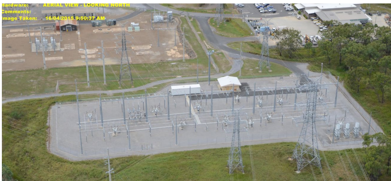
T152 and T019 Gladstone South substation yard bird view
