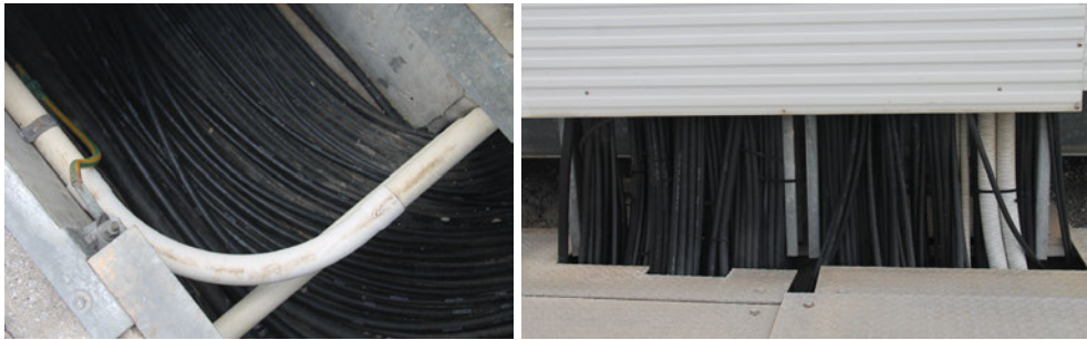
Control cables at T152
