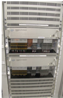
Power Quality Monitoring panel
