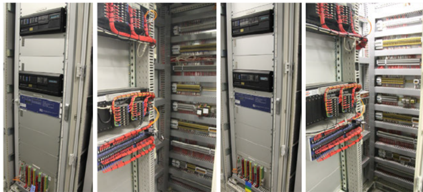
3 & 6 Transformer protection and control panels
