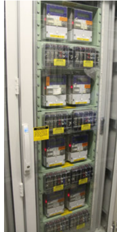
Metering devices for Feeder 7102, 7101, 7103 and 7147 at T152
