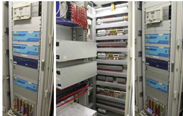
Feeder 7104 and 105 protection and control panels
