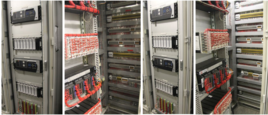
1 and 2 Bus zone protection and control panels
