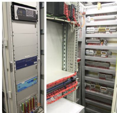
Feeder 7147 and 7169 protection and control panels
