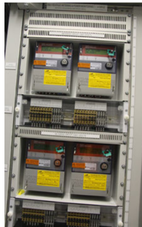
Metering panels for T3 and T6
