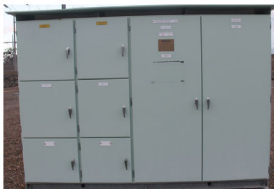
AC supplies and associated distribution boards
