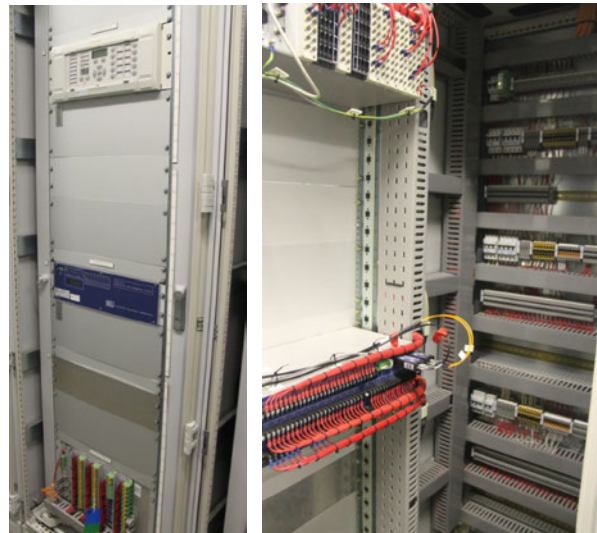
Feeder 760 protection and control panel
