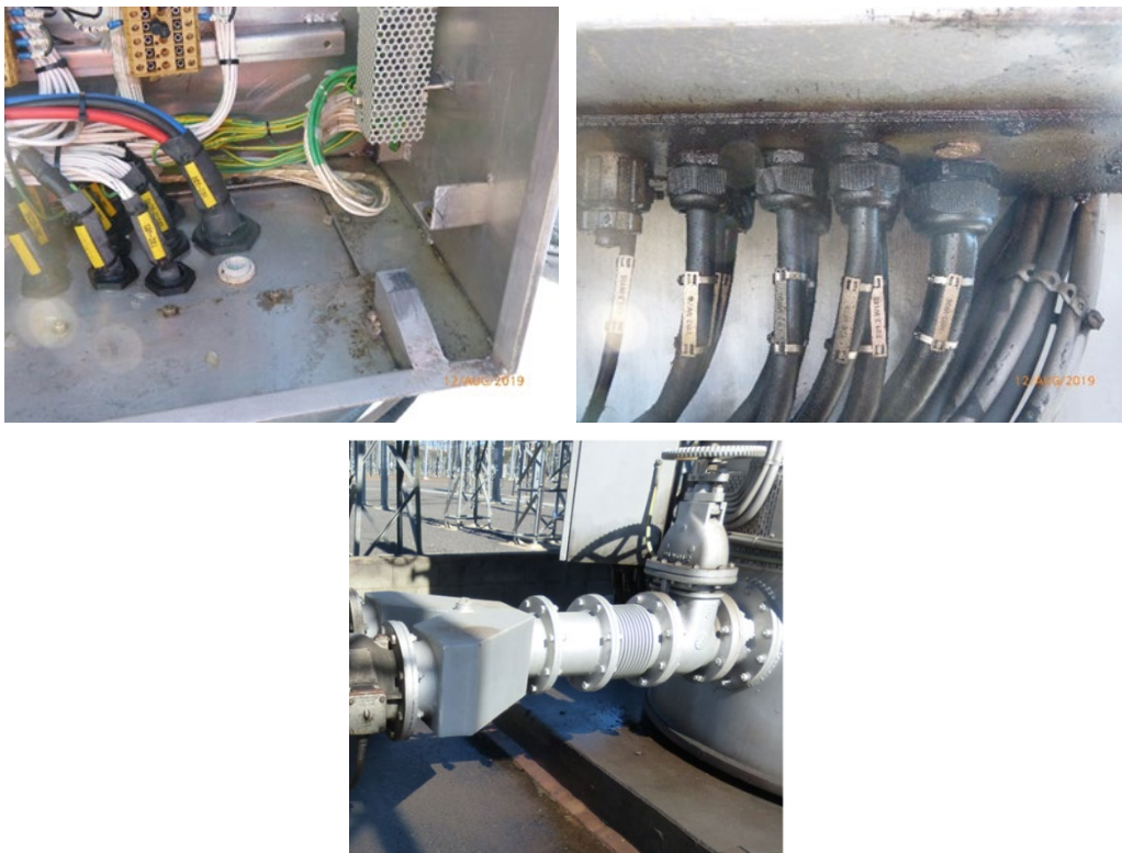
Figure 26- Oil through the cables and control box.
