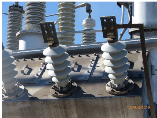
Figure 58 - Oil leaks from Terminal box on tertiary bushings
