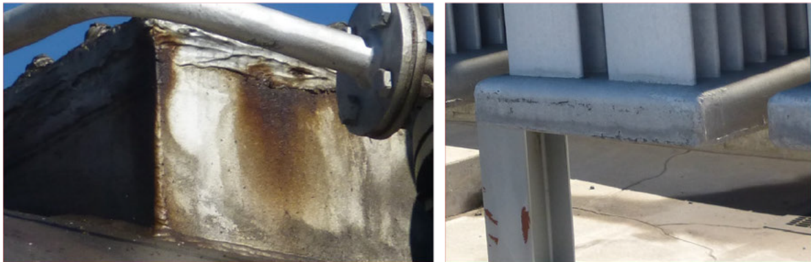
Figure 22 – Minor corrosion & galvanisation damage
