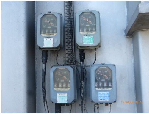
Figure 31 - HV WTI instrument, LV WTI instrument and OTI instrument. All the viewing windows are clear enabling easy instrument reading except the OTI.
