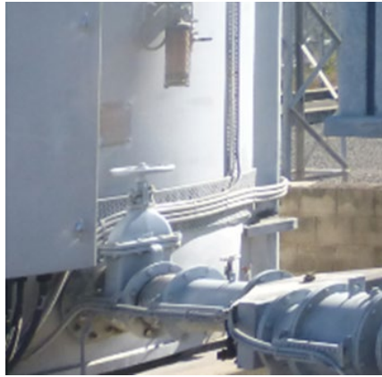
Figure 12- Multi-core cables attach to the Main tank
