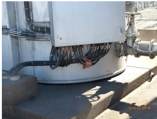
Figure 44- Multi-core cables attach to the Main tank
