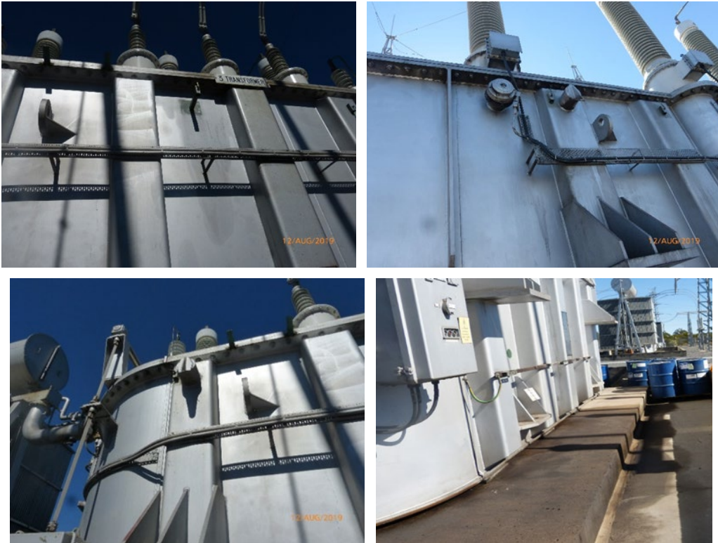
Figure 42- Oil film leaking from the top of main tank.
