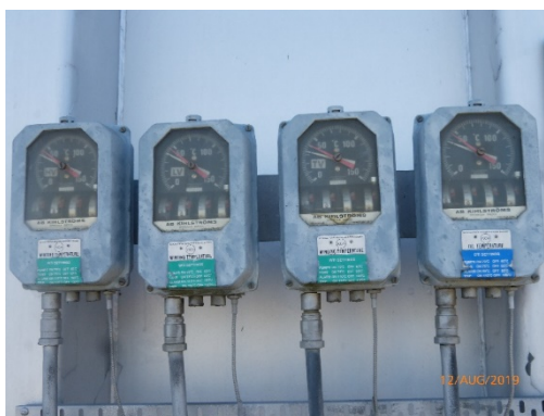
Figure 60 - HV WTI instrument, LV WTI instrument and OTI instrument. All the viewing windows are clear enabling easy instrument reading except the OTI
