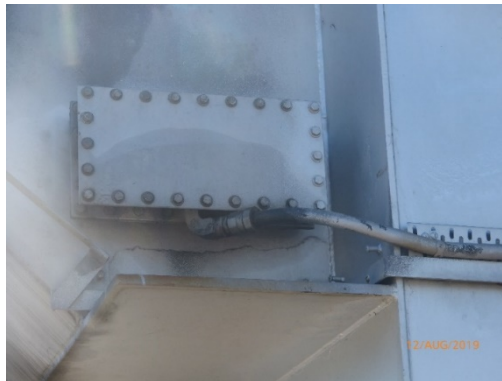
Figure 57- Oil leaks from Terminal box on tertiary bushings.
