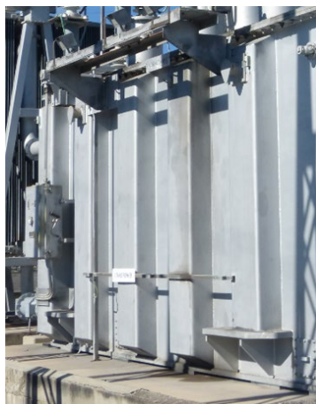
Figure 8- Oil film spreading to the bund from the main tank lid gasket.
