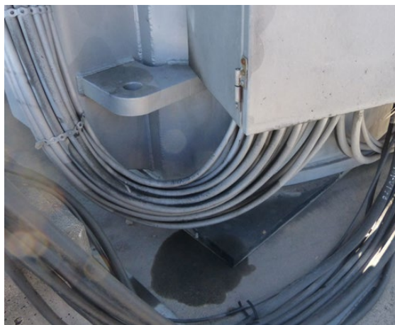
Figure 11 - Oil leaks from a radiator bank visible on the control cables located underneath
