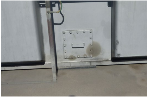
Figure 9- Oil leaks from the side wall hatch
