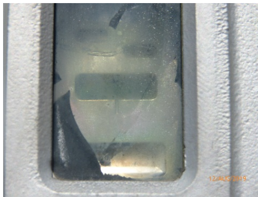
Figure 30- Tap changer sight glass
