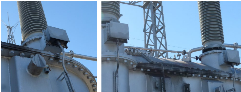
Figure 28- Oil leaking from HV bushing CT box
