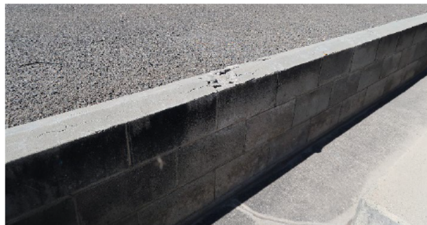
Figure 6 - H018 T1 bund condition.
