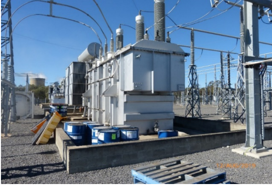
Figure 3 -70/90 MVA 275/66kV transformer T3 at H018 Tarong substation.
