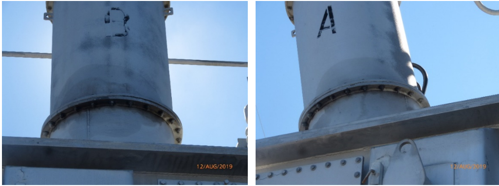
Figure 56 - Oil leaks from Bushing Turrets
