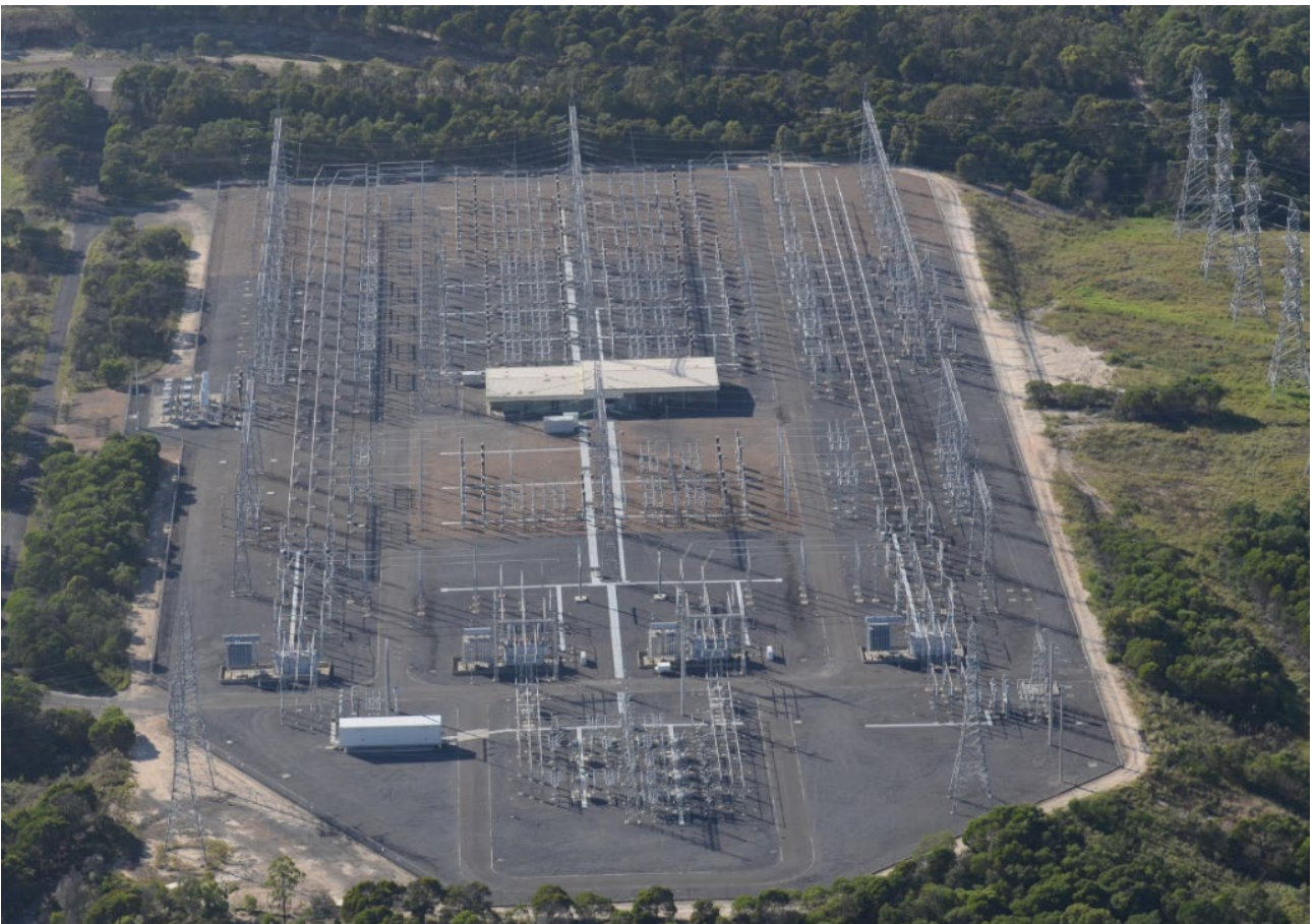
Figure 2: Aerial view of Tarong Substation
