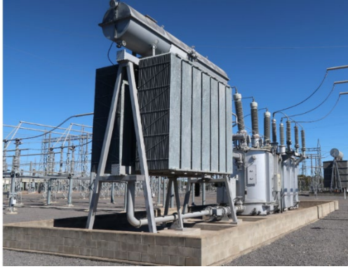
Figure 4 -70/90 MVA 275/132 kV transformer T4 at H018 Tarong substation
