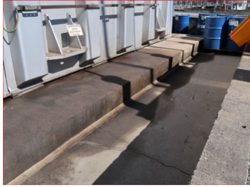
Figure 40 – Bund floor cracks
