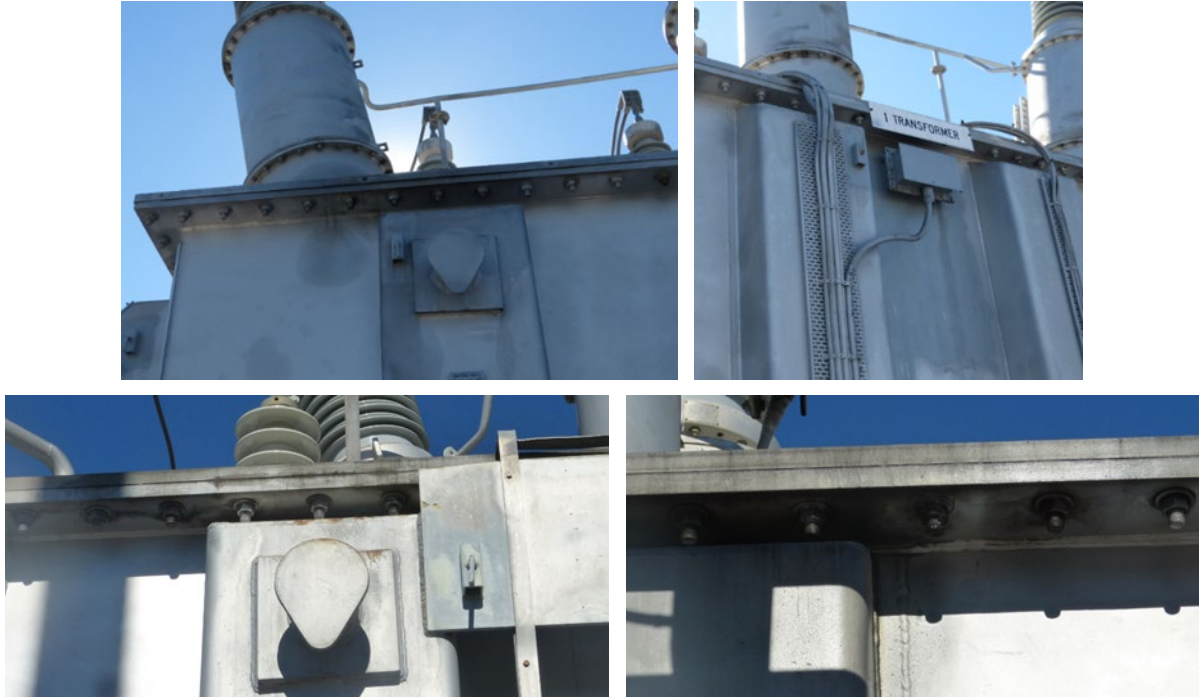
Figure 7. - Oil leaking from the main tank to lid gasket
