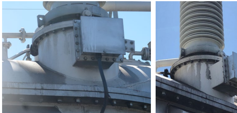
Figure 41 - Oil leaks from the A & C phase bushing turrets
