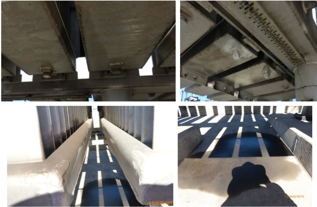
Figure 27- Oil leaks from the radiator banks
