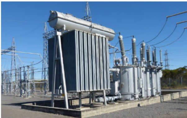
Figure 2 -70/90 MVA 275/132kV transformer T1 at H018 Tarong substation.
