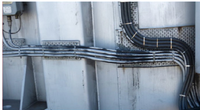
Figure 39 – paint on multicore cables.
