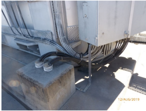
Figure 59- Multi-core cables attach to the Main tank
