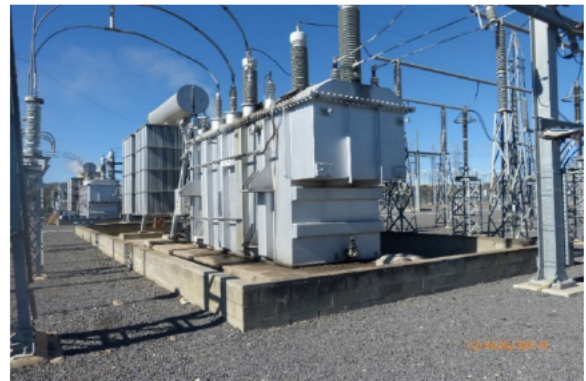
Figure 1-70/90 MVA 275/66kV transformer T2 at H018 Tarong substation
