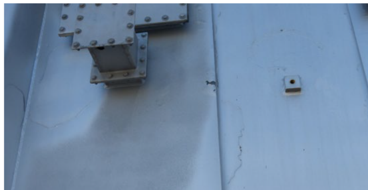
Figure 53- Flaking of paint
