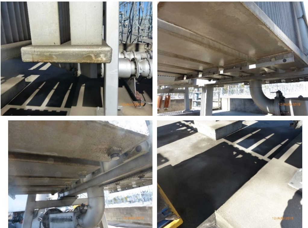
Figure 43- Oil leaks from radiator banks.
