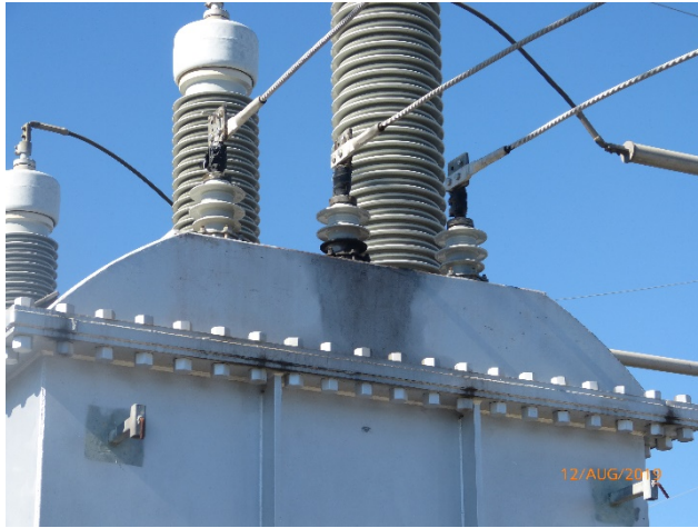
Figure 25- Oil film leaking from the TV bushing base.
