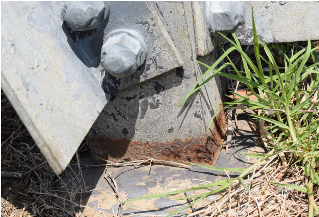
Figure 17: 1018-STR-3192 Interface Corrosion
