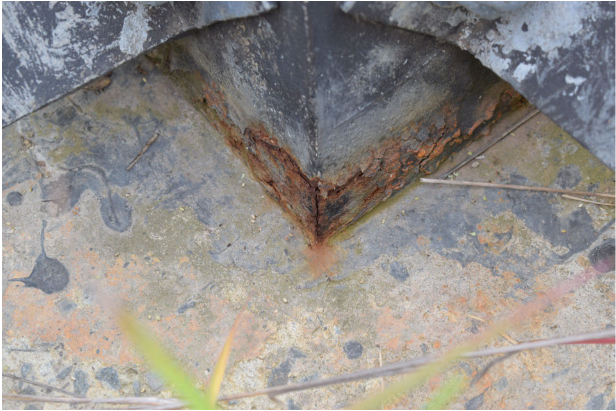
Figure 21: 1019-STR-3401 Interface Corrosion
