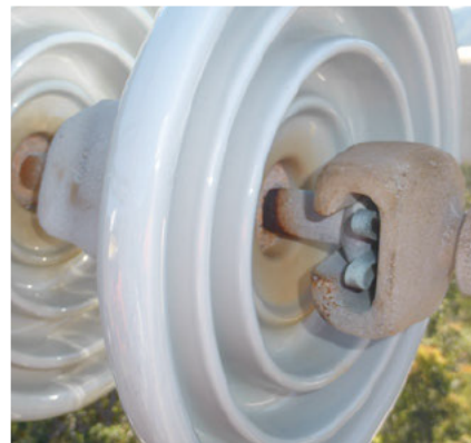
Figure 26: 1018-STR-3112 Tension Insulator Corrosion
