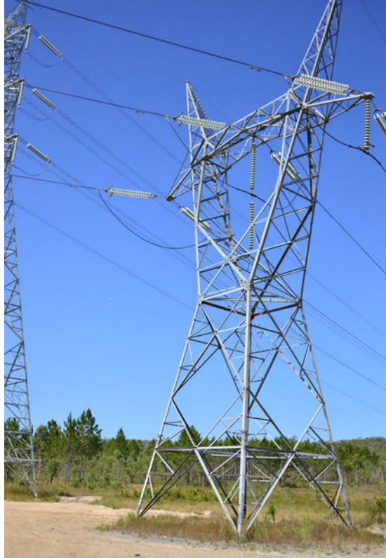
Figure 8: 1019-STR-3288 - Tension Tower
