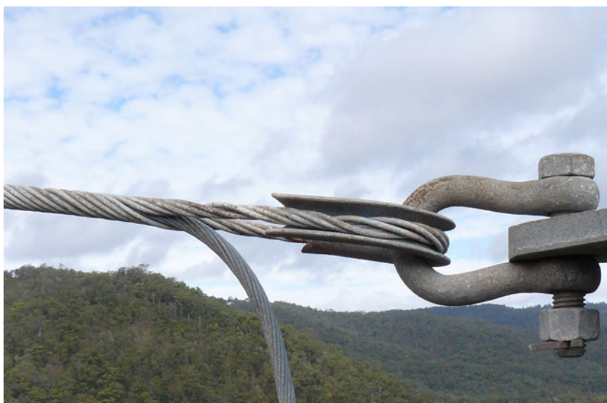
Figure 1: OHEW Hardware Corrosion
