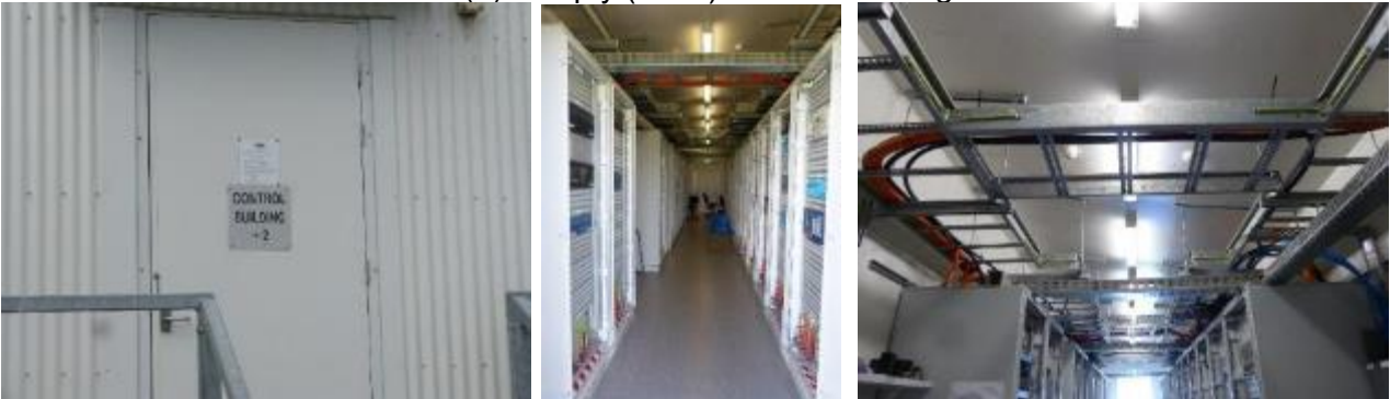
(b) 275kV Demountable Control Building +2
