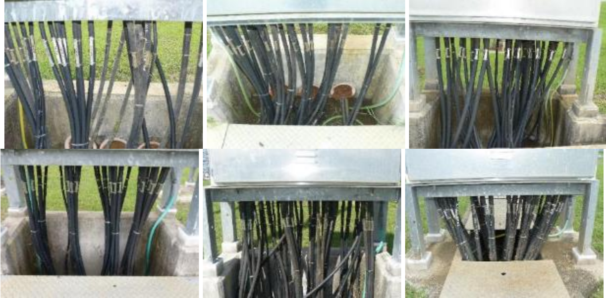
Figure 7 – Physical appearance of typical outdoor secondary system cables
