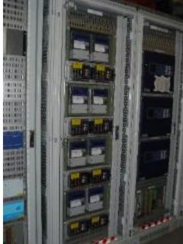
Figure 14 – Revenue Metering Panel
