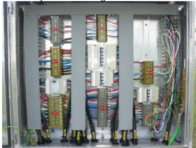
(f) =C04-A91 Bay AC Marshalling Kiosk
