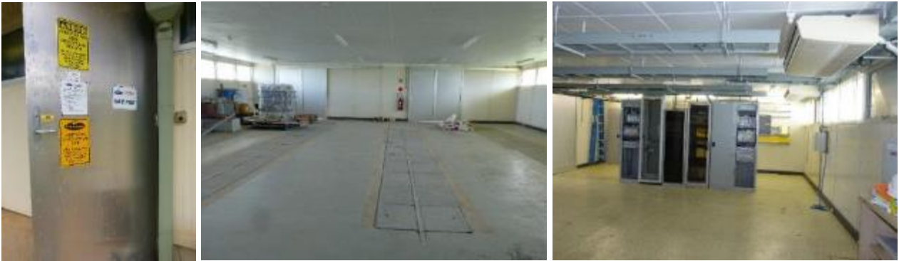
(a) Empty (Brick) Control Building +1
