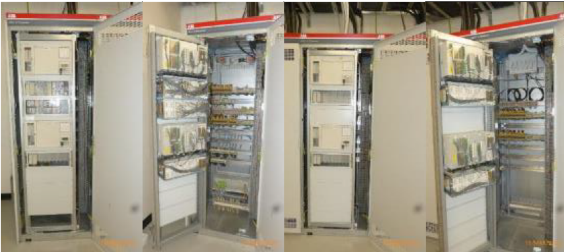
SVC X Protection Panels
