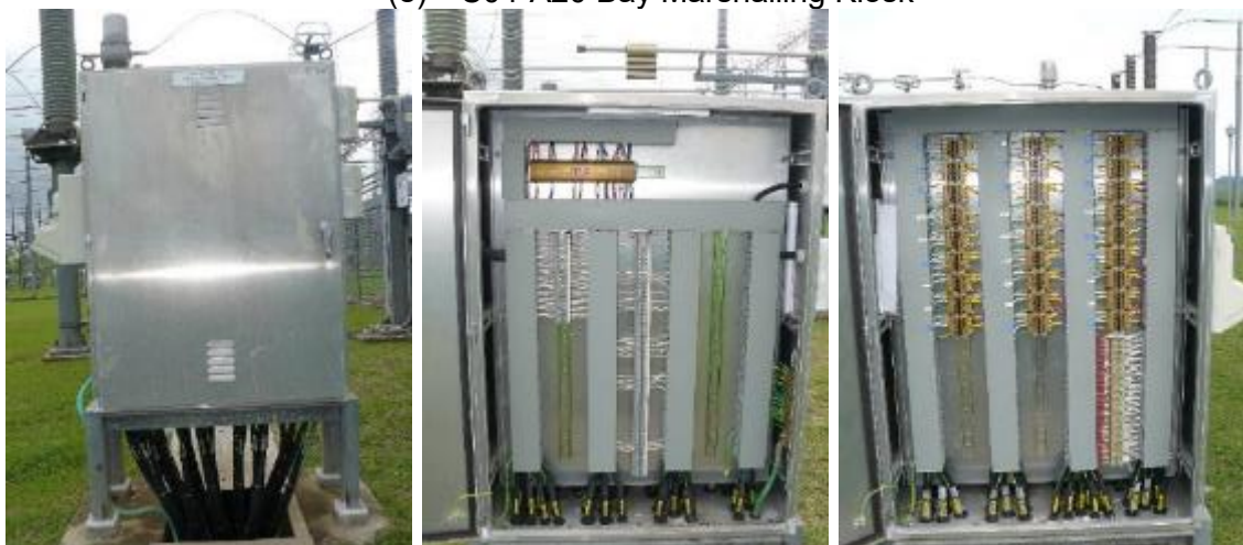
(f) =C06-A10 Bay Marshalling Kiosk
