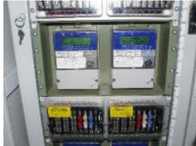
Figure 15 – Woollooga Substation and SVC Metering Equipment
