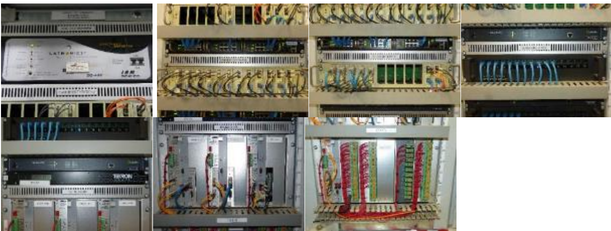
Figure 17 – Woollooga Substation and SVC OpsWAN Equipment
