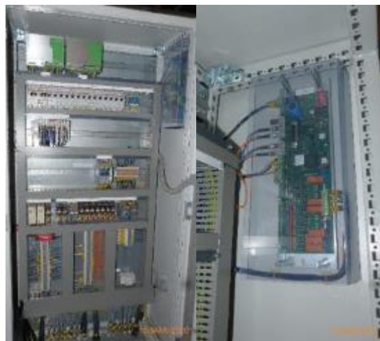
Figure 11 – SVC Cooling Control System Panel
