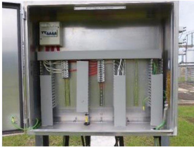
(a) =D07-A91 Bay AC Marshalling Kiosk
