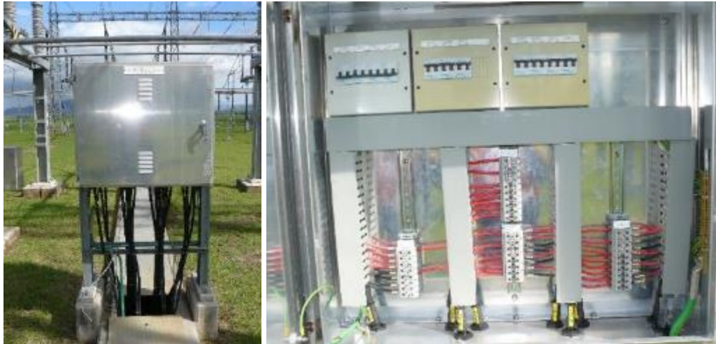
(g) =C04-A92 Bay DC Marshalling Kiosk
