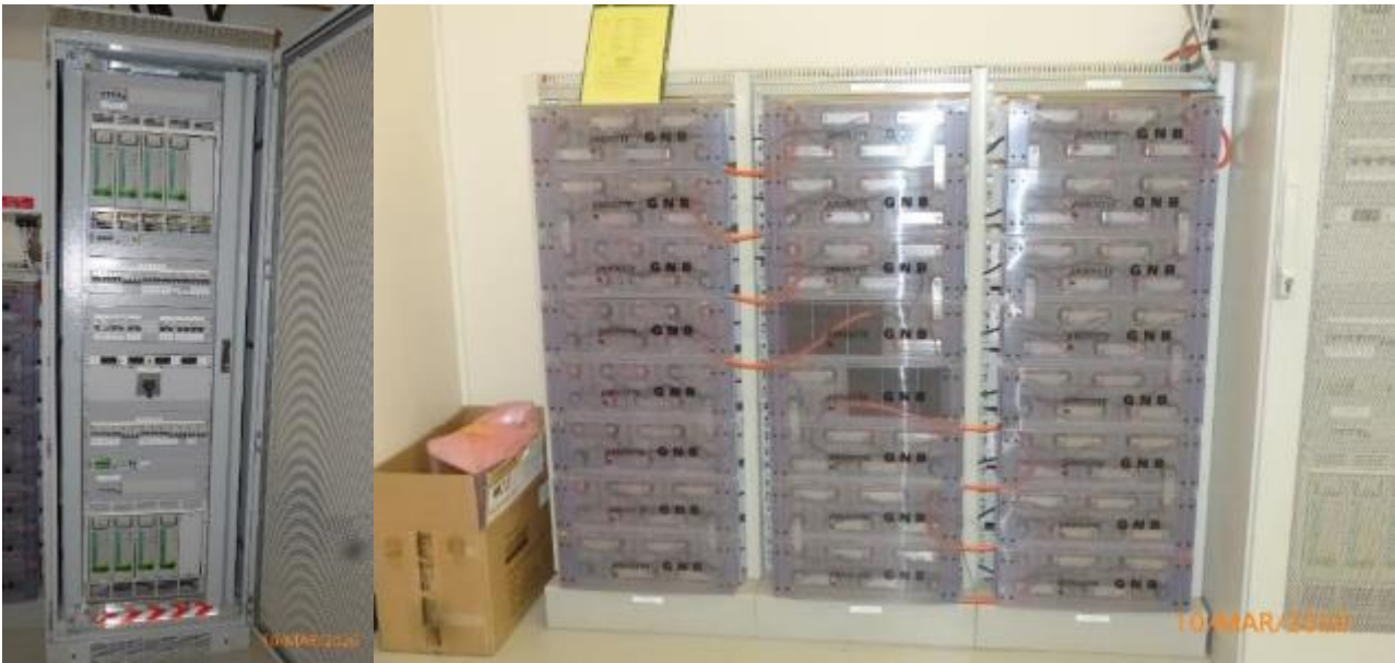
(Buildings +4 - SVC 125V X and Y DC Batteries and Chargers - 2008)
