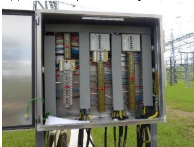
(b) =D07-A92 Bay DC Marshalling Kiosk
