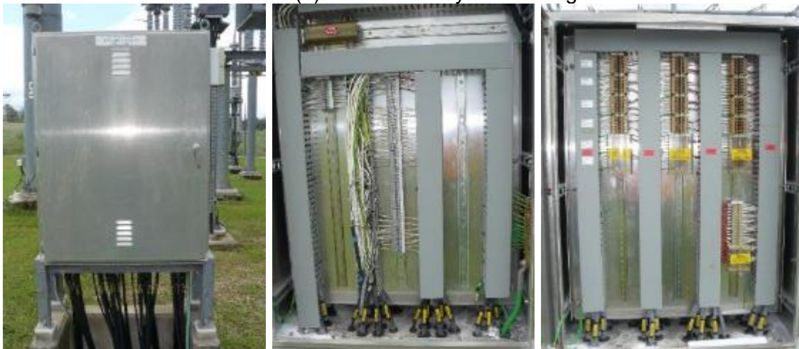
(c) =D18-A10 Bay Marshalling Kiosk
