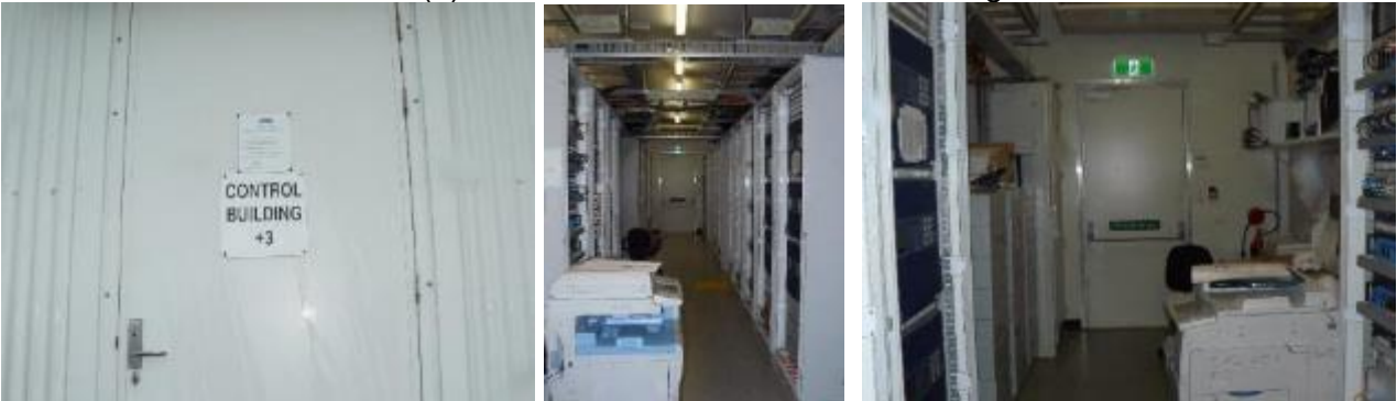
(c) 132kV Demountable Control Building +3
