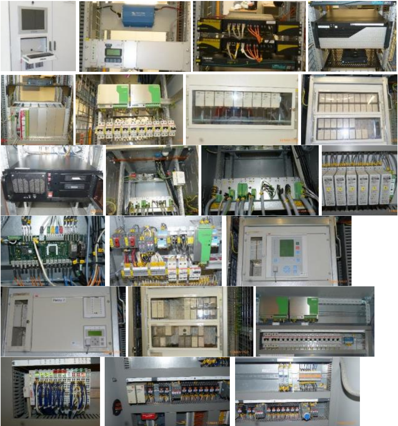
Figure 13 – Woollooga SVC Typical SVC Indoor Secondary System Equipment (2008)
