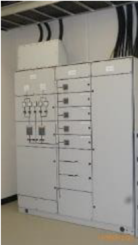
SVC 400V AC Auxiliary / Changeover Panel
