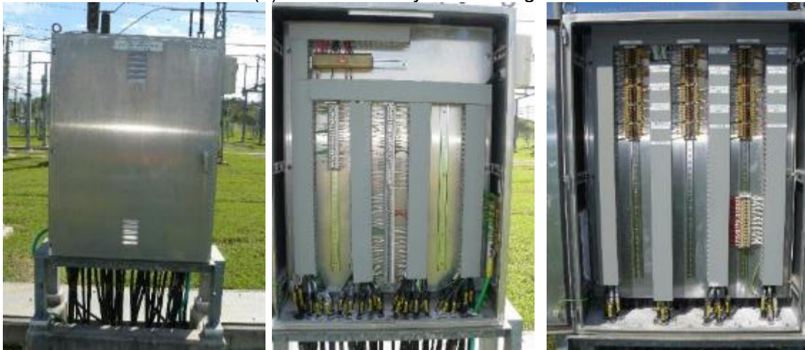
(e) =C04-A20 Bay Marshalling Kiosk
