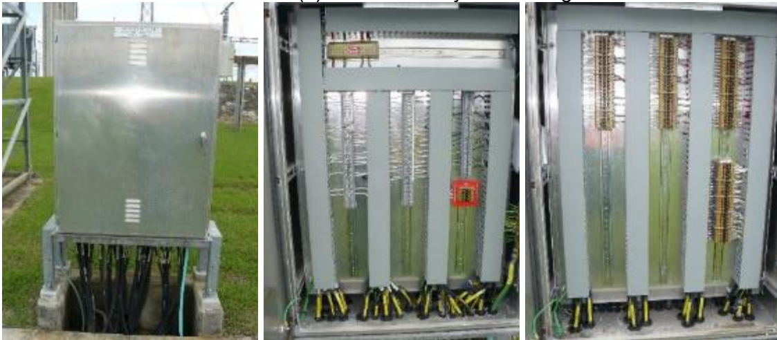
(b) =D11-A10 Bay Marshalling Kiosk
