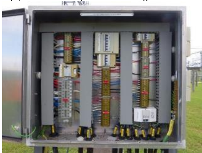
(c) =D15-A91 Bay AC Marshalling Kiosk
