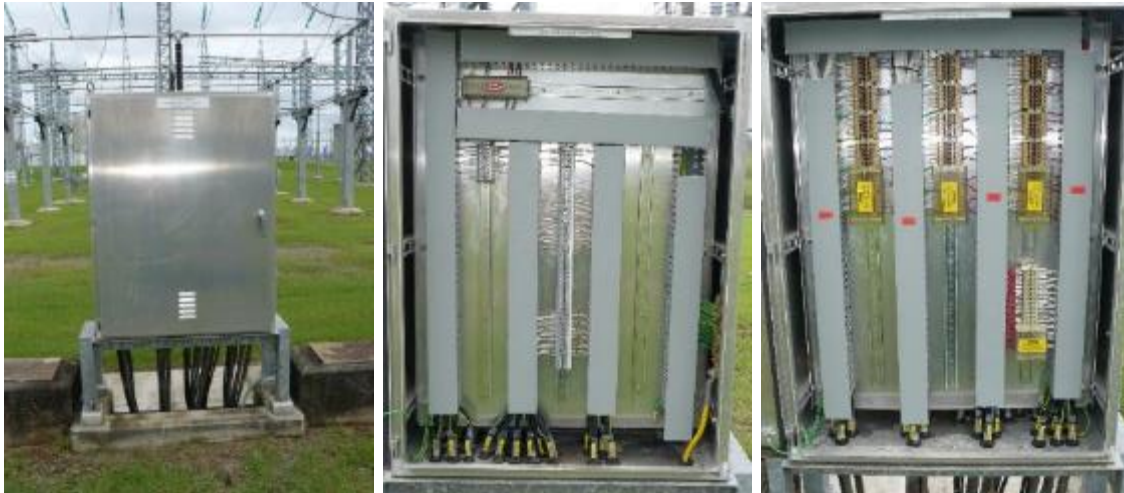
(a) =D03-A10 Bay Marshalling Kiosk
