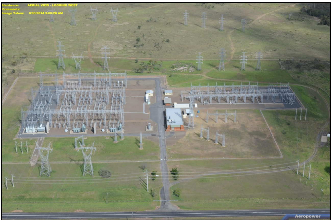
Figure 2: Aerial view of Bouldercombe Substation
