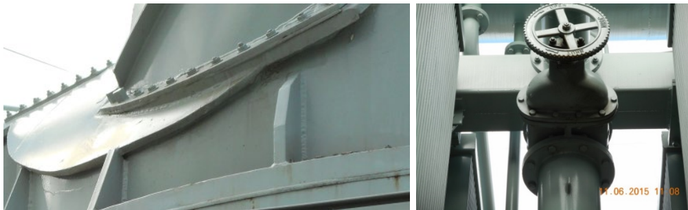
Figure 35: (LHS) 'C'-phase bushing turret to lid gasket oil leak. (RHS) Cooler bank top header gate valve oil leak.
