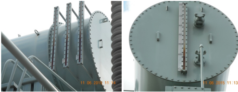
Figure 43: (LHS) Three separate oil level gauges and oil delivery pipes for each OLTC phase. (RHS) One oil level gauge on the end for the main tank oil.
