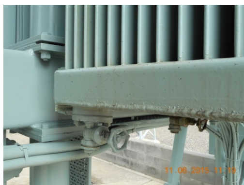
Figure 10: Typical oil leaks from where the oval tubes enter the headers. Note insects (black dots) stuck to the oil film on the side of the bottom header.
