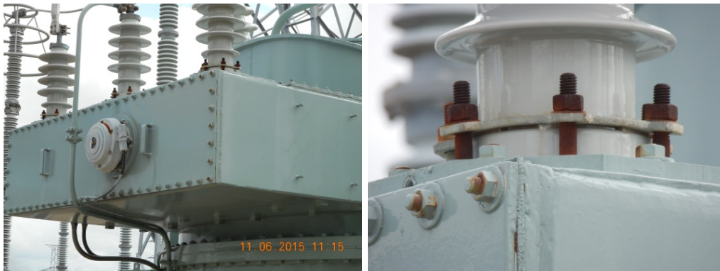
Figure 2: Corrosion of TV mounting bolts and pressure relief vent cover.
