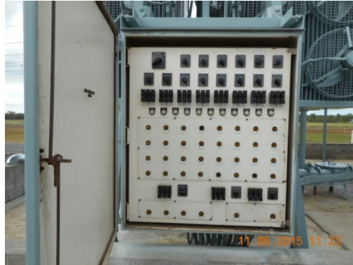
Figure 14: There were no issues noticed inside the Cooler Control Cubicle.
