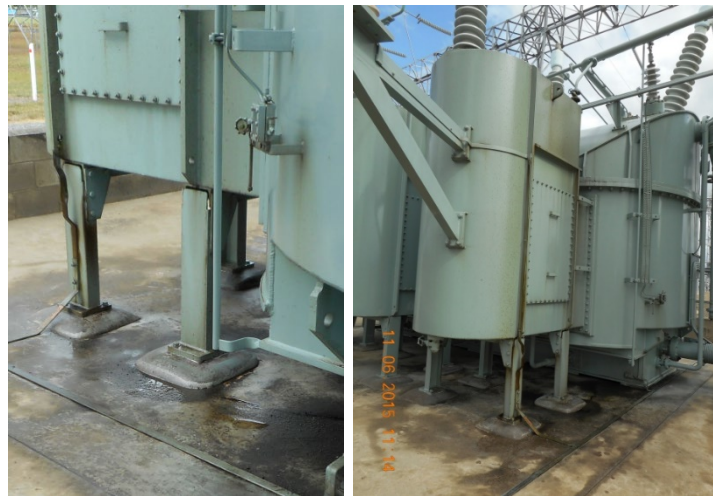
Figure 9: Typical oil leaks from the side mounted LV bushing & OLTC chambers. Note the free oil pooling on the ground.
