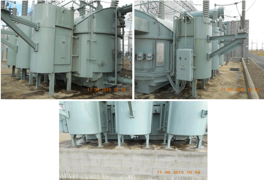
Figure 34: Typical oil leaks from the side mounted LV bushing & OLTC chambers. Note the free oil pooling on the ground.
