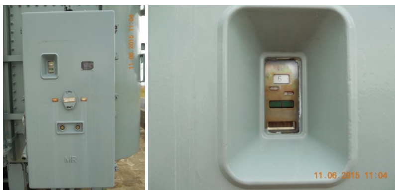
Figure 41: Reinhausen tap changer control cubicle for type 3 x M1 1200 150B 10193W.
