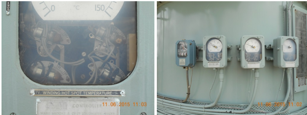
Figure 39: Mercury switches in the 2 WTI & 1 OTI instruments for cooling control and alarm and trip signalling.
