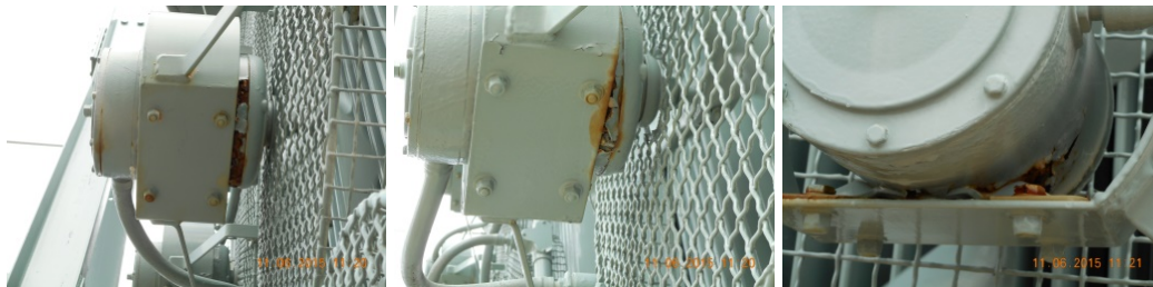
Figure 3: Advanced corrosion of cooler bank fan motor casings.
