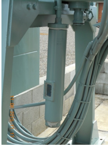
Figure 23: The conservator desiccant breather design does not allow comprehensive visual inspection for serviceability.
