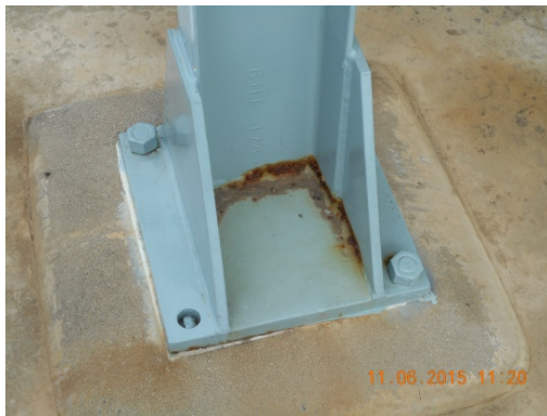
Figure 5: Corrosion of the cooler bank 'A'-frame support structure mounting feet welds.
