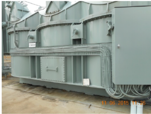
Figure 11: The UV stabilisers in the paint covering the external multicore cables will assist in preserving the outer PVC covering.
