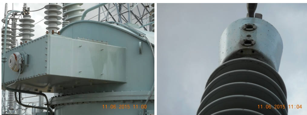
Figure 33: (LHS) Oil leak from the hatch gasket on top of the TV bushing CT chamber. (RHS) HV 'B'-phase bushing oil level indicator oil leak.
