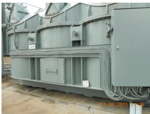
Figure 6: No welded lid to main tank but no corrosion visible between mating steel flanges which sandwich the gasket.
