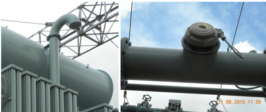
Figure 42: The explosion vent (rupture diaphragm) at the end of a high rise pipe as well as a PRD on the top main oil pipe between cooler bank and transformer main tank.
