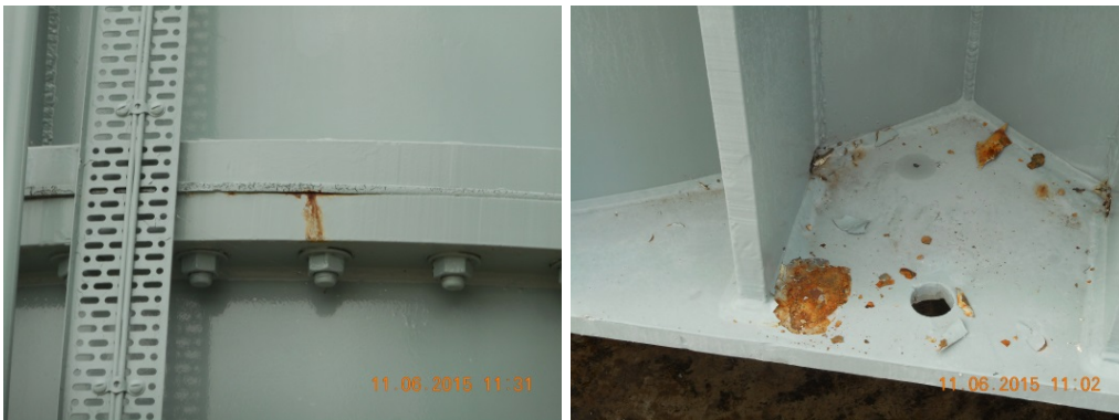
Figure 30: (LHS) Corrosion between the main tank and lid mating steel flanges. (RHS) Corrosion on a horizontal main tank stiffener plate.
