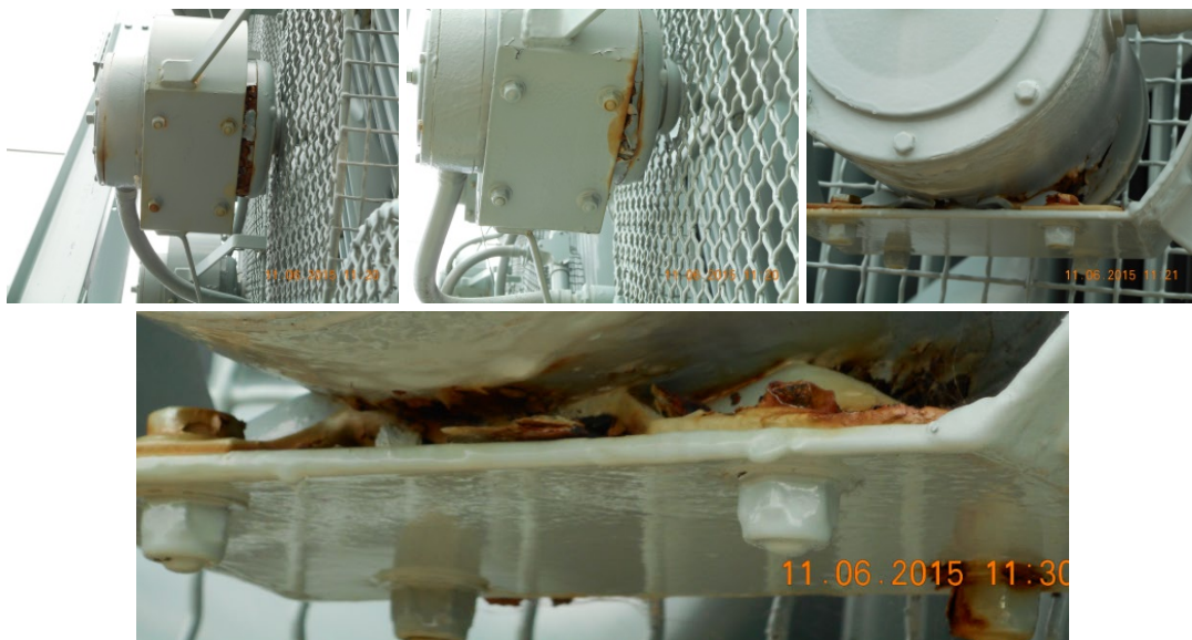
Figure 27: Advanced corrosion of cooler bank fan motor casings.
