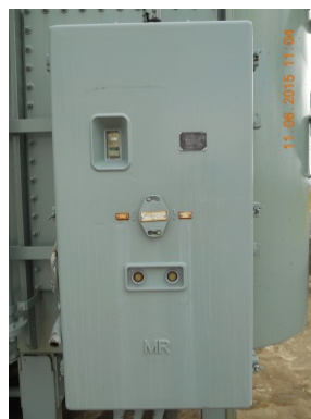
Figure 15: Reinhausen tap changer control cubicle for type 3 x M1 1200 150B 10193W.
