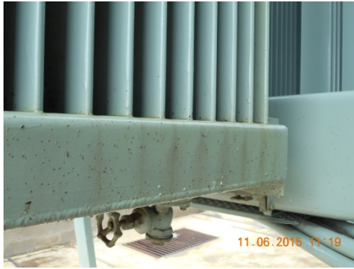
Figure 4: Corrosion of cooler bank radiator panels where the oval tubes enter the headers causing oil leaks. Note insects (black dots) stuck to the oil film on the side of the bottom header.
