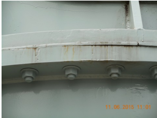
Figure 32: No welded lid to main tank but corrosion is visible in some locations as well as oil leaks.
