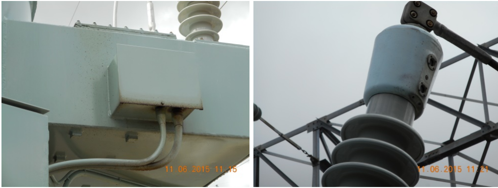
Figure 8: (LHS) Oil leak from the hatch gasket on top of the TV bushing CT chamber. (RHS) HV 'A'-phase bushing oil level indicator oil leak.
