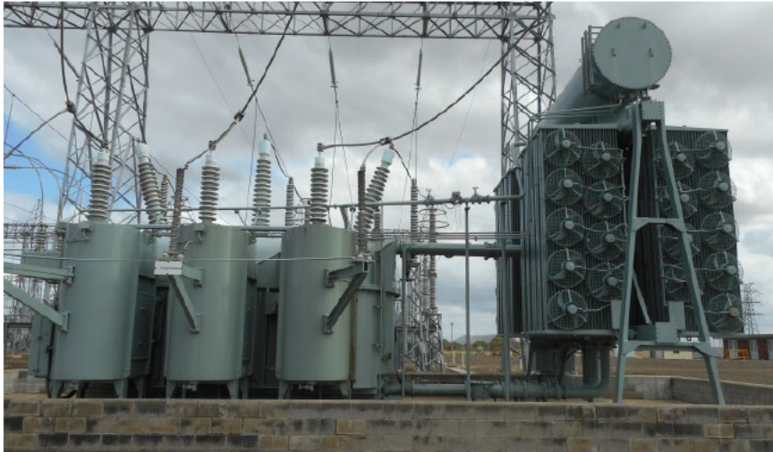
Figure 1: 200MVA 288/138/19.1kV transformer T1 at H010 Bouldercombe.
