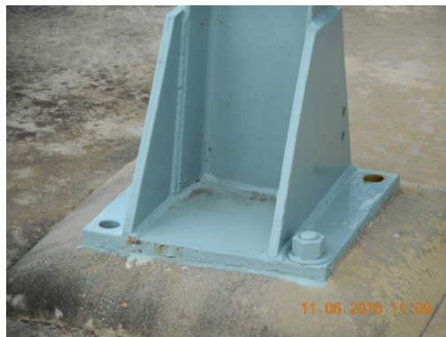
Figure 31: Corrosion occurring beneath the paint of the cooler bank 'A'-frame support structure mounting feet.
