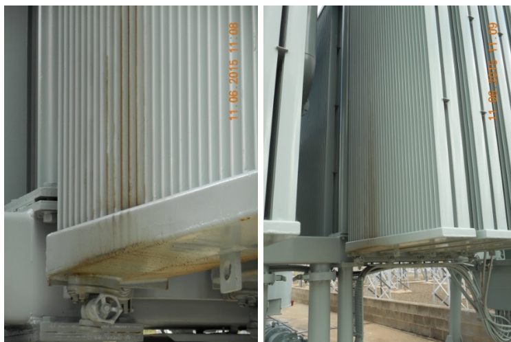
Figure 36: Typical oil leaks from where the oval tubes enter the headers.
