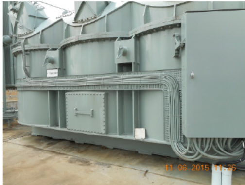
Figure 37: The UV stabilisers in the paint covering the external multicore cables will assist in preserving the outer PVC covering.
