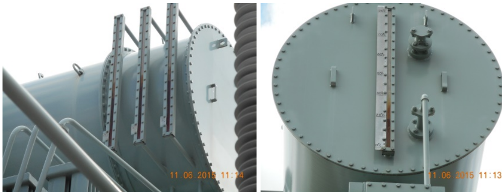
Figure 17: (LHS) Three separate oil level gauges and oil delivery pipes for each OLTC phase. (RHS) One oil level gauge on the end for the main tank oil.
