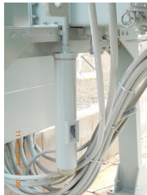
Figure 49: The conservator desiccant breather design does not allow comprehensive visual inspection for serviceability.
