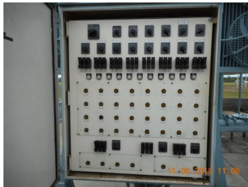
Figure 40: There were no issues noticed inside the Cooler Control Cubicle.
