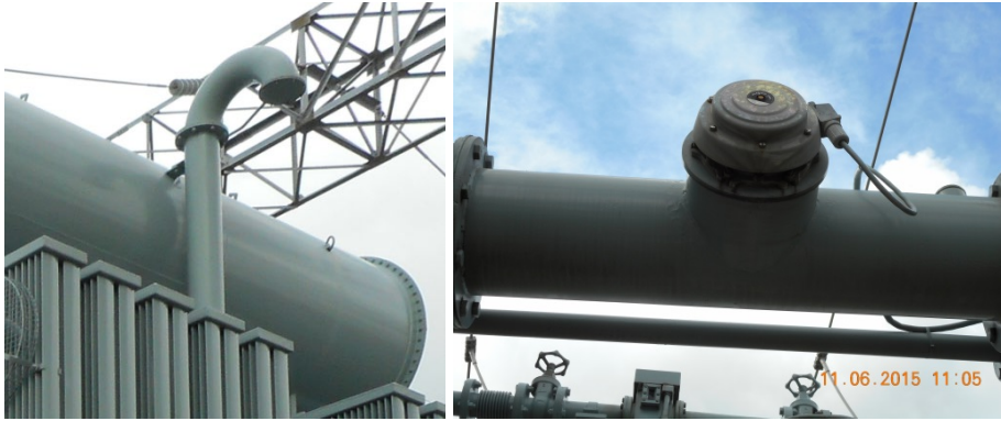
Figure 16: The explosion vent (rupture diaphragm) at the end of a high rise pipe as well as a PRD on the top main oil pipe between cooler bank and transformer main tank.
