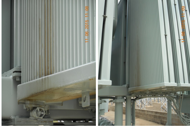
Figure 28: Corrosion of cooler bank radiator panels where the oval tubes enter the headers causing oil leaks.
