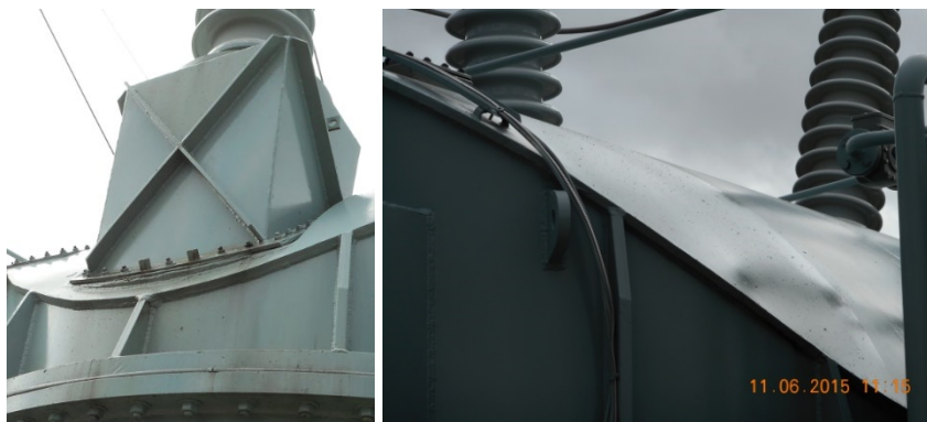
Figure 7: (LHS) Oil leak from the HV 'B'-phase bushing mounting flange gasket to turret. (RHS) Oil leaks from gaskets further up on lid.
