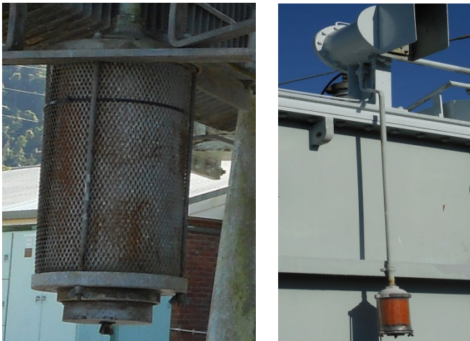
Figure 10: Main tank conservator breather showing concealed oil bath and the separate VT conservator and breather
