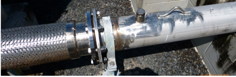
Figure 6: Main oil pipework installed in 2008.
