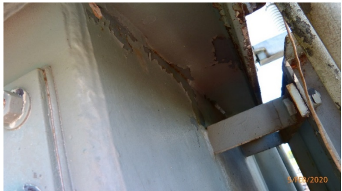
Figure 1: Transformer LV side of the main tank showing the oxidised repainted surfaces
