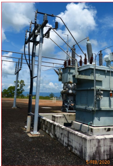
Figure 21 – Insulated cables connection to T2
