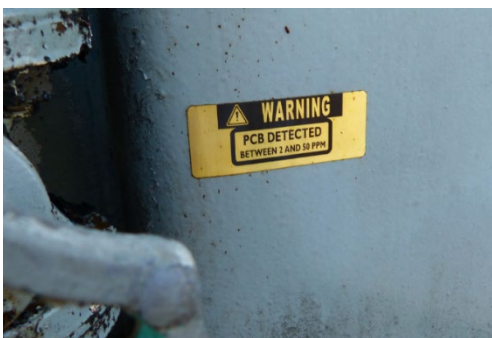
Figure 8: Signage for PCB contamination
