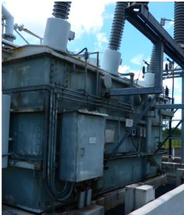
Figure 2: Transformer T2 HV side of the main tank showing paint oxidation
