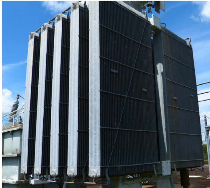
Figure 7: Cooler bank on the transformer
