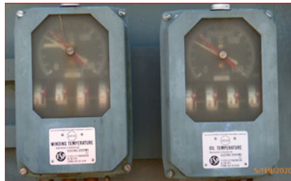
Figure 25 – Temperature Indicators (OTI and WTI)
