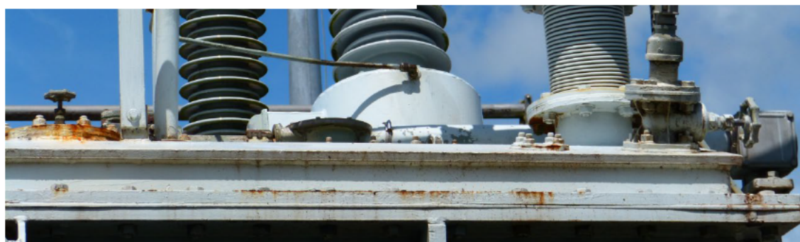
Figure 5: Corrosion on the top of the tank
