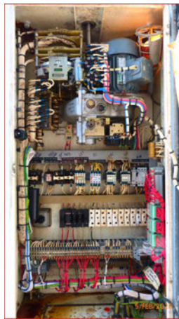
Figure 24:OLTC Control Cubicle
