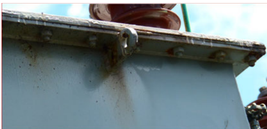
Figure 9: Minor oil leak
