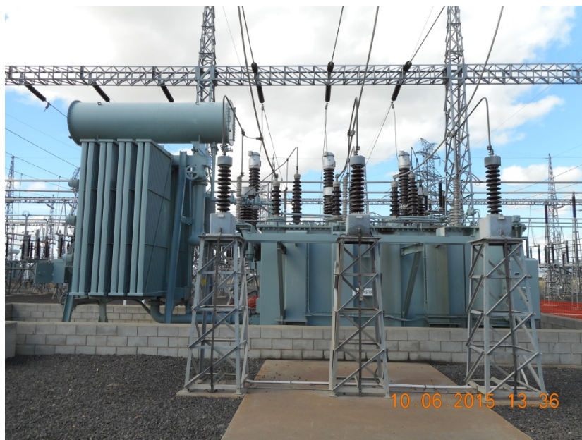
Figure 2 T032 transformer T2 from the LV side.
