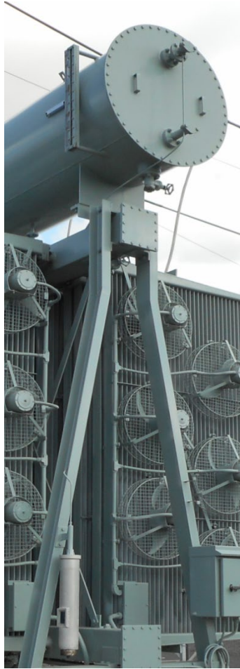
Figure 15 The original Drycol refrigerant breather removed from the conservator and a new, small breather pipe installed to connect to the home-made desiccant breather.
