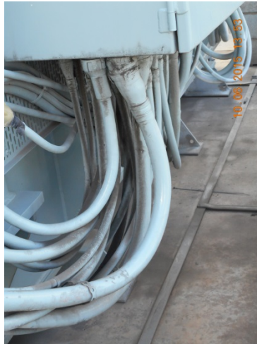
Figure 11 Painted multicore cables entering the main control cubicle.
