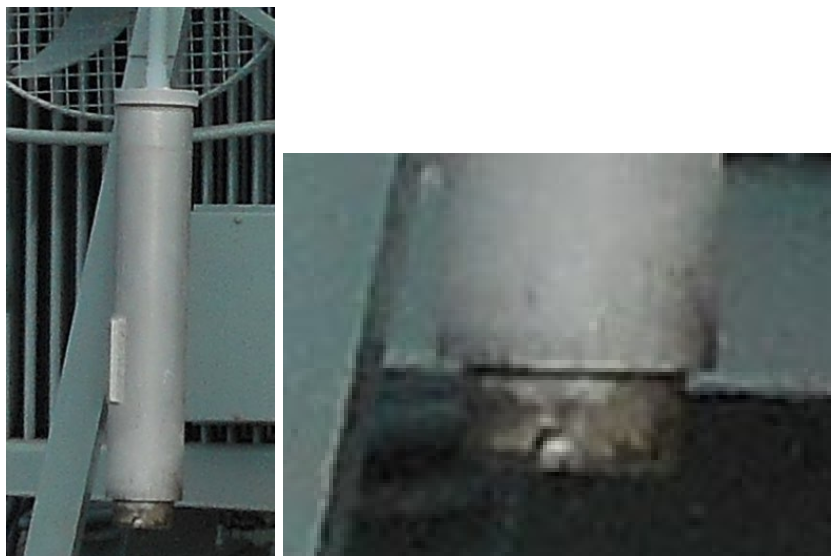
Figure 17 The “home made” main conservator desiccant breather and oil bath.
