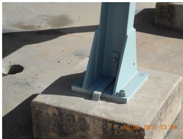
Figure 3 No visible corrosion evident around the cooler bank ‘A’-frame support structure feet.
