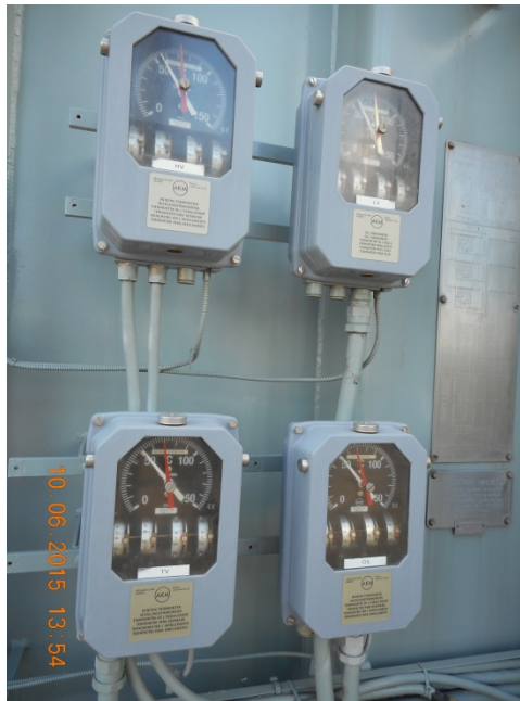
Figure 13 The three winding hot spot and one top oil temperature indicators are still readable through the viewing window.
