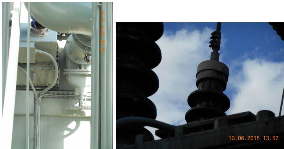
Figure 5 (LHS) Oil leaks from TV turret box gasket. (RHS) Oil leak at top cap of HV 'B' phase bushing
