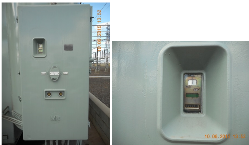
Figure 12 Reinhausen OLTC with a counter reading of 94,330 operations.
