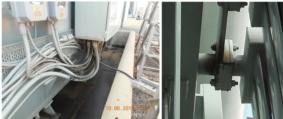
Figure 30 (LHS) HV side free oil on concrete. Appears to be coming from 'A' & 'B' phase HV bushing top cap oil leaks combined with oil from the multicore cables. (RHS) Oil dripping from top header radiator panel mounting gasket.
