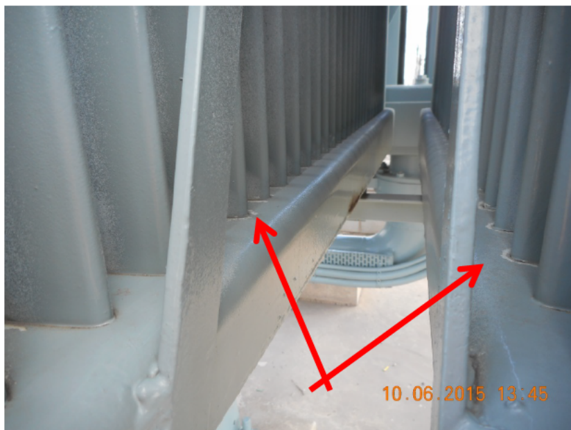
Figure 25 Residual localised corrosion where the radiator panel oval cooling tubes penetrate the bottom headers is re-emerging through the new paint.
