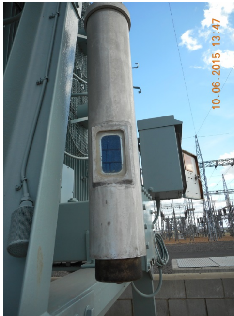
Figure 39 The “home made” main conservator desiccant breather and oil bath.
