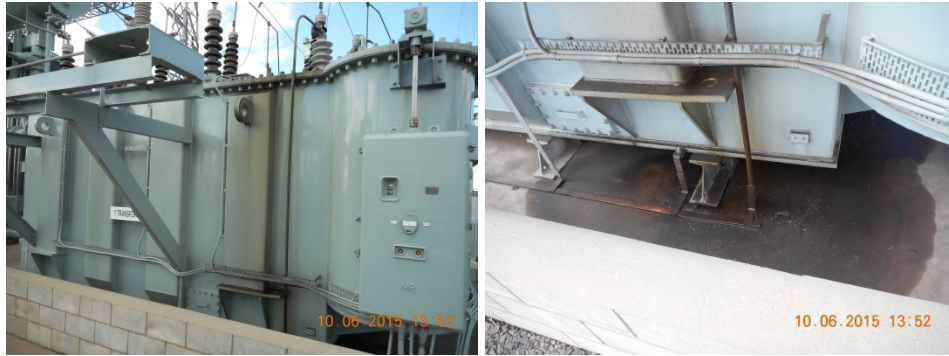
Figure 6 (LHS) Oil leak from neutral bushing mounting gasket. (RHS) Free oil pooling on concrete due to neutral bushing mounting gasket oil leak.
