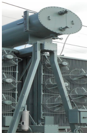
Figure 38 The original Drycol refrigerant breather removed from the conservator and a new, small breather pipe installed to connect to the home-made desiccant breather.
