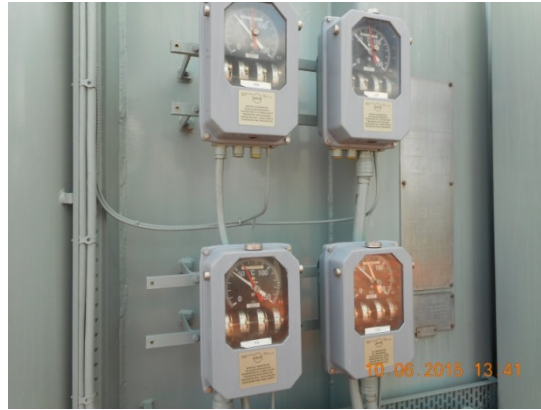
Figure 36 The three winding hot spot and one top oil temperature indicators are still readable through the viewing window.
