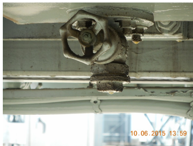
Figure 10 Oil leak from radiator panel drain valves fitted to the underside of the bottom header.
