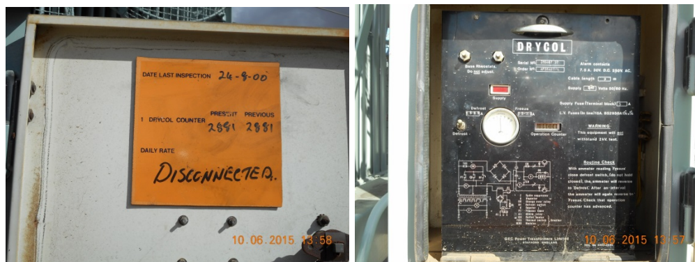
Figure 14 The original Drycol refrigerant breather (now removed) control cubicle still mounted on the cooler bank support frame.
