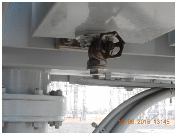
Figure 33 Oil leak from radiator panel drain valves fitted to the underside of the bottom header.
