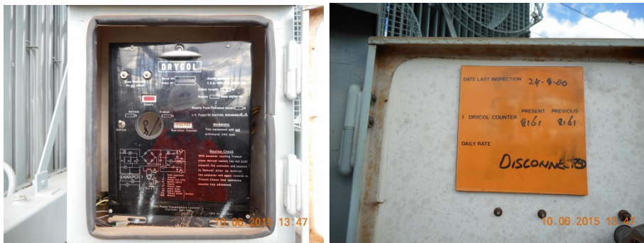
Figure 37 The original Drycol refrigerant breather (now removed) control cubicle still mounted on the cooler bank support frame.
