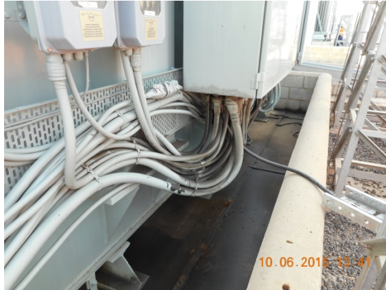
Figure 34 Painted multicore cables entering the main control cubicle.
