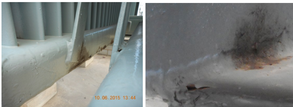
Figure 32 (LHS) Oil leak from radiator panel cooling tube to bottom header joint. (RHS) Another radiator panel oil leak on the lower shoulder weld seam of the bottom header. Note also the delaminating paint.
