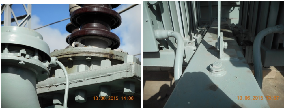
Figure 7 (LHS) HV 'B'-Phase top cap oil leak. (RHS) Oil dropping on bottom header from top radiator panel mounting gaskets.
