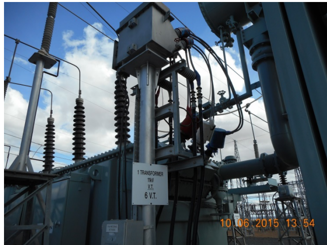
Figure 16 The TV connections for supplying the station services transformer (not in this picture) and Ergon 11kV load. The metering VT is visible on the steel post structure.
