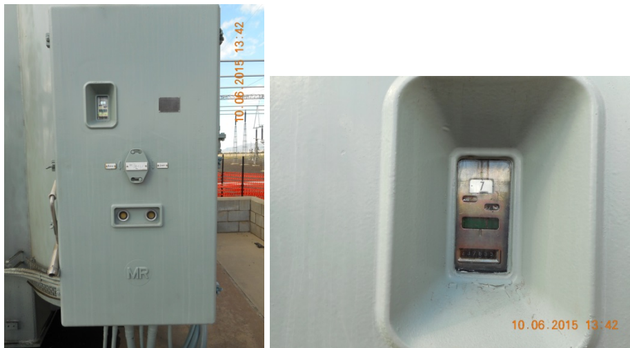
Figure 35 Reinhausen OLTC with a counter reading of 94,330 operations.
