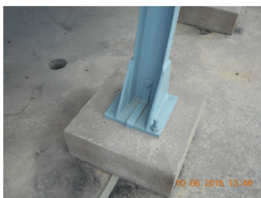
Figure 26 No visible corrosion evident around the cooler bank ‘A’-frame support structure feet.
