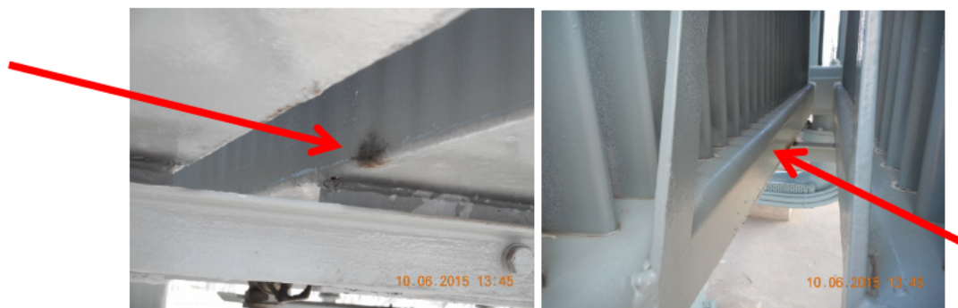
Figure 24 Localised corrosion on the shoulder weld of radiator panel bottom headers now showing a pin hole oil leak.
