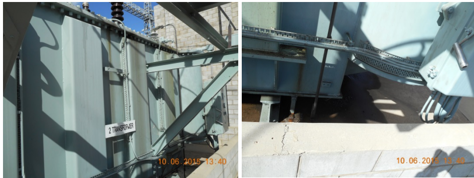
Figure 29 (LHS) Oil leak from neutral bushing mounting gasket. (RHS) Free oil pooling on concrete due to neutral bushing mounting gasket oil leak.
