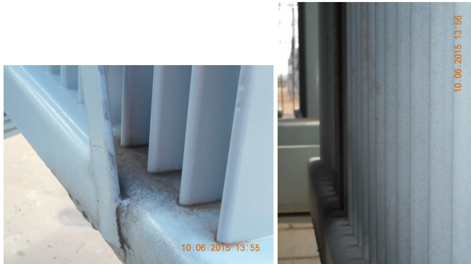
Figure 9 (LHS) Oil leak from radiator panel cooling tube to bottom header joint. (RHS) Another similar oil leak between cooling tube to bottom header.
