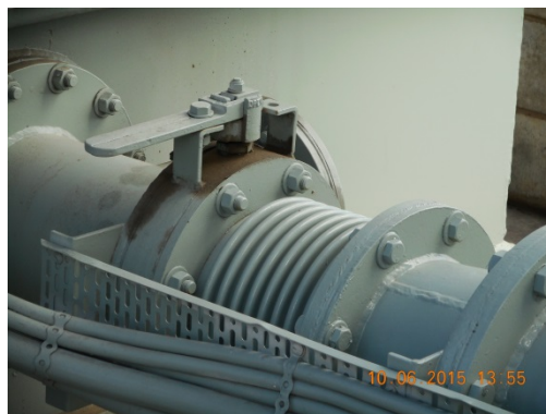
Figure 8 (LHS) Oil leak from bottom main butterfly valve (not gate valve) adjacent to main tank
