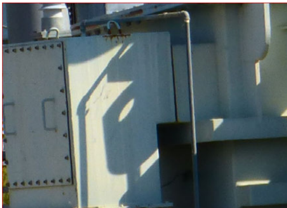
Figure 2- Transformer coating condition
