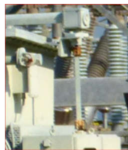
Figure 33 – Tap Changer Drive Shaft Coupling (2019)
