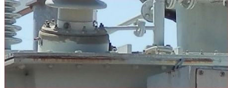
Figure 11 – Tank Lid Corrosion
