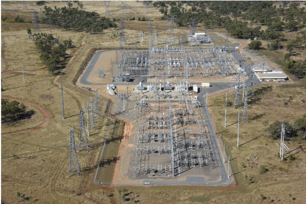
Figure 1: Aerial view of H11 Nebo Substation
