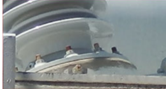
Figure 10 - Minor Bolt Corrosion
