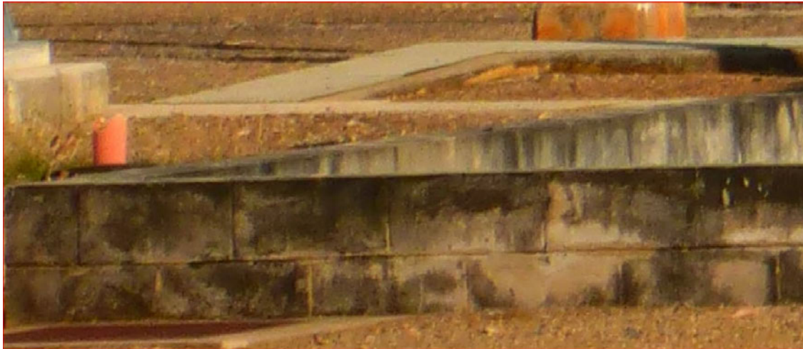
Figure 40 –Transformer 4 Bund Wall
