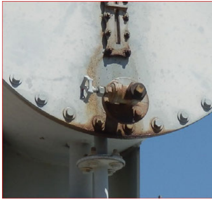
Figure 13 –Minor Oil Leak
