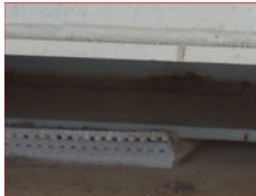
Figure 9—Tank Base Condition
