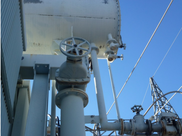
Figure 19: Small localised corrosion on cooler bank fittings.
