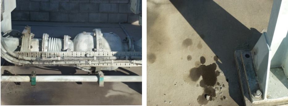
Figure 36: (LH) Oil leak from the lower main butterfly isolating valve adjacent to the main tank, and (RH) from OLTC conservator breather oil bath.
