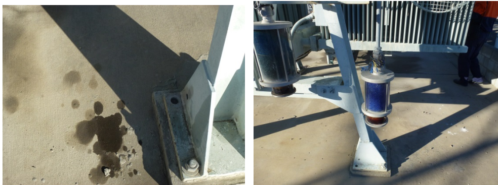
Figure 33: Cooler bank 'A' Frame structure using only two bolts per foot pad. No visible corrosion
