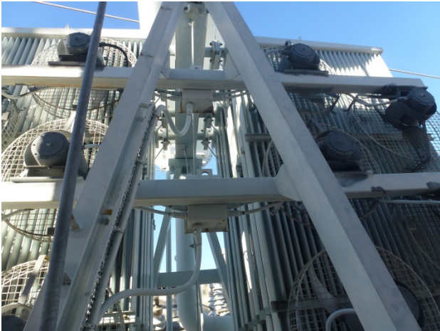
Figure 21: Small localised corrosion on cooler bank fittings.
