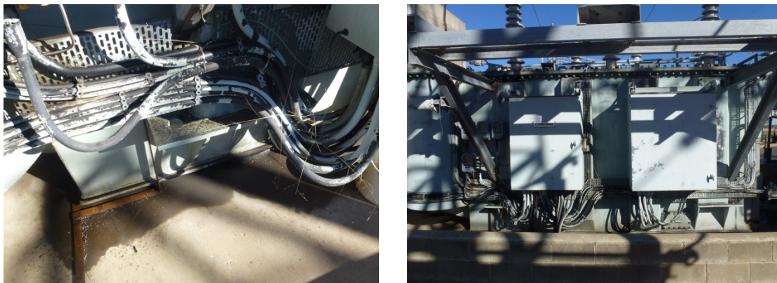
Figure 11: External cabling showing no signs of surface cracking but would have taken a set and should not be subjected to any significant flexing.
