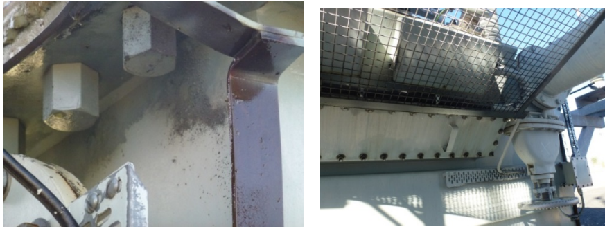
Figure 23: (LH) Oil leaks coming from gaskets on top of the main tank lid were dripping from the flange bolts. (RH) Oil leaks coming from the bolts which hold the cover plate for TV bushing connection access.
