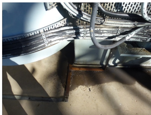
Figure 8: Oil leaks resulting in free oil collecting on the concrete around the main tank on the HV side.
