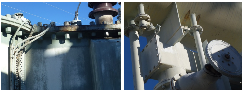
Figure 31: (LH) Corrosion of welded tank/lid strap. (RH) Corrosion on the bottom of the conservator appears like two holes forming.
