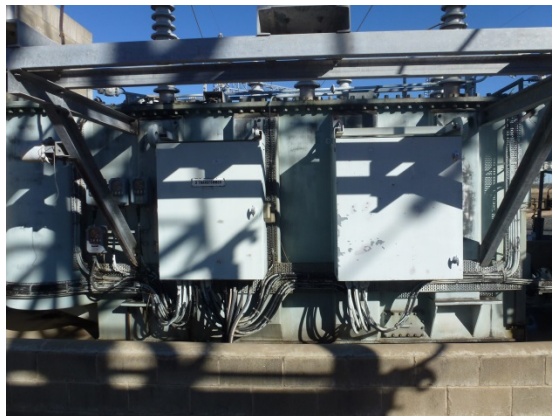
Figure 3: Transformer T3 HV side of the main tank showing paint delaminating off the cubicle doors.
