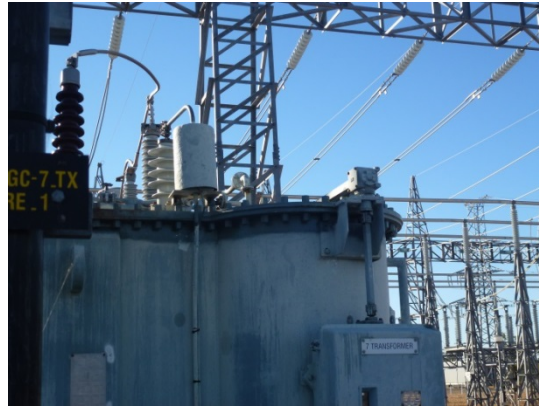
Figure 29: The dark strip around the tank / lid flange area is cold galvanising paint to combat the local corrosion.
