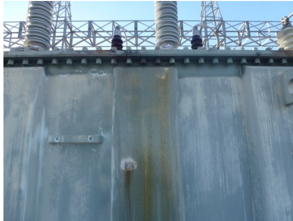
Figure 34: Oil run noticed on the LV side of the transformer main tank.
