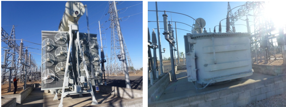
Figure 35: Relatively few oil leaks noticed on the concrete foundation.
