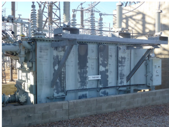
Figure 15: Transformer T4 LV side of the main tank showing the oxidised repainted surfaces.
