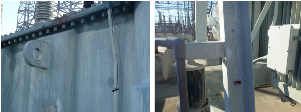
Figure 28: (LH) Transformer T7 LV side of the main tank showing the oxidised repainted surfaces. (RH) Surface paint cracking on the cooler bank support structure.
