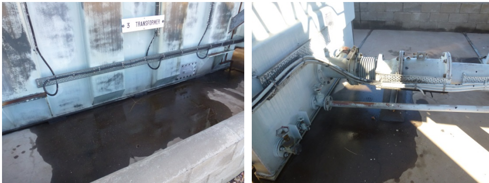
Figure 7: Oil leaks resulting in free oil collecting on the concrete around the main tank on the LV side as well as at the tertiary bushings end.
