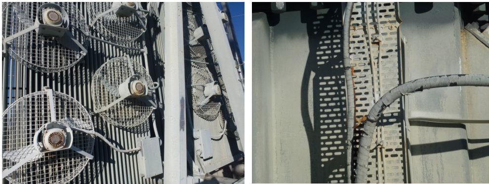
Figure 32: (LH) Corrosion of the fan motor housings. (RH) Corrosion on cable trays.
