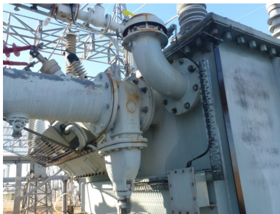
Figure 17: Corrosion around the flanges, valve body and PRD.
