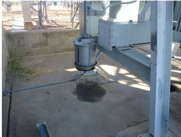
Figure 25: There were minimal oil leaks on the cooler bank with only two notable traces of oil on the concrete, one being due to maintenance of the breather..
