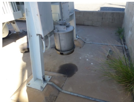
Figure 6: Cooler bank 'A' Frame structure using only two bolts per foot pad.
