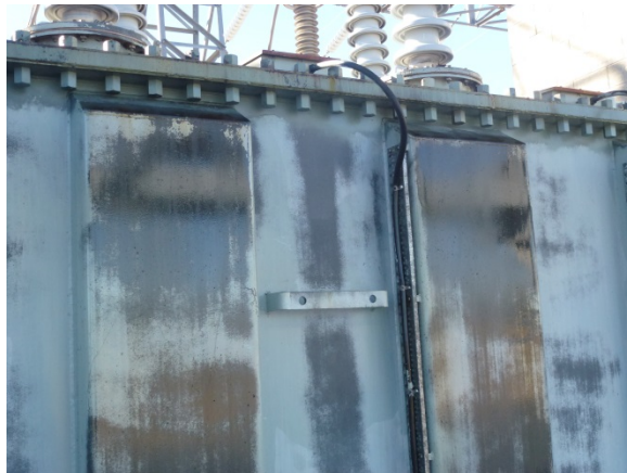
Figure 2: Transformer T3 LV side of the main tank showing the oxidised repainted surfaces.
