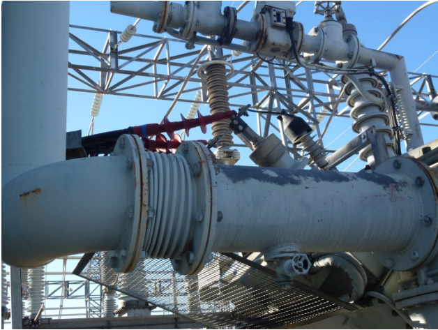
Figure 20: Small localised corrosion on main oil pipe & fittings.
