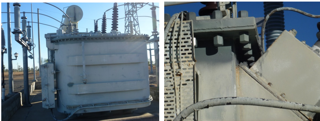
Figure 30: (LH) Tap changer end showing oxidised paint. (RH) Surface corrosion of weld on TV tank extension. Note also the cold galvanising on the welded lid strap.
