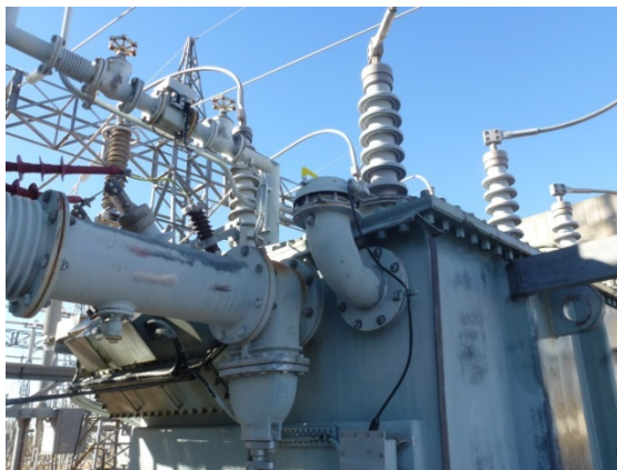
Figure 5: Corrosion between the mating flanges of the top main oil pipe between the main tank and the cooler bank.
