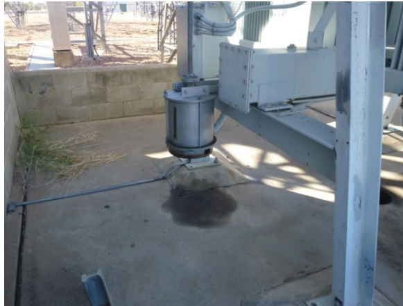
Figure 22: Cooler bank 'A' Frame structure using only two bolts per foot pad.
