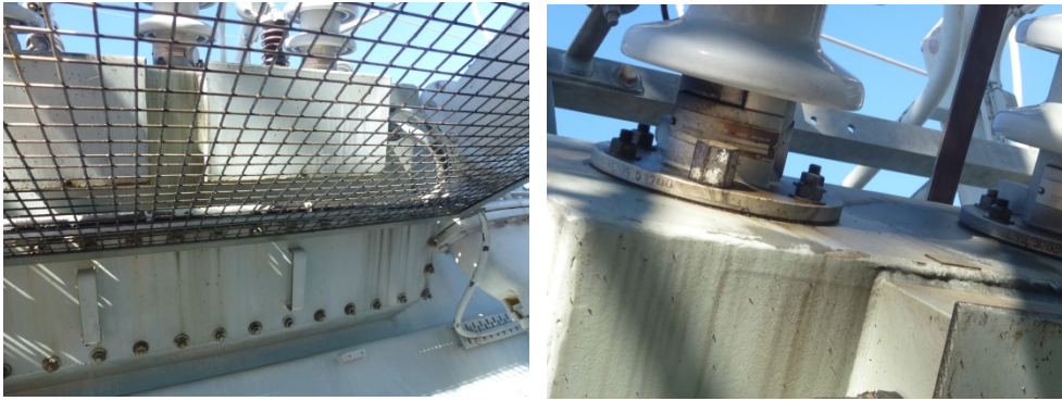
Figure 9: Oil leaks at tertiary bushings resulting in free oil running down the end of the main tank surface and collecting on the concrete below.
