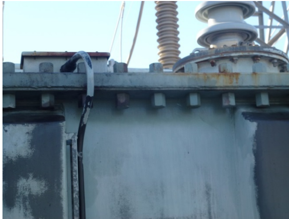
Figure 16: Typical type of minor corrosion visible on the transformer.
