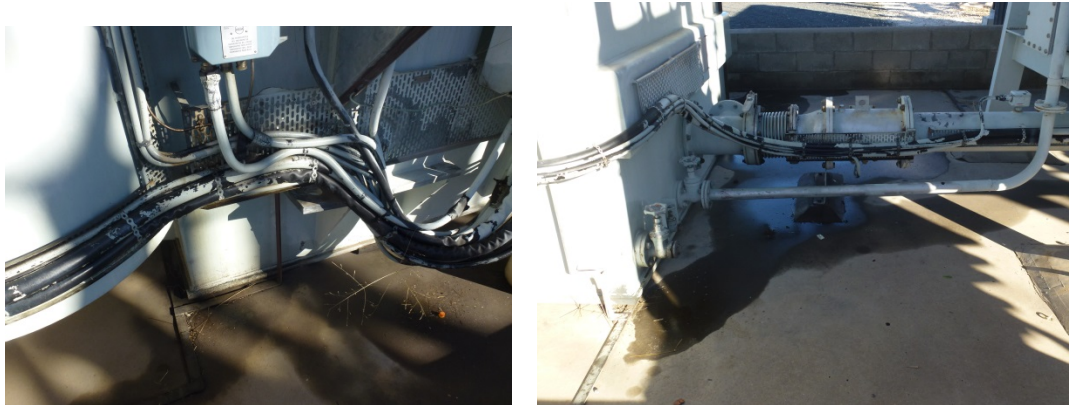
Figure 24: (LH) Oil running down the side of the main tank. (RH) Oil was also leaking from seals around the bottom main tank isolating valve.
