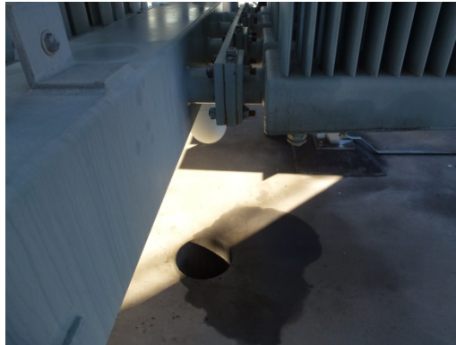
Figure 10: Cooler bank oil leaks around some radiator panel mounting flanges / butterfly valves.
