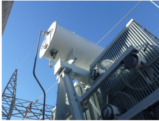
Figure 13: Main tank conservator original upper and lower mounting flanges for a Drycol refrigeration breather unit.
