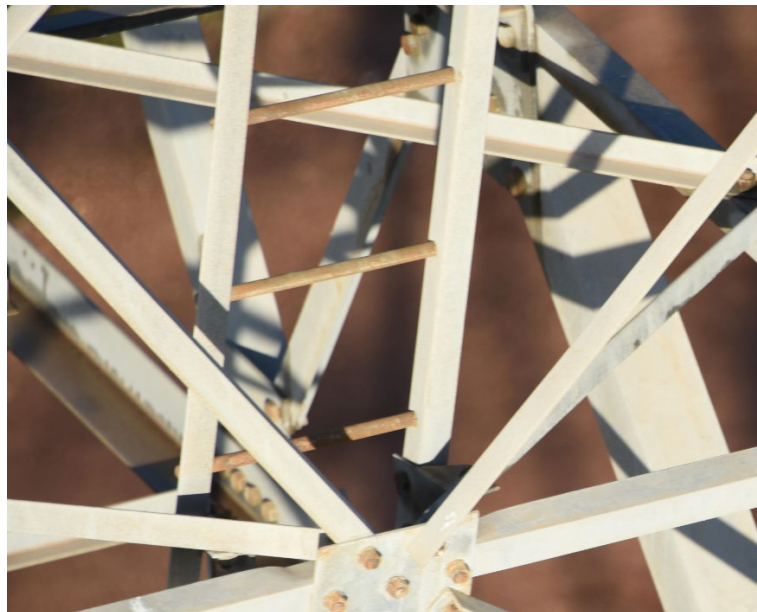
Figure 5: G2 & G3 Corrosion on ladder 1515-STR-0012
