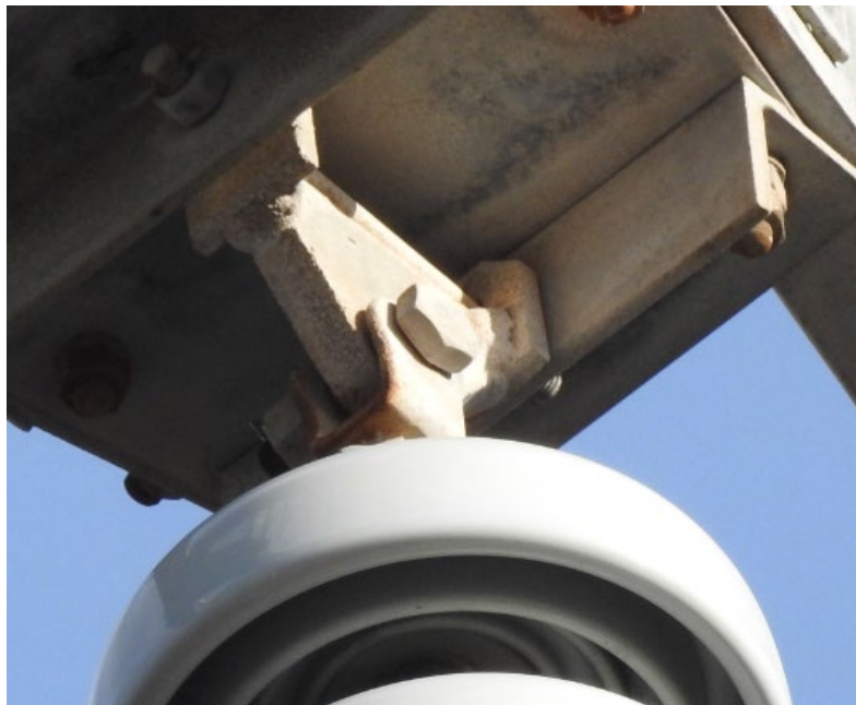
Figure 23: 1515-STR-0015 – Suspension Hardware Cold End
