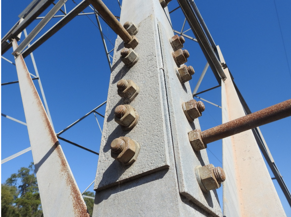
Figure 7: 1515-STR-0013 Tower Base Corrosion
