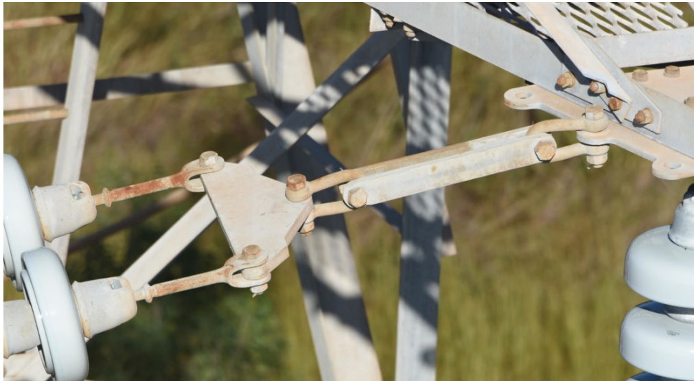
Figure 26: 1515-STR-0017 Tension Insulator Hardware – Cold End
