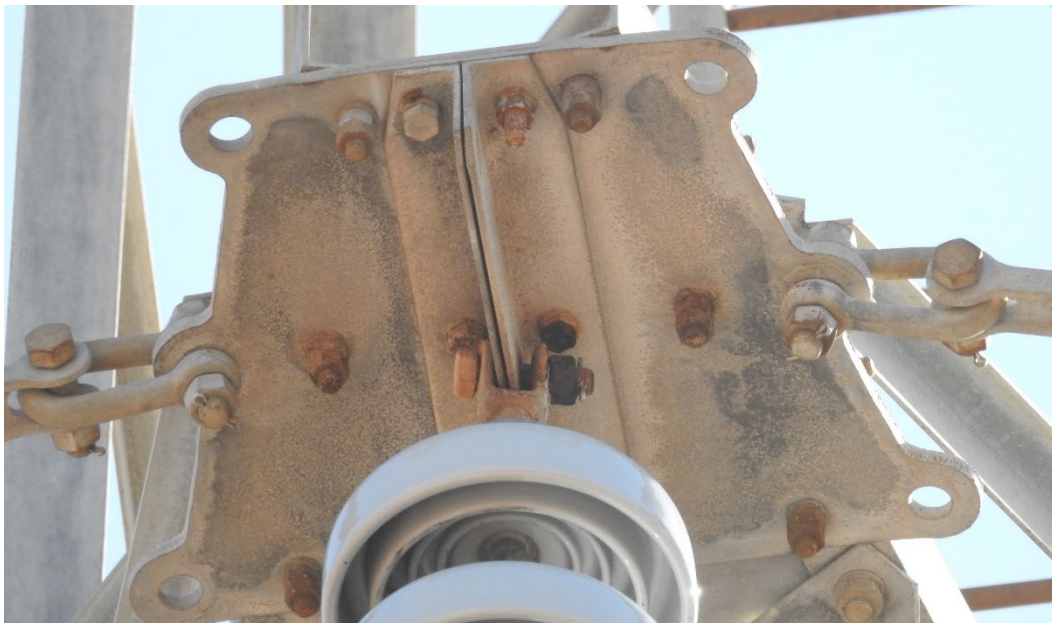
Figure 12: 1515-STR-0012 Attachment Plate bolt corrosion
