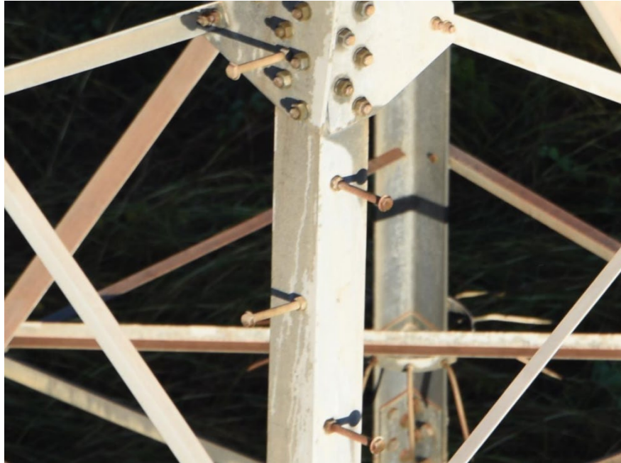
Figure 4: G2 & G3 corrosion shown on step bolts 1515-STR-0012
