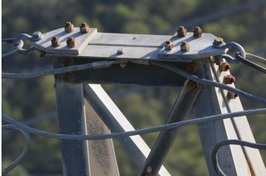
Figure 15: 1515-STR-0028 G2/G3 corroded bolts and member on earth wire peak
