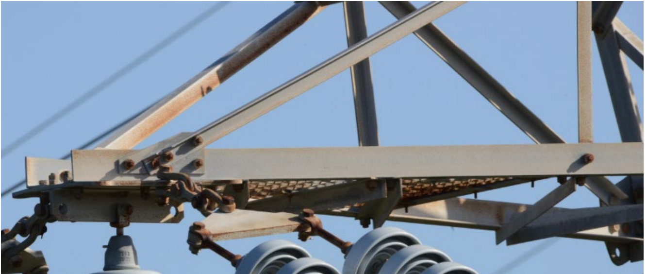
Figure 13: 1515-STR-0028 cross arm corrosion
