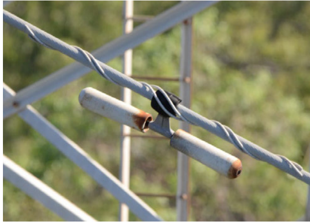
Figure 19: 1515-STR-0028 Damper showing signs of aging and corrosion
