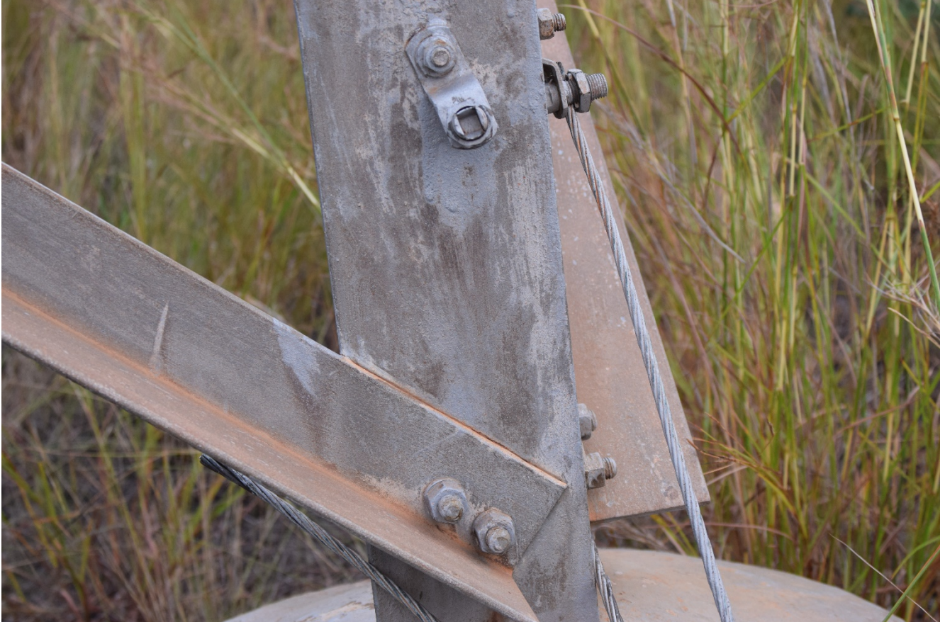
Figure 17: 1515-STR-0019 Earth strap not connected
