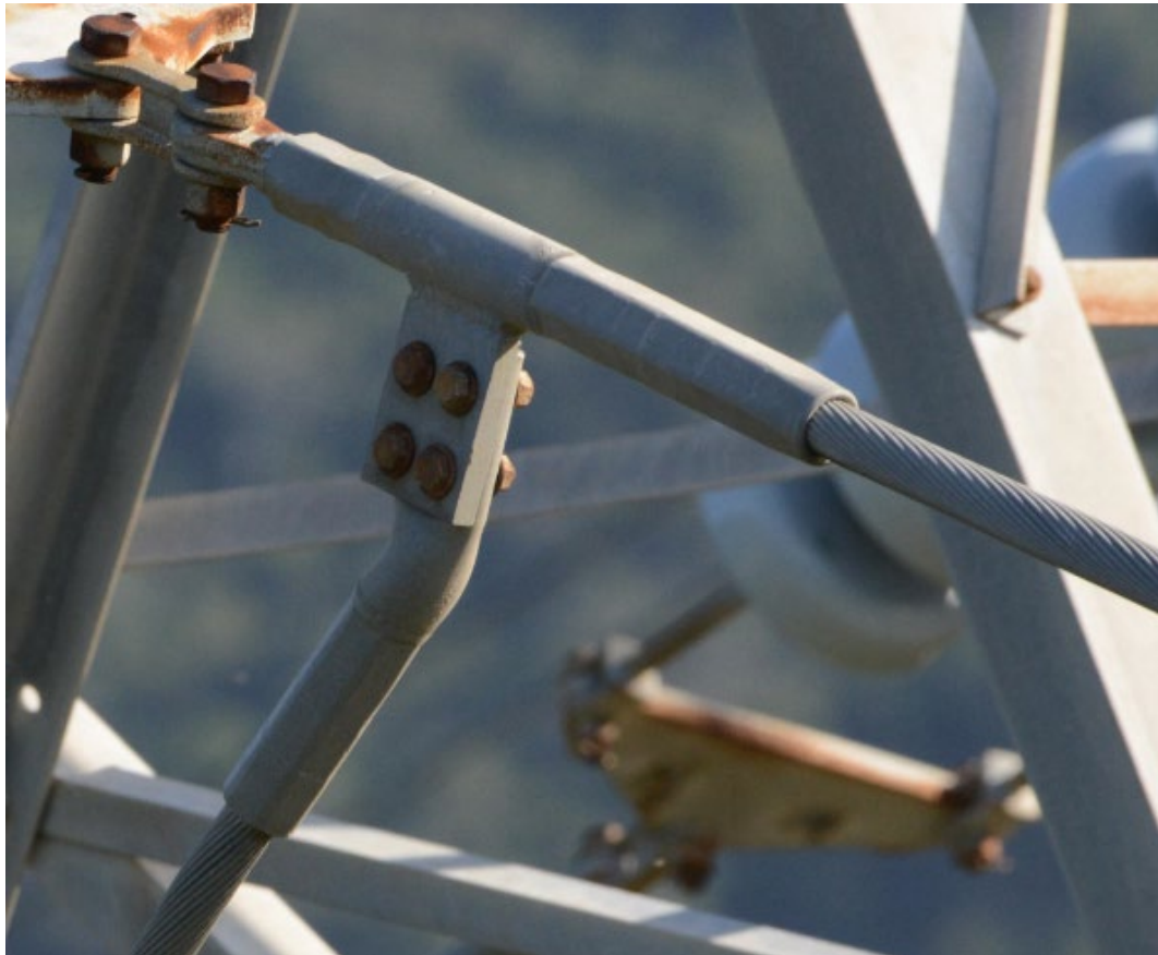
Figure 18: 1515-STR-0028 Compression Fitting Corrosion
