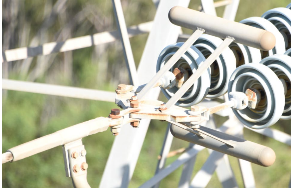
Figure 27: 1515-STR-0017 Tension Insulator Hardware – Hot End
