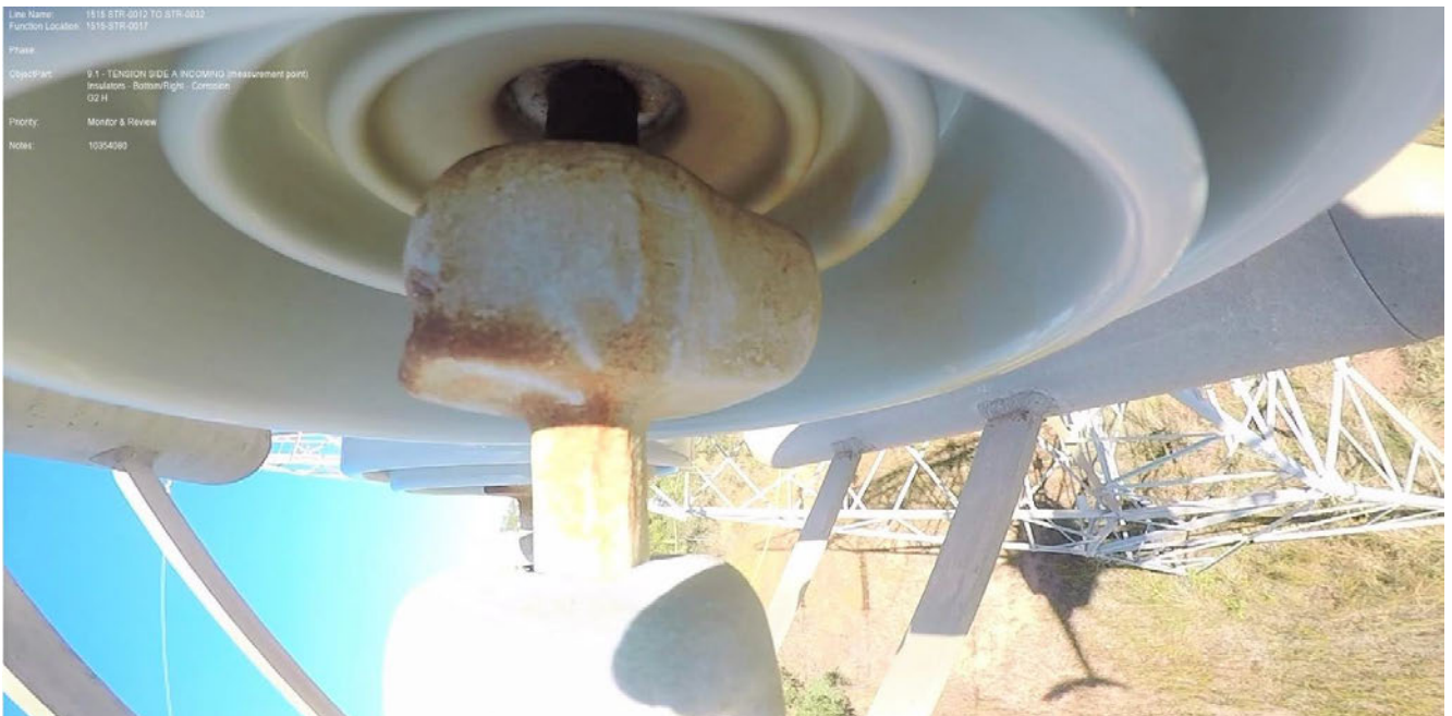
Figure 25: 1515-STR-0017 Tension Insulator G3L
