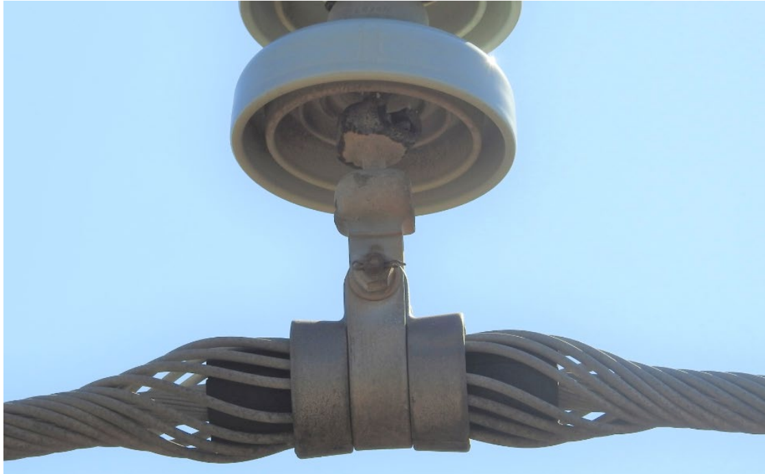
Figure 22: 1515-STR-0013 – Suspension Hardware Hot End
