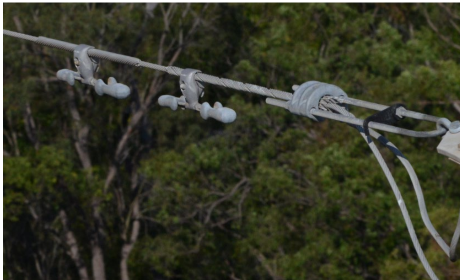
Figure 20: 1515-STR-0021 OHEW & OHEW Hardware
