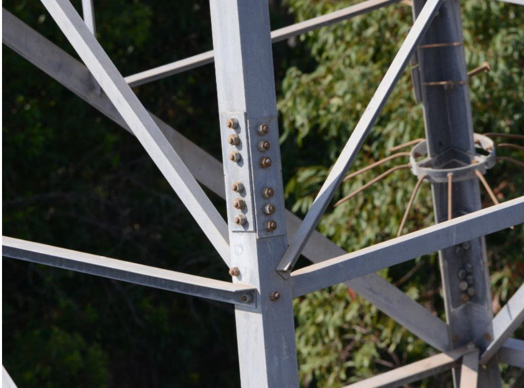
Figure 8: 1515-STR-0021 Tower Body corrosion
