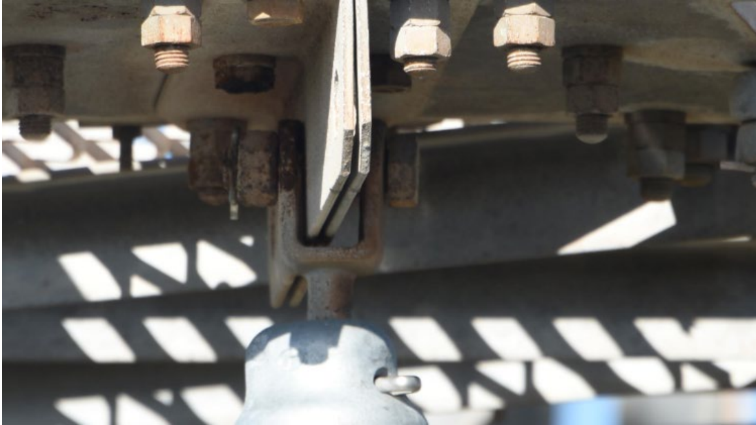
Figure 29: 1515-STR-0017 Bridging Insulator Hardware - Cold End
