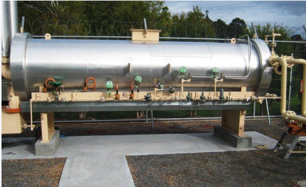
Figure 3-1: Typical water bath heater
