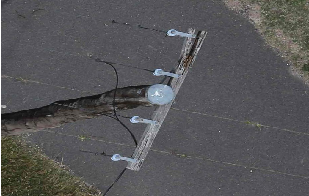
Figure 4.10 Low Voltage pole off Cotter 11kV feeder (March 2014)
