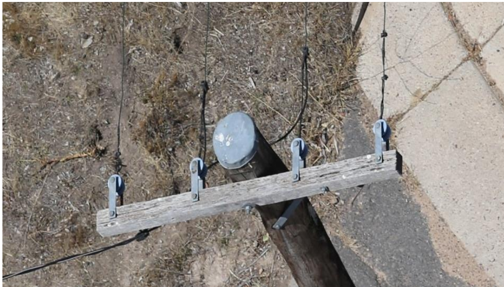
Figure 4.9 Low Voltage pole off Cotter 11kV feeder (June 2013)
