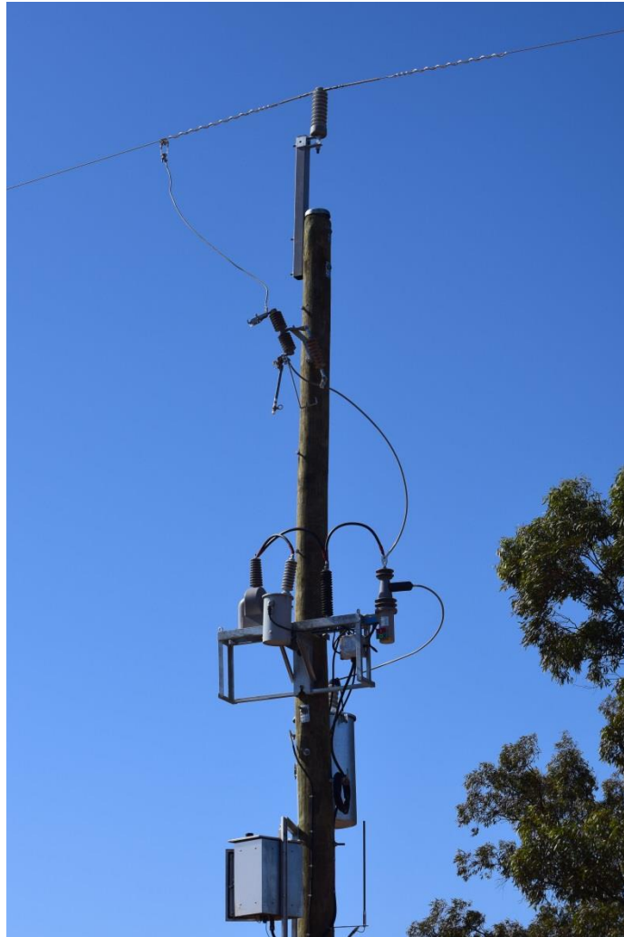
Figure 15: Nyngan SWER Switched Reactor
