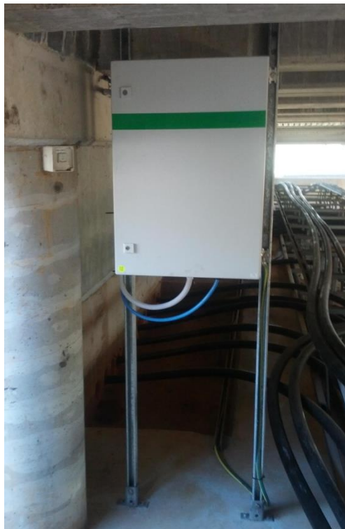
Figure 9 - Clearwater Zone Substation 5kVA four quadrant inverter (atypical) installation
