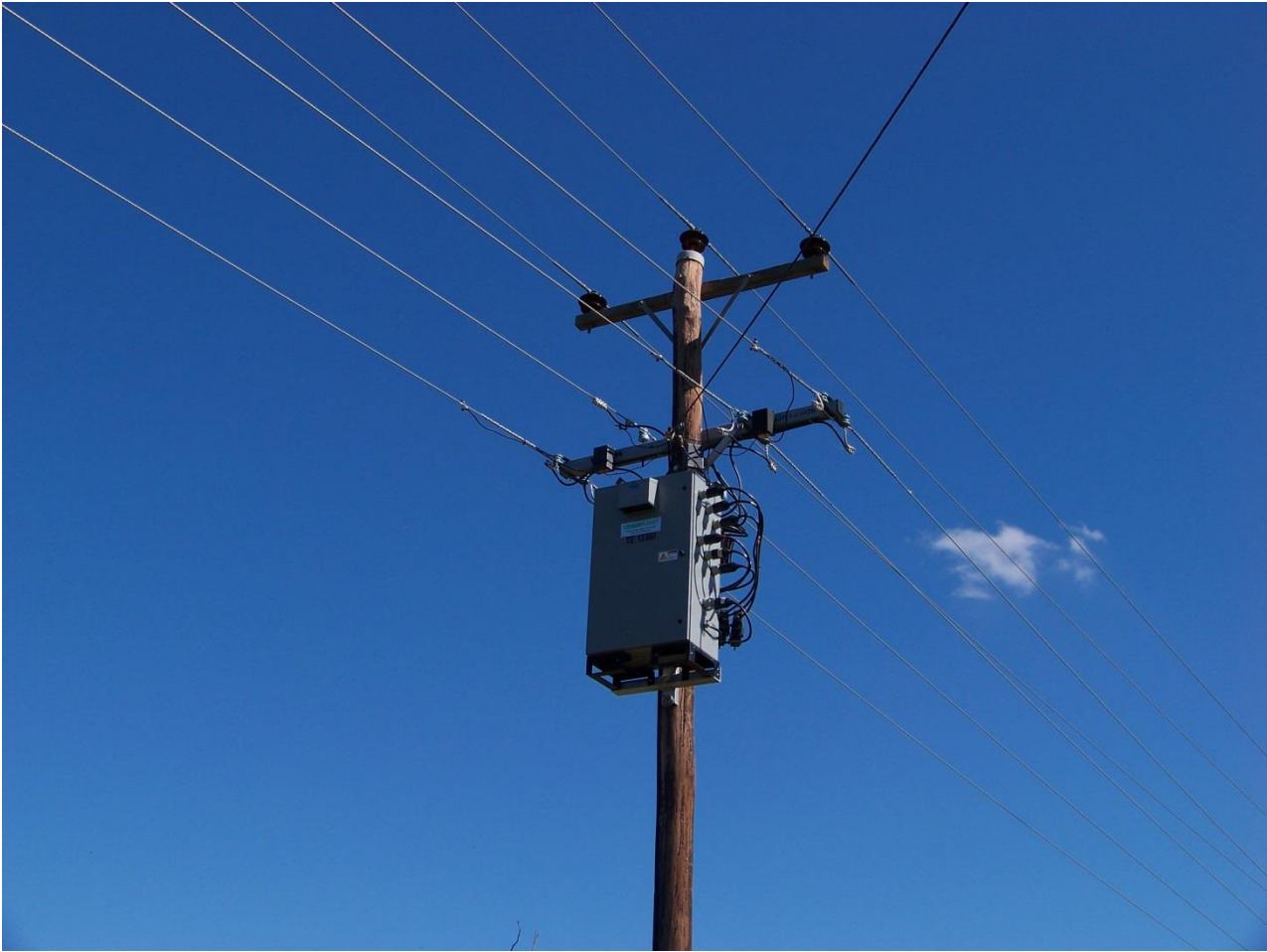
Figure 11 - Low Voltage Regulator
