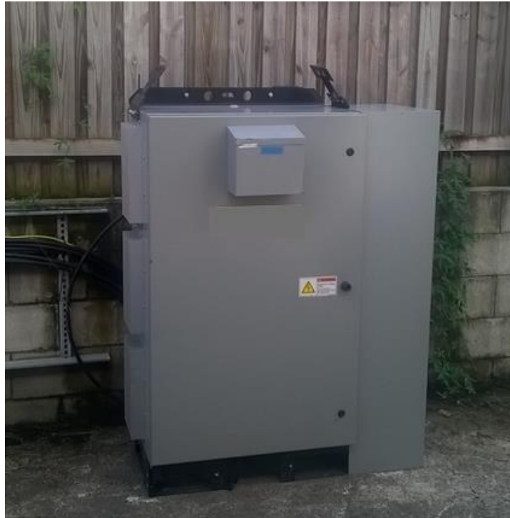
Figure 13: 3 phase LV regulator connected to a commercial load
