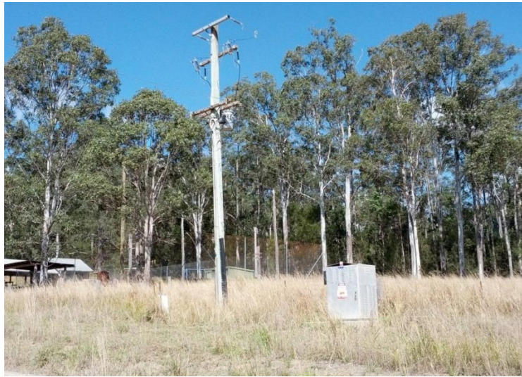
Figure 6 Pappinbarra Inverter Installation
