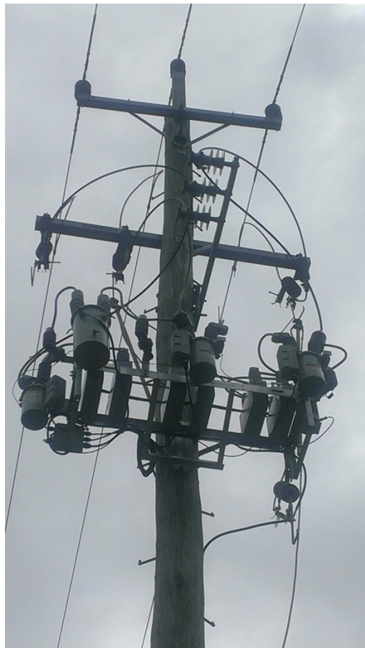
Figure 3 - Clarendtown trial capacitor bank installation
