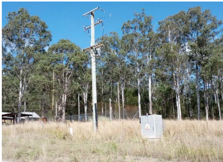
Figure 3 Pappinbarra Inverter Installation
