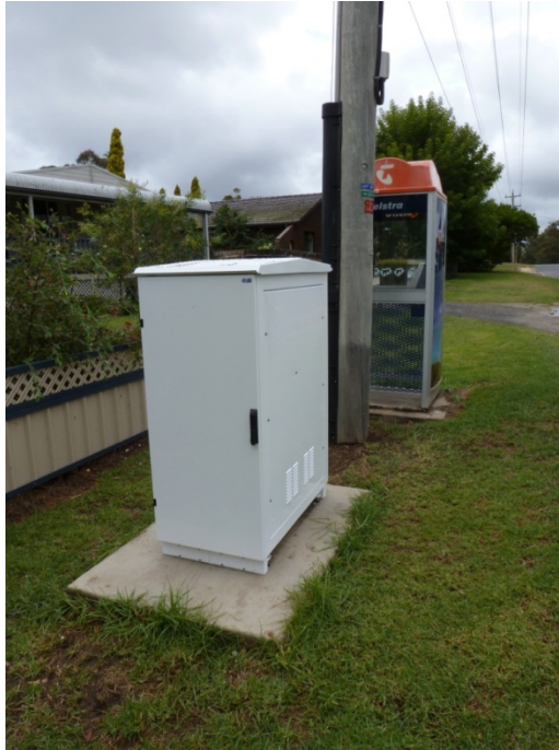
Figure 2 Bega / Kalaru Inverter Installation
