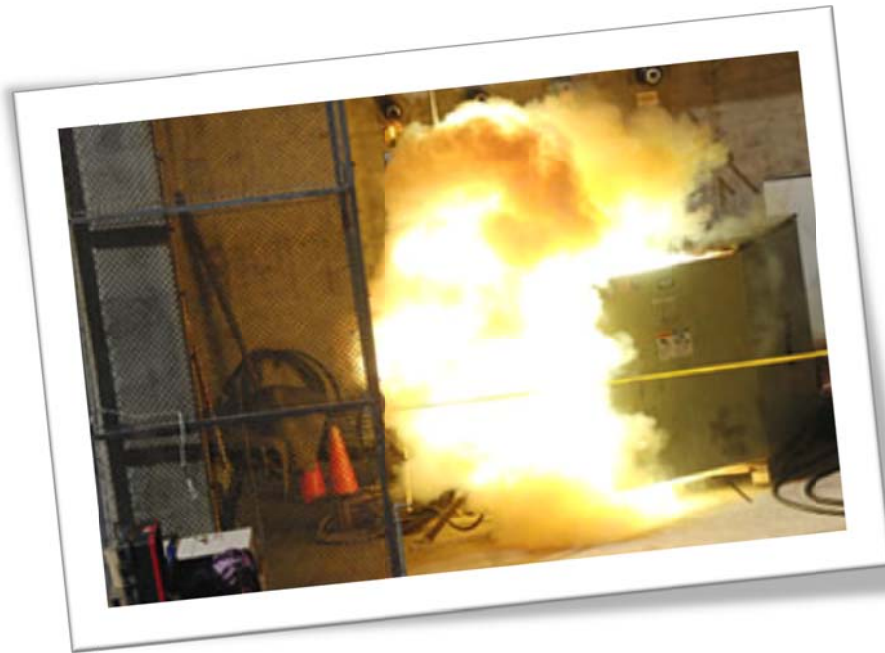
An arc flash explosion from a 21kV padmount switch [1]
