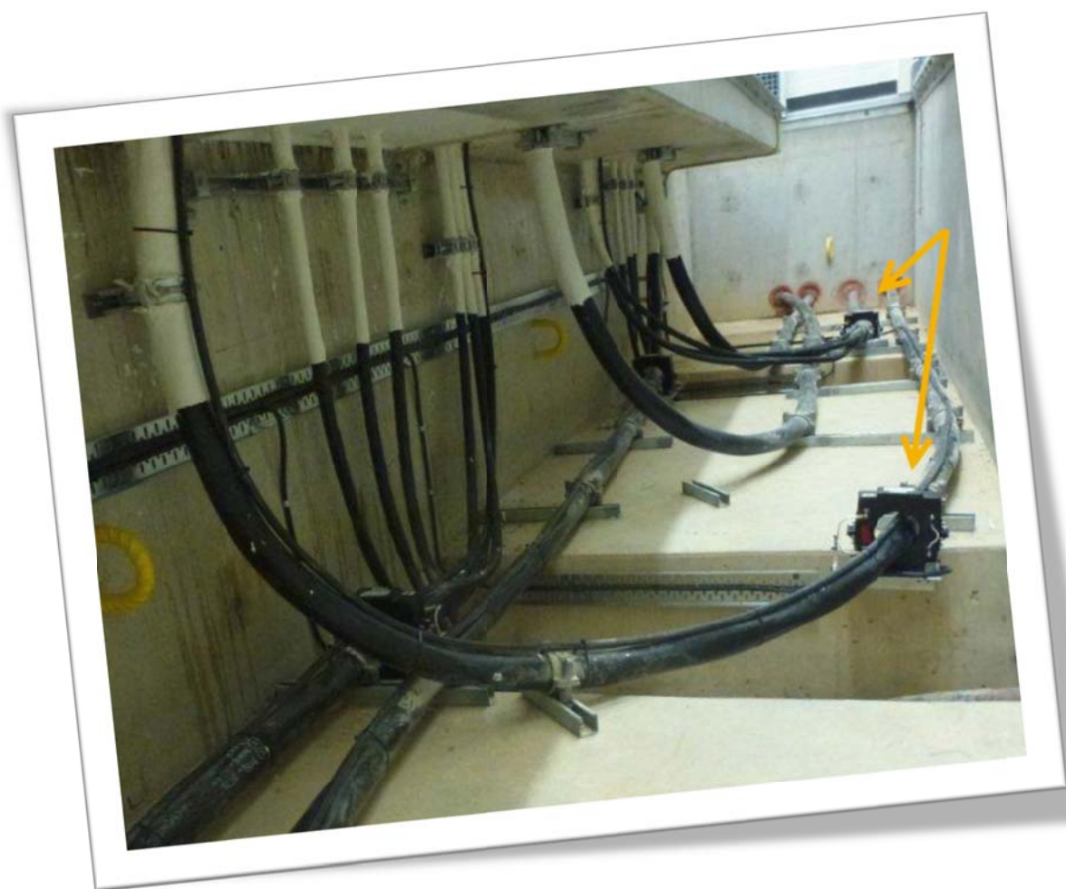
Core balance CT's installed at Blackheath Zone Substation
