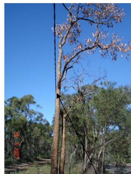
Tree in physical contact with LVABC shall be removed
