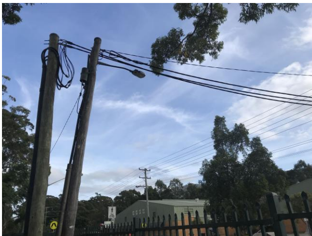
Figure 2 – Bray Street Coffs Harbour – New road crossing pole inserted behind existing road crossing pole
