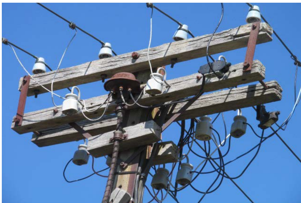
Figure 3 Typical cast iron LV pothead
