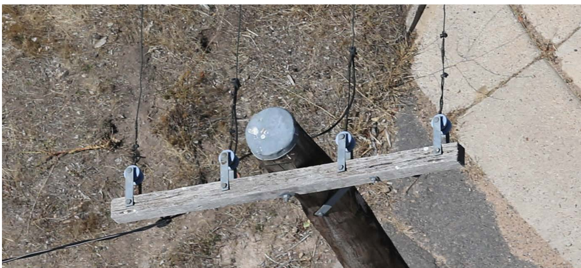
Figure 1 March 2014 – Low voltage pole off Cotter 11 kV feeder
